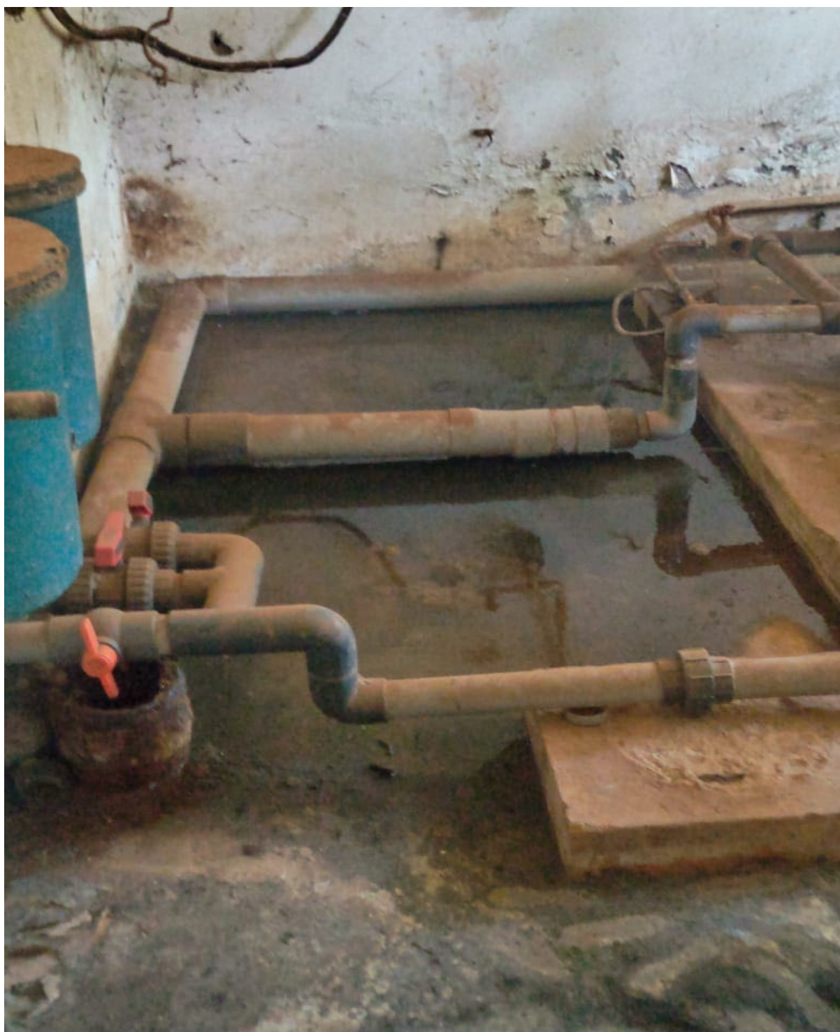
Figure 3: Water spread across the floor of a stance in the toilet
