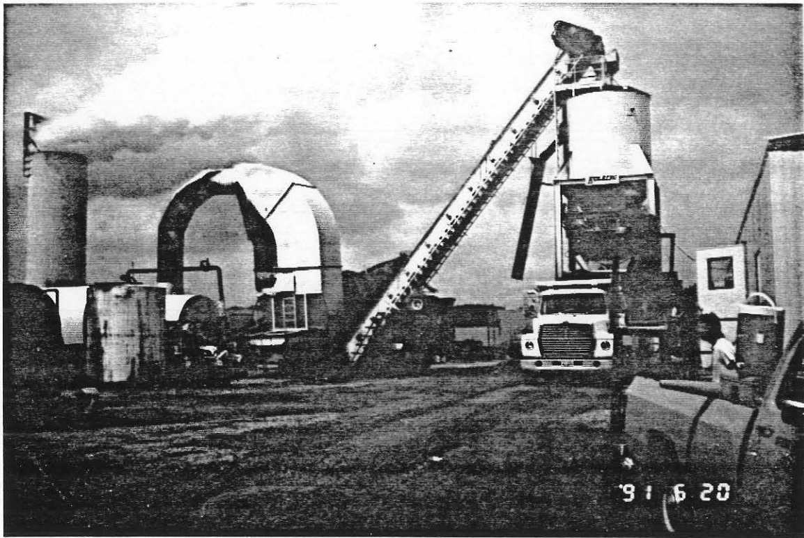
Figure 4. Bituminous Mixture Production Plant
