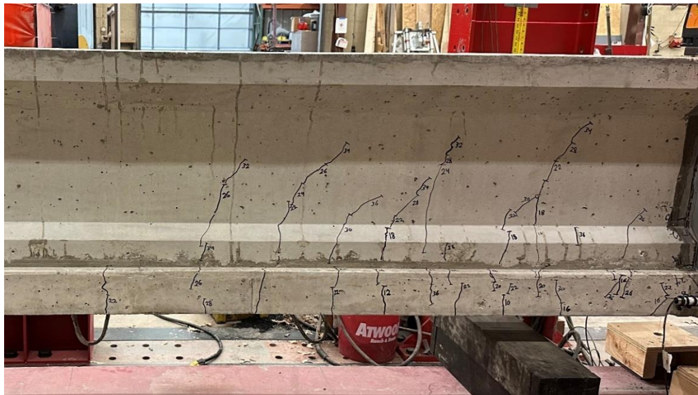
Figure 83: East side of south girder SSDU-1 showing flexural cracks after negative moment test
