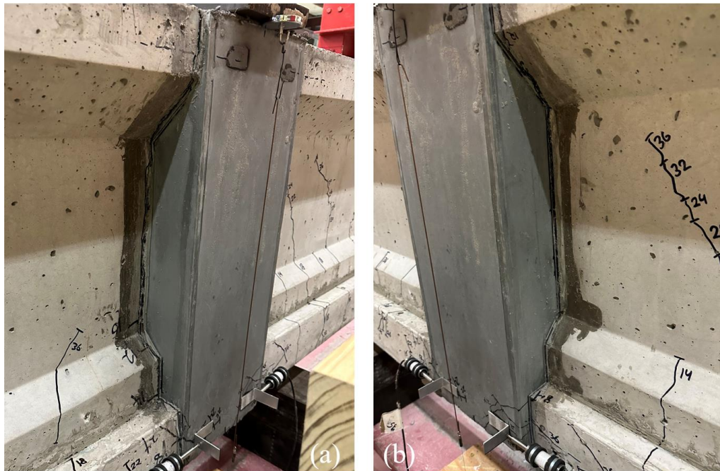
Figure 88: Southeast (a) and northeast (b) side of joint SSDU-1 showing cracking along the interfaces under final negative moment test loading
