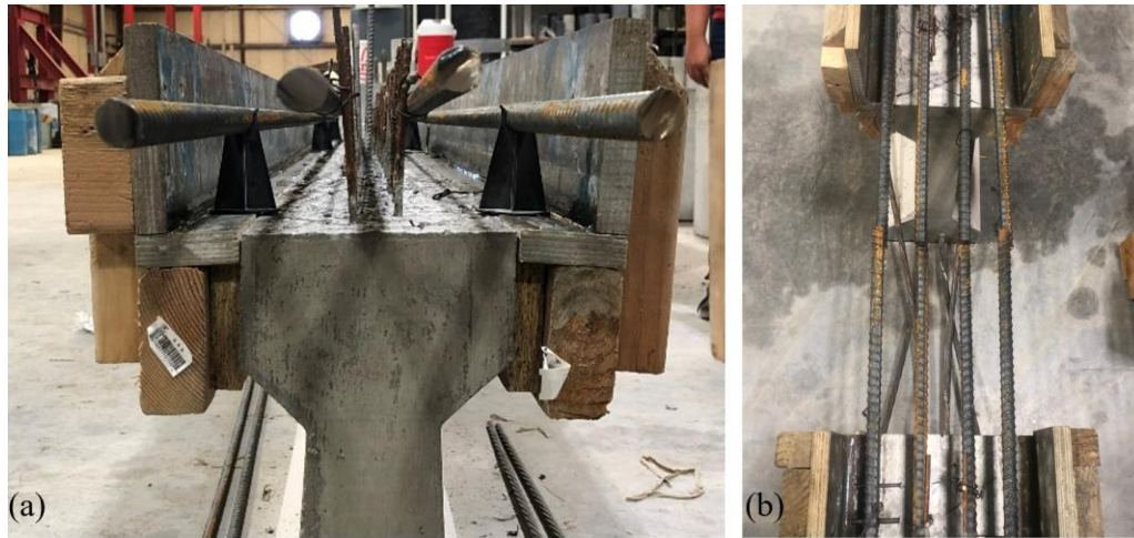
Figure 13: Deck reinforcement vertical offset (a) and adjacent lap splice alignment (b)
