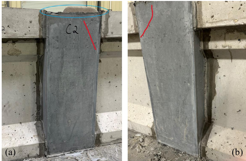
Figure 44: Preexisting settlement is indicated by a blue oval and preexisting cracking is indicated by a red line on the southeast (a) and northeast (b) side of the joint HSJ3-2 before testing.
