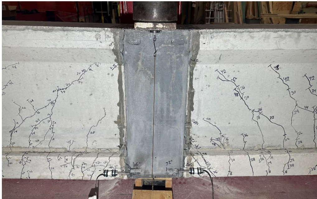
Figure 39: Flexural cracking at east side of the joint for HSJ3-2 under final loading
