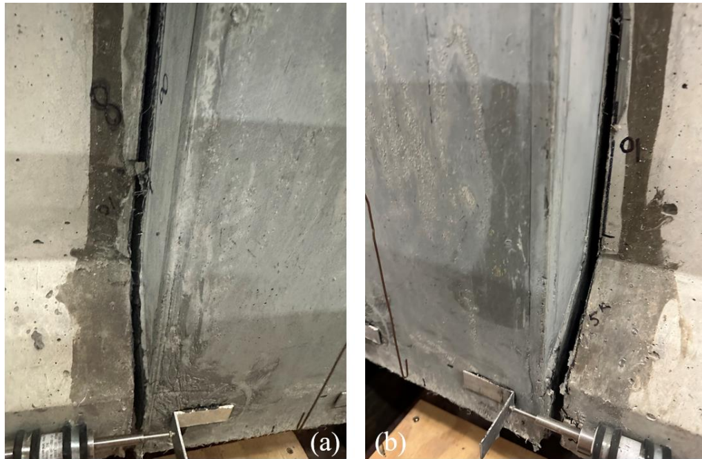
Figure 107: Northwest (a) and southwest (b) side of joint SSDU-2 showing cracking along the as-cast bottom of the interfaces after final positive moment test loading
