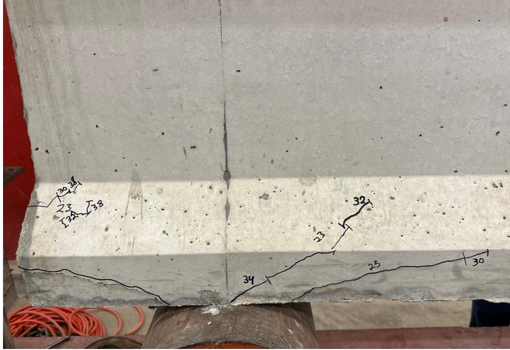
Figure 59: Cracking on the northwest side of HSDU-2 in the girder directly above the north roller support
