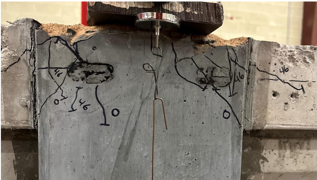
Figure 100: West side of joint SSDU-2 in positive moment orientation showing undocumented cracks near the as-cast top surface caused by negative moment testing Note: All cracks unlabeled or labeled 46 kips resulted from final loading of approximately 41.6 kips
