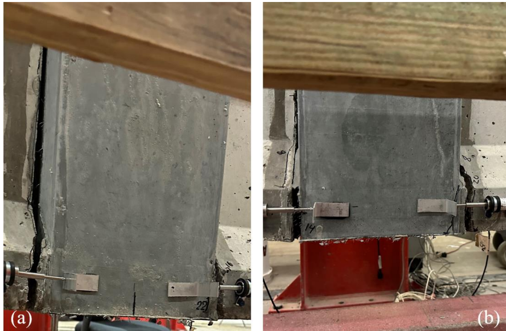
Figure 57: Separation at the interface of HSDU-2 from the east (a) and west (b) side under final positive moment test loading
