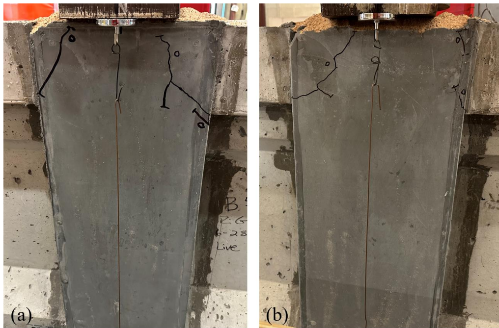
Figure 71: East (a) and west (b) side of joint SSDU-1 showing preexisting cracks before positive moment testing
