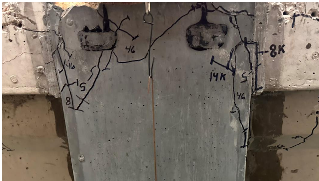
Figure 105: East side of joint SSDU-2 showing cracks near the as-cast top face after final positive moment test loading
