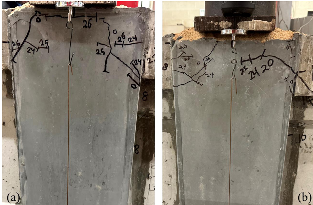
Figure 76: East (a) and west (b) side of joint SSDU-1 showing cracks near as-cast top face under final positive moment test loading
