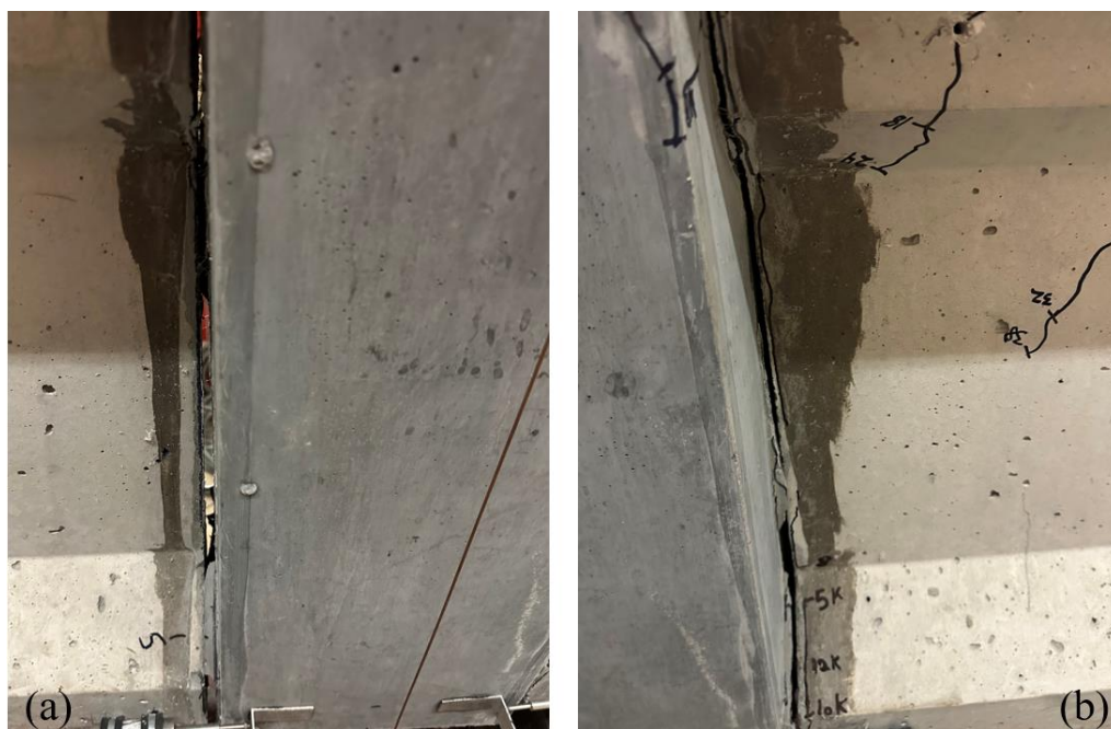
Figure 106: Southeast (a) and northeast (b) side of joint SSDU-2 showing cracking along the as-cast bottom of the interfaces after final positive moment test loading
