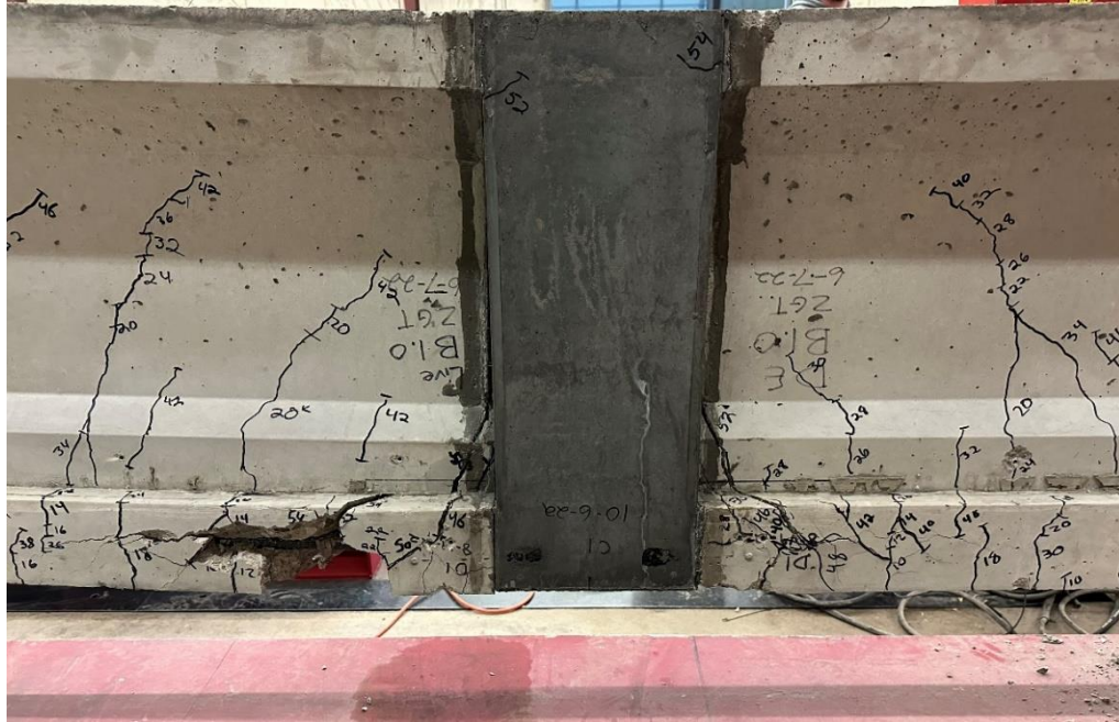
Figure 30: East side of HSJ3-1 joint after final loading showing locations of significant concrete spalling
