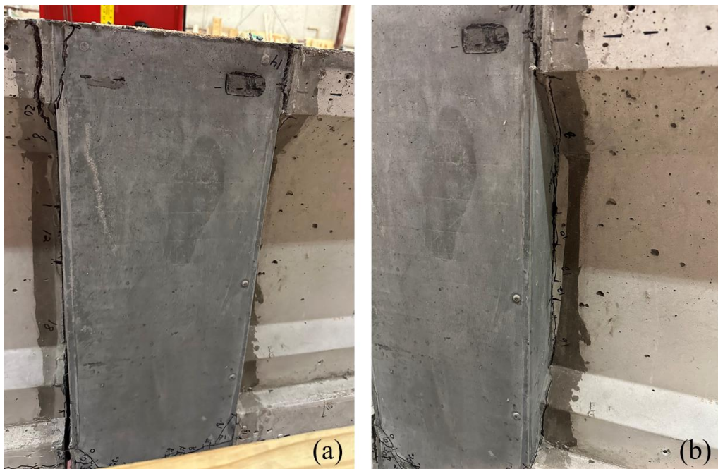
Figure 65: Southeast (a) and northeast (b) side of joint HSDU-2 showing cracks at the interface after negative moment testing
