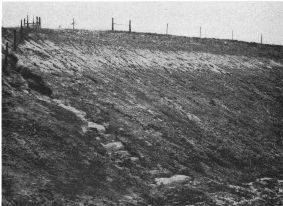
Figure 5. Soil erosion occurs as a result of improper design through omission of a physical barrier along the shoulder to concentrate and remove excess water (top photo), and because of inadequate rights-of-way interceptor ditches could not be constructed on top of cut slopes particularly for the orderly removal of excess water (bottom photo) from terrace outlets, or adjacent watershed.
