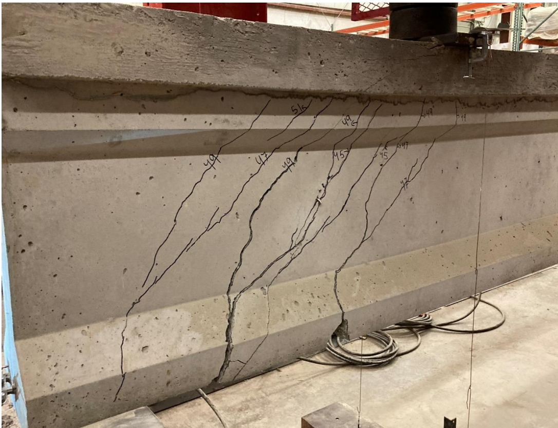
Figure 76. Girder with cracks after initial load test.
