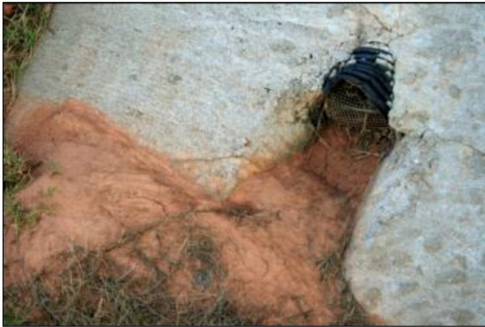
Figure 121. Soil flowing out of underdrain outlet.
