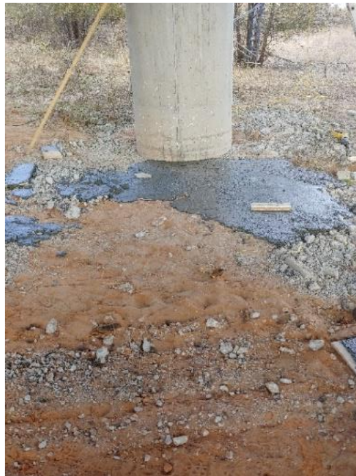
Figure 93. UHPC from failed formwork
