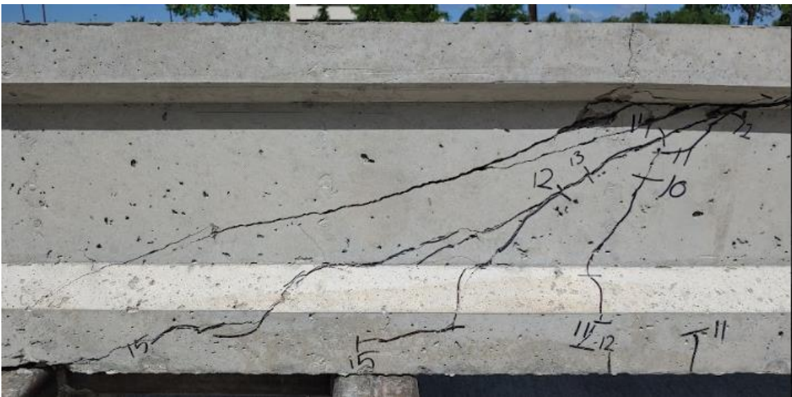
Figure A-24: Shear cracking in RC-B2 NW side after buckling
