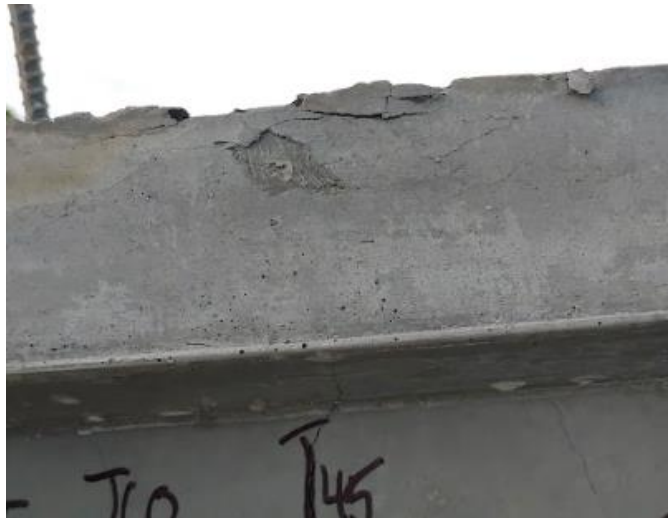
Figure A-50: Crushing of concrete in UHPC-B5 in middle section
