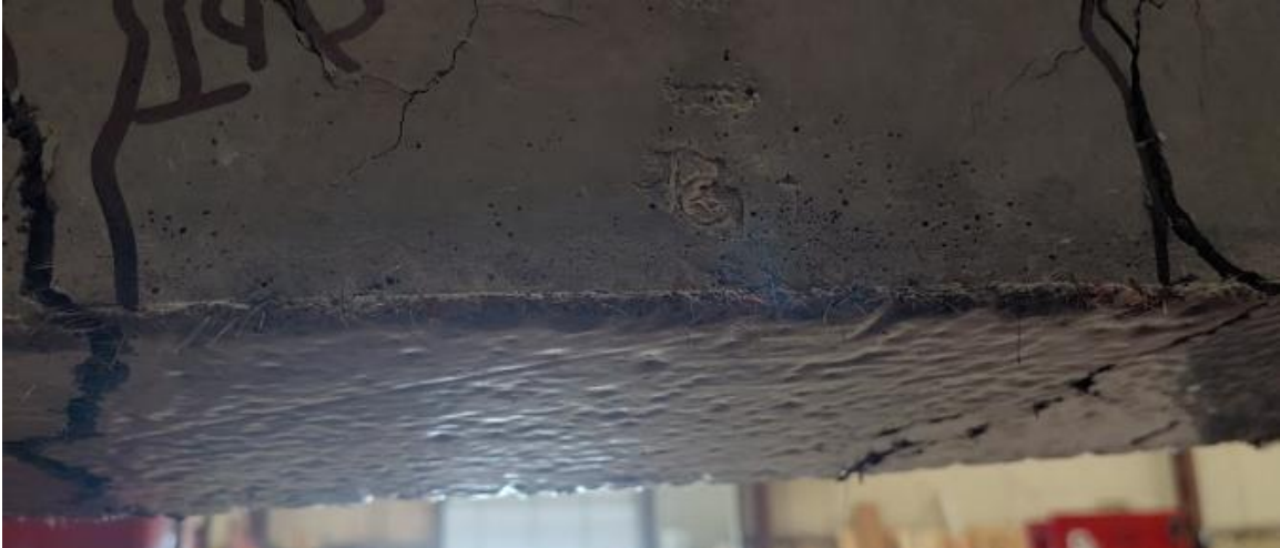
Figure A-35: Cracks across bottom of UHPC-B3
