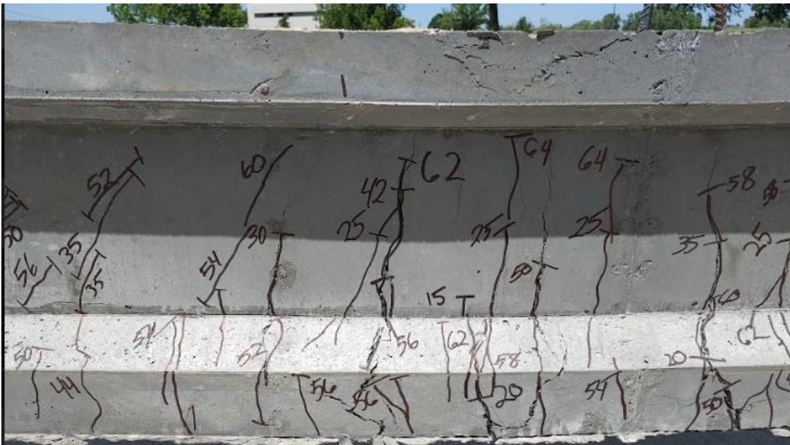
Figure A-44: Crushing of concrete between loading point in UHPC-B4 W side
