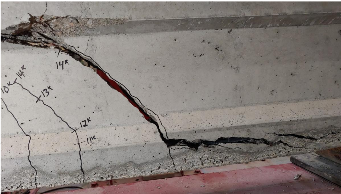
Figure A-14: Shear cracking in RC-B1 NE side after buckling
