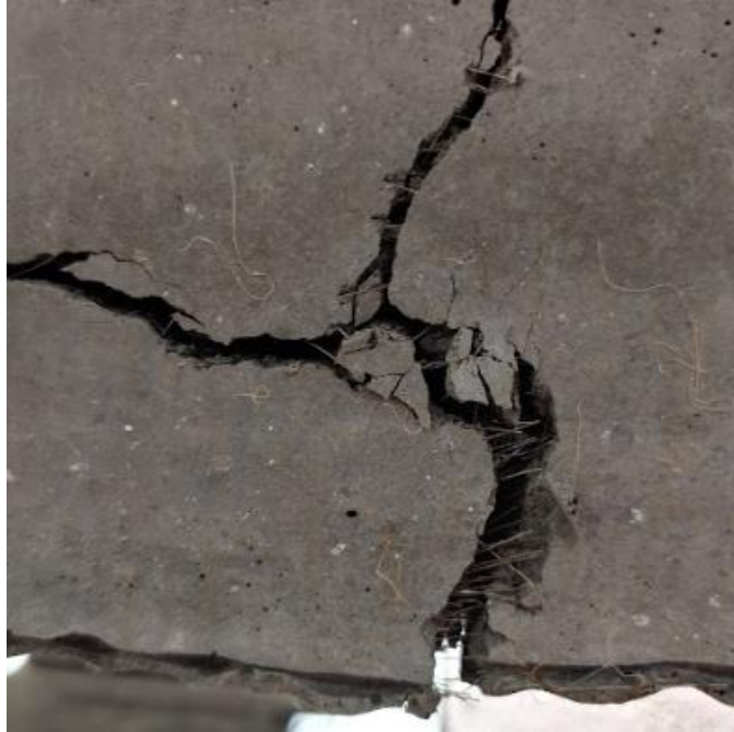
Figure A-43: Cracking in UHPC-B4 center of bottom flange W side
