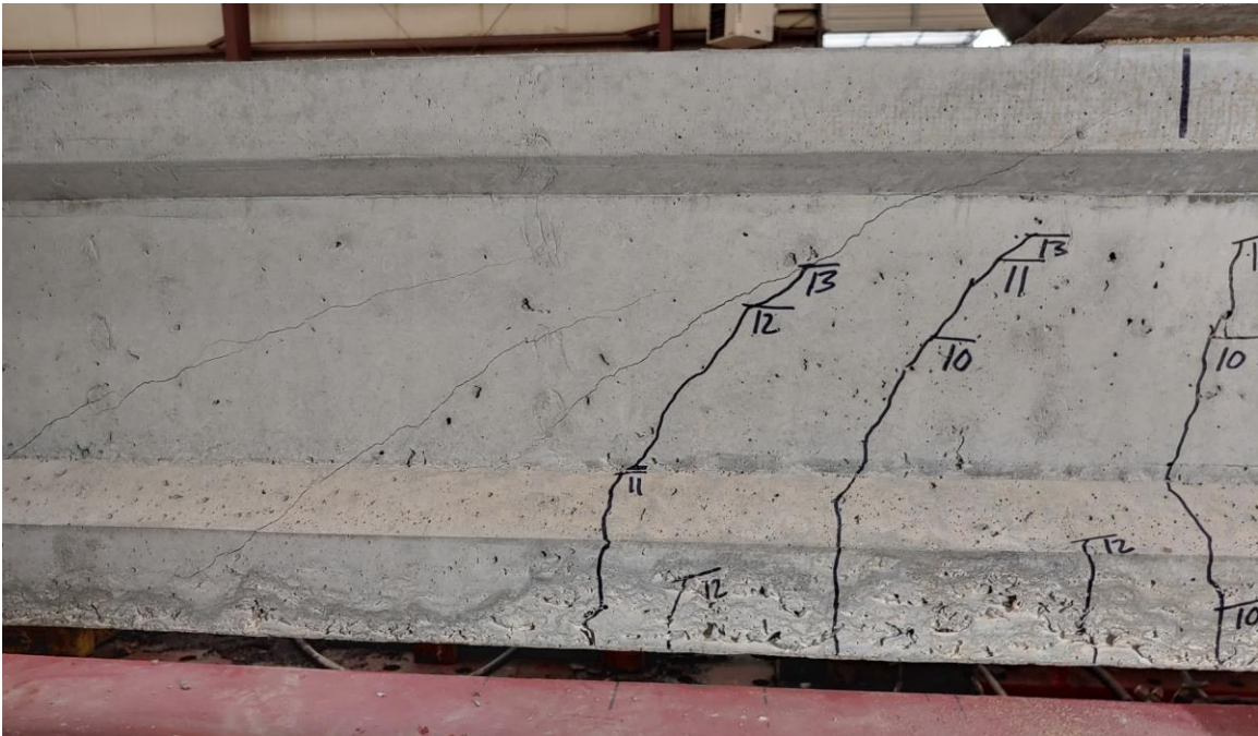
Figure A-12: Shear cracking in RC-B1 SE side
