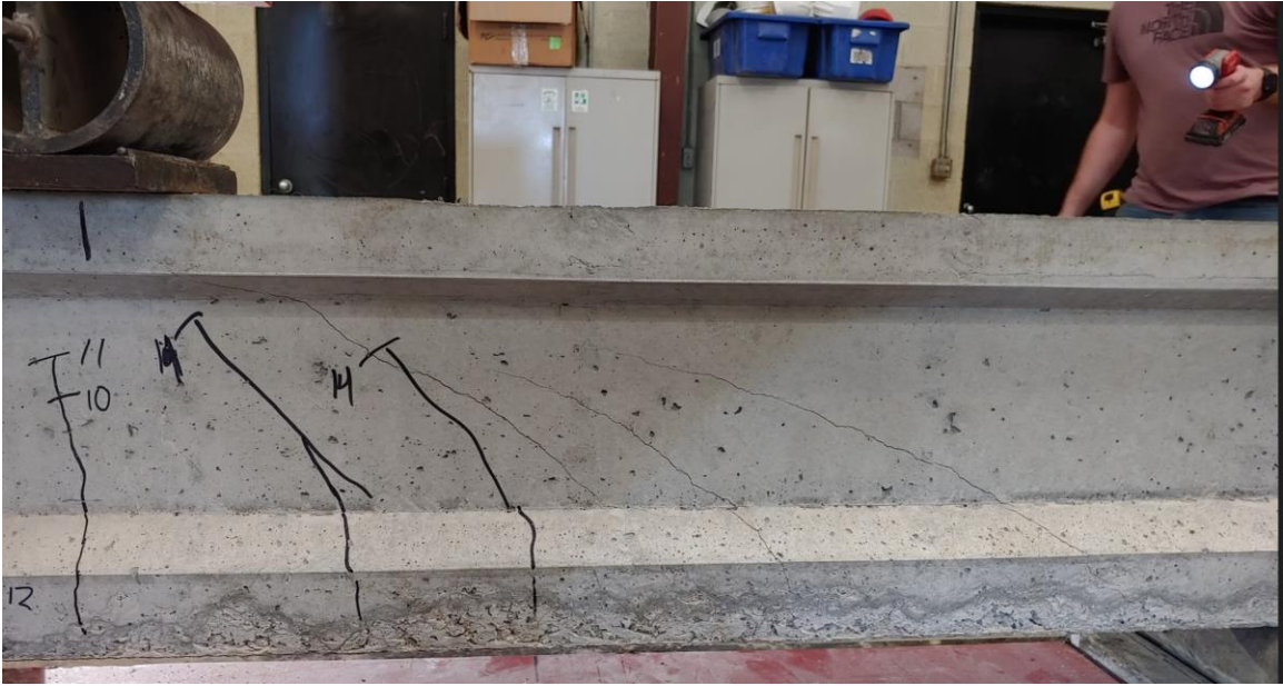
Figure A-11: Shear cracking in RC-B1 SW side
