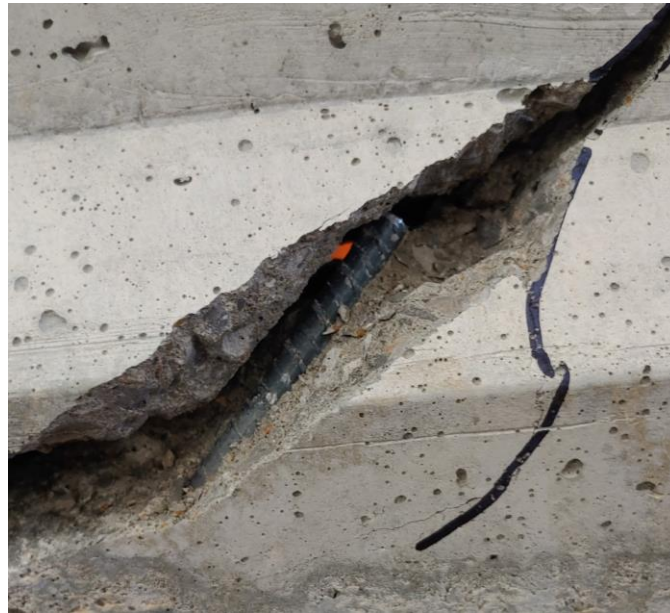
Figure A-18: Shear crack revealing crosstie
