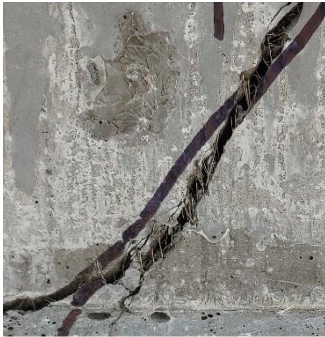
Figure A-36: Angled crack with steel fibers in UHPC-B3
