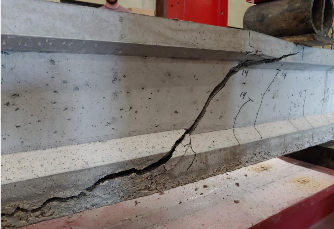
Figure A-15: Shear cracking in RC-B1 NW side after buckling
