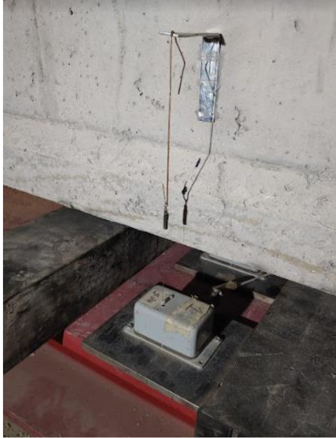
Figure A-10: Wire pot attached to beam
