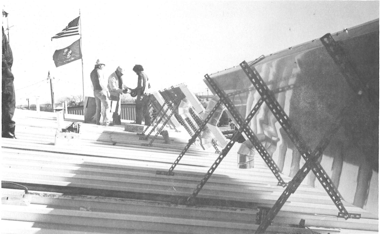
Figure B-3. Mounting brackets bolted to roof holding collectors at 45° angle.
