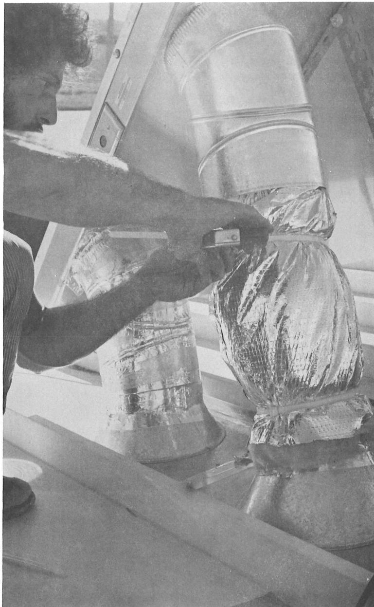
Figure B-6. Foil backed insulation put around air ducts.
