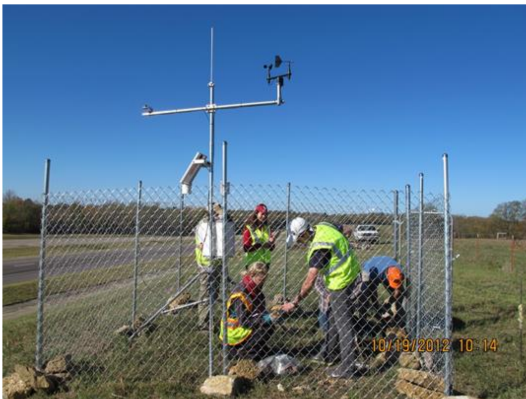
Figure 3.1. Weather station installed at Idabel test site.
