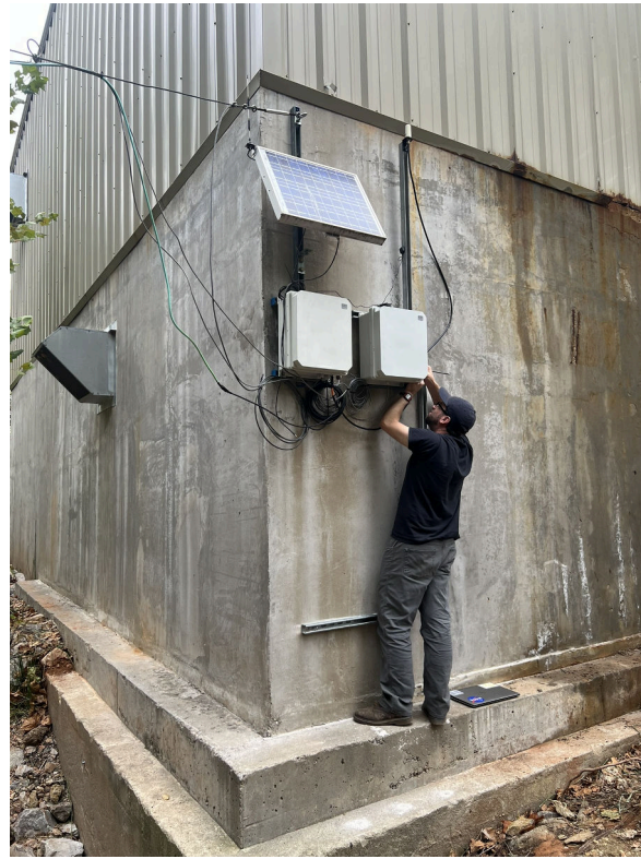
Figure 5.4: Enclosures and Solar Panel at Falls Creek near Davis, OK
