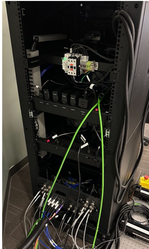
Figure 3.16: Equipment rack back view (Courtesy: eMWave-tech)
