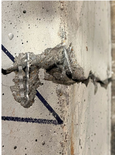
Figure 39: Fiber-Reinforcement Bridging Cracking Interface, Example 2
