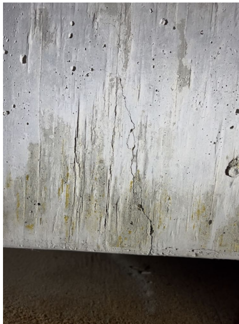
Figure 91: Cracked CSCR Specimen
