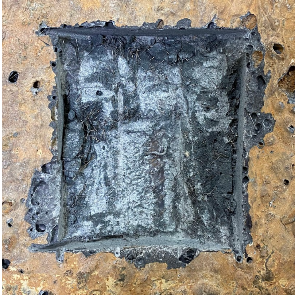
Figure 5-30: CU-L observed rebar D, 65 days tested
