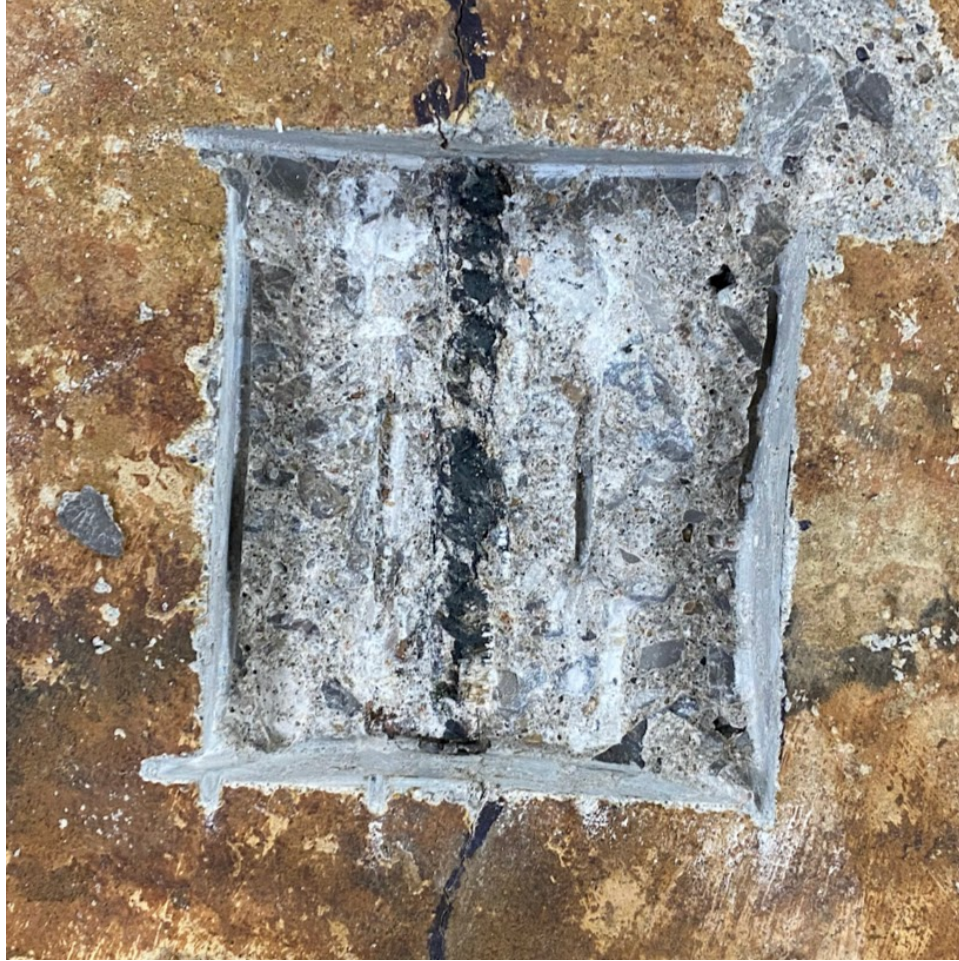
Figure 5-27: CAA-N observed rebar D, 65 days tested
