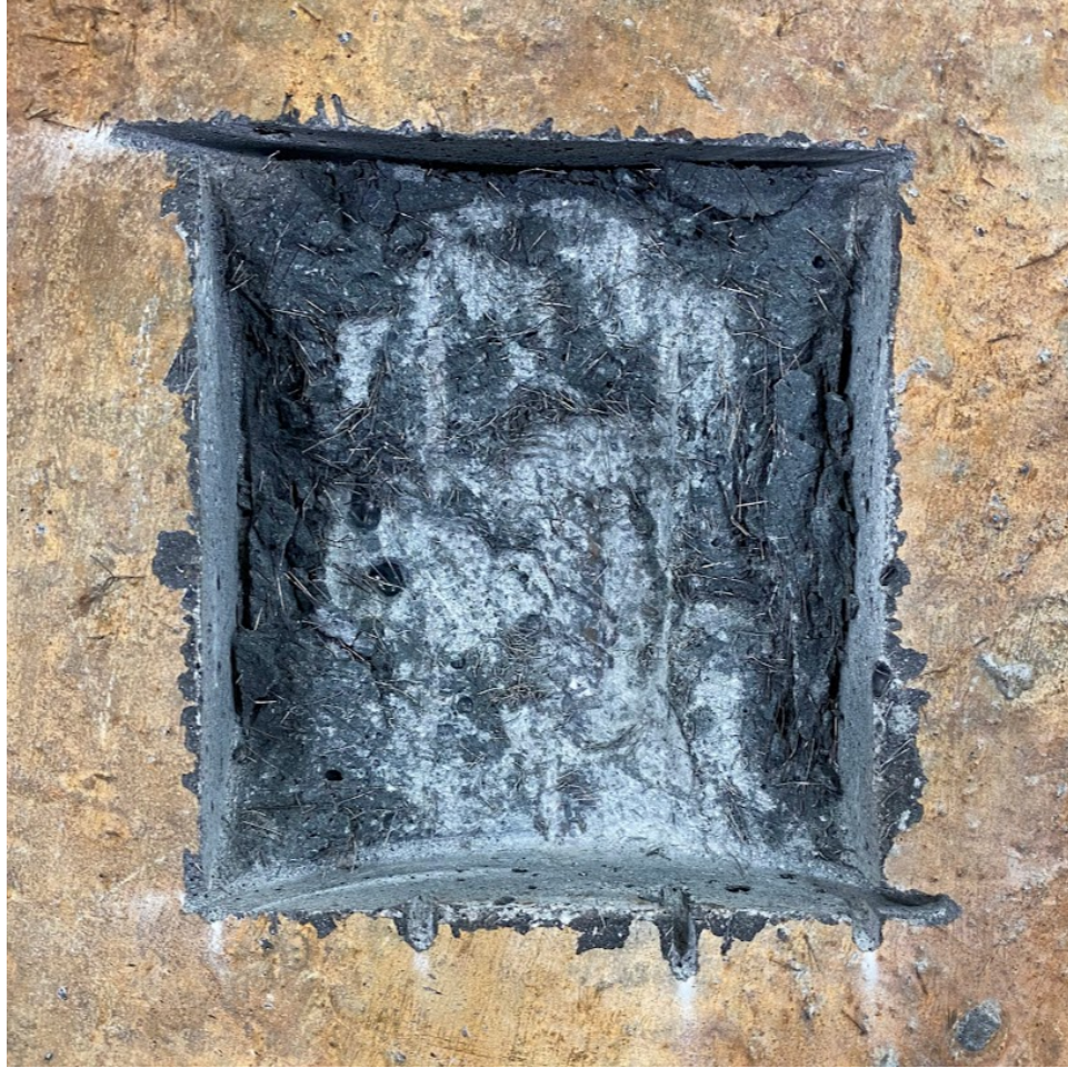
Figure 5-33: CU-N observed rebar D, 65 days tested
