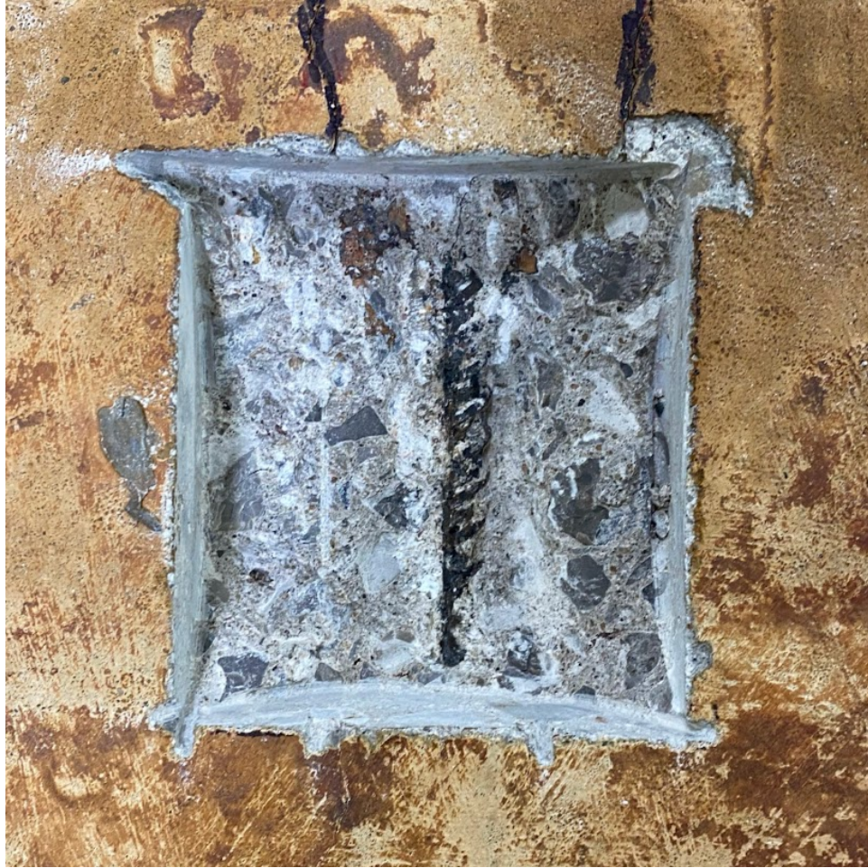
Figure 5-23: CAA-L observed rebar C, 65 days tested
