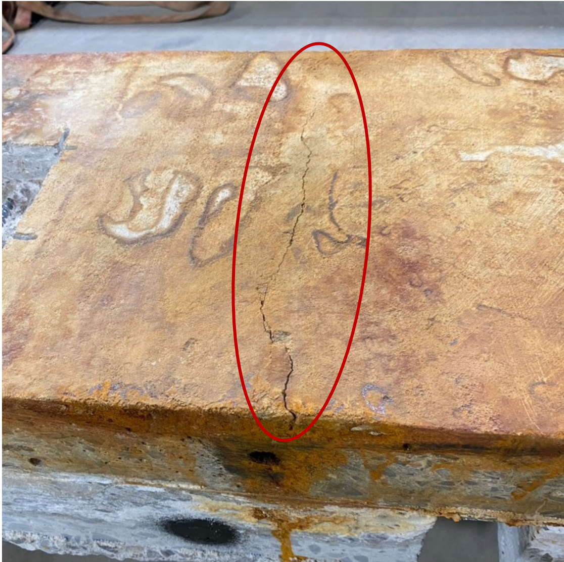
Figure 5-14: Cracking in specimen CAA-N (annotated)
