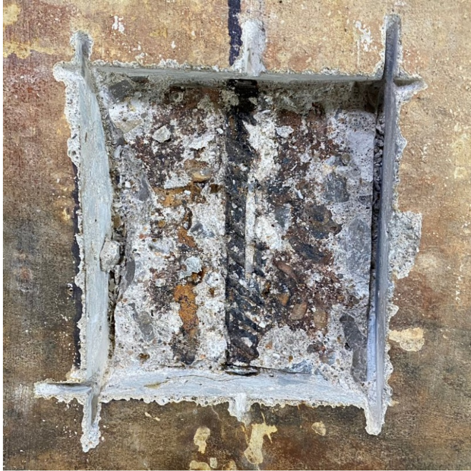
Figure 5-13: CAA-N observed rebar B, 37 days tested
