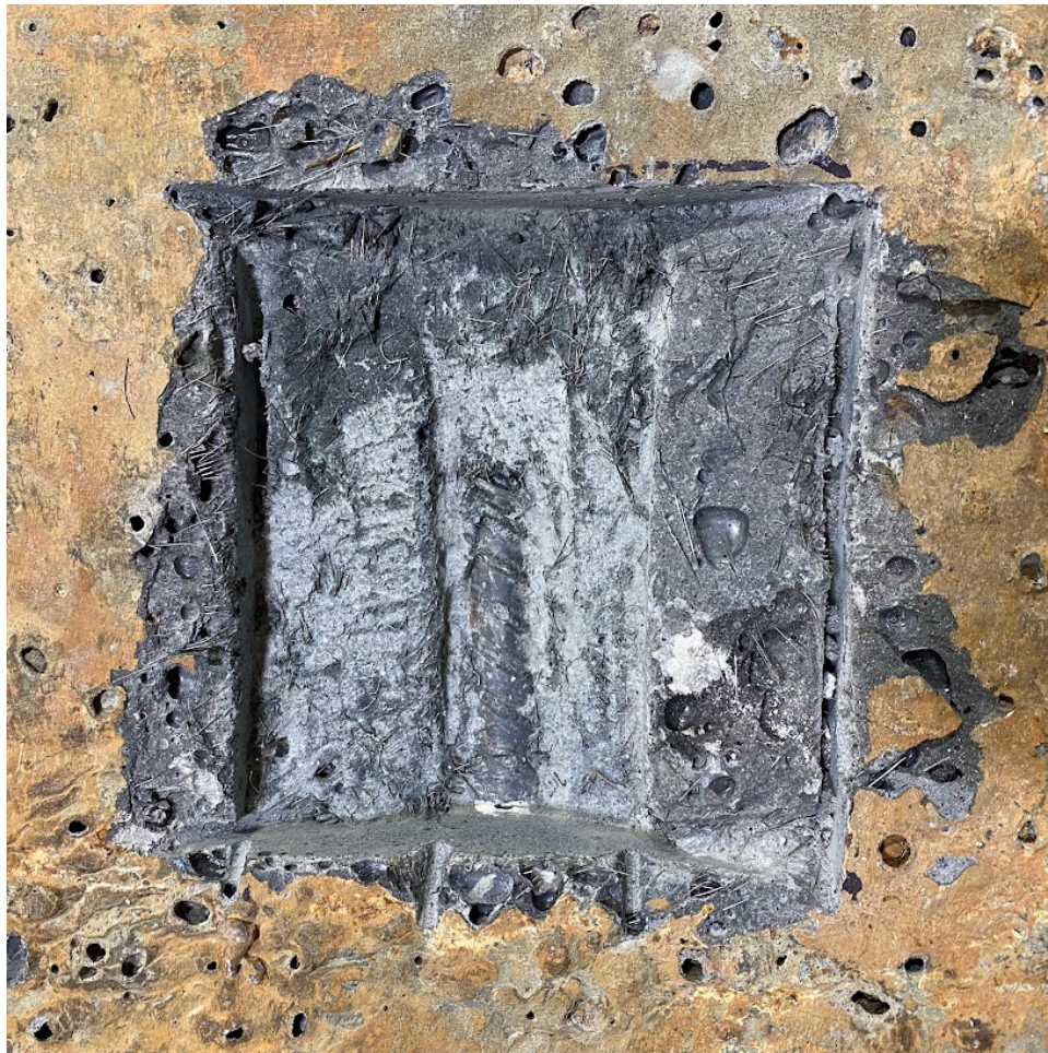
Figure 5-29: CU-L observed rebar C, 65 days tested
