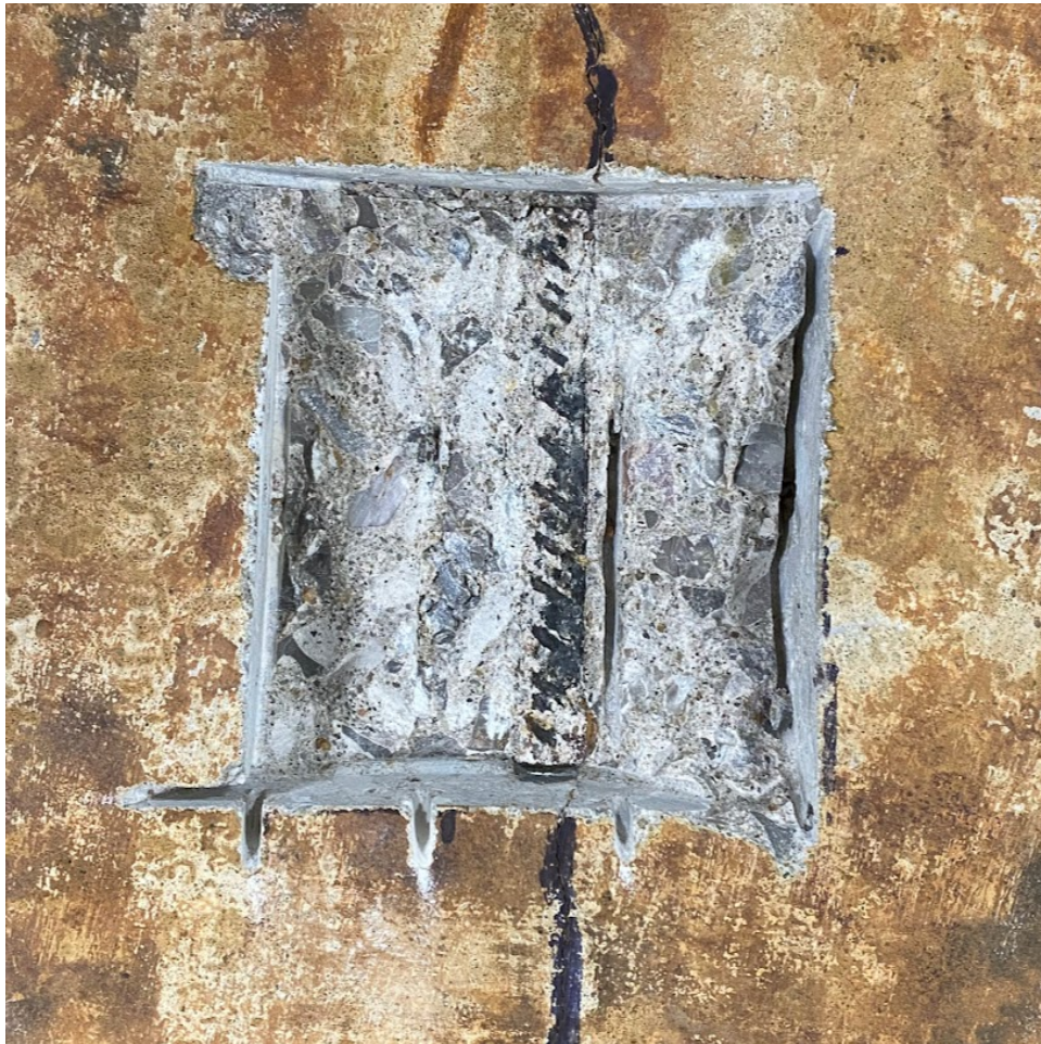
Figure 5-26: CAA-N observed rebar C, 65 days tested
