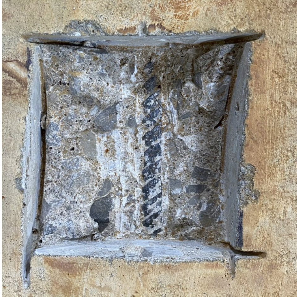
Figure 5-9: CAA-L observed rebar B, 37 days tested
