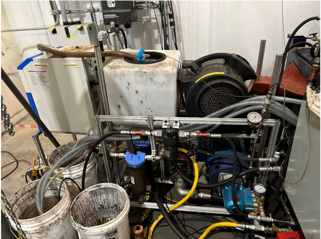
Figure 19: Various Components in the Cooling System
