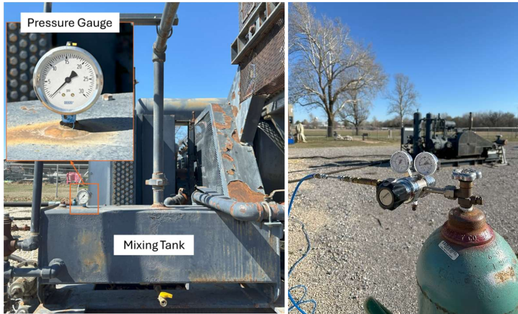
Figure 10: (left) Mixing tank pressure gauge, (right) hydrogen tank pressure regulator
