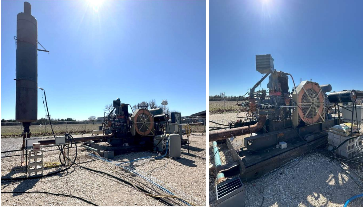
Figure 7: AJAX DPC-105 natural gas-fed, two-stroke compressor
