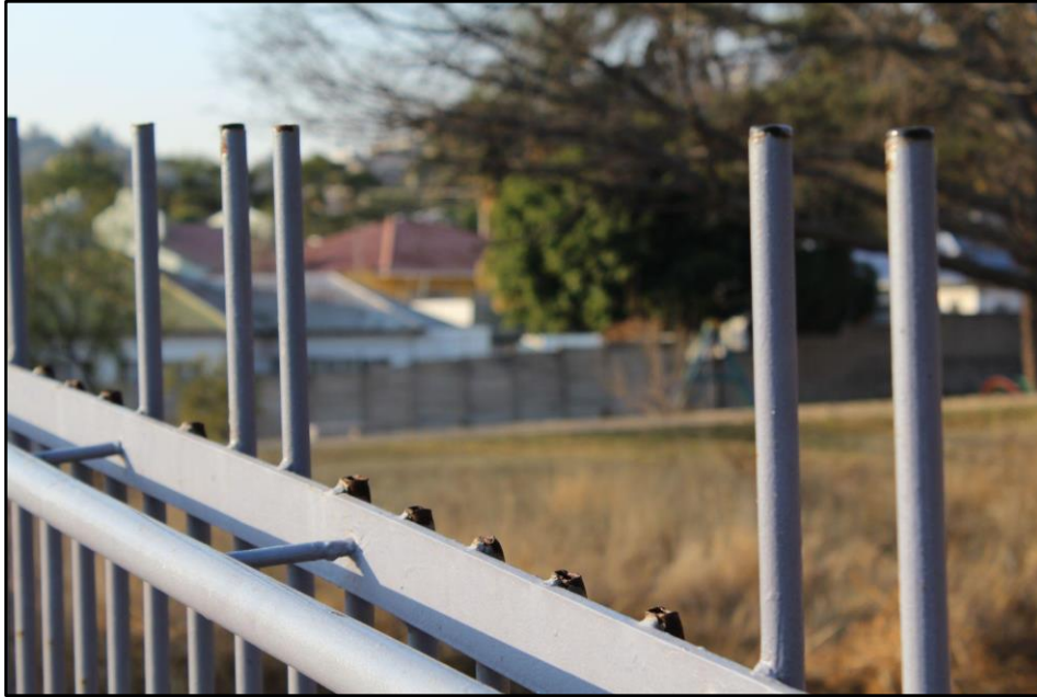
Figure 5.7: Steel bars of railing for the foot bridge crossing a small river (vlei) of Paterson Park welded off and sold to local metal scrapyards (Photo by Le Roux, 2021).
