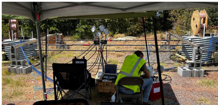
Figure 7.15 – Hydraulic manifold with pressure gauges for each of the four jacks.
