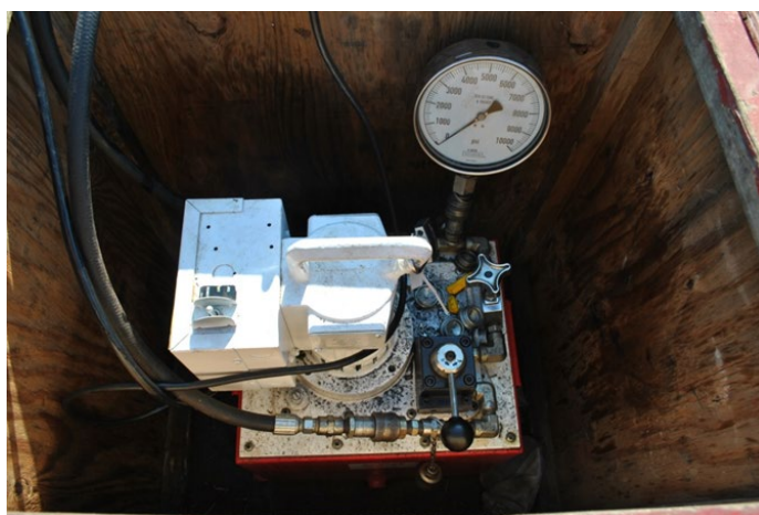
Figure 7.14 – Hydraulic pump with pressure gage.
