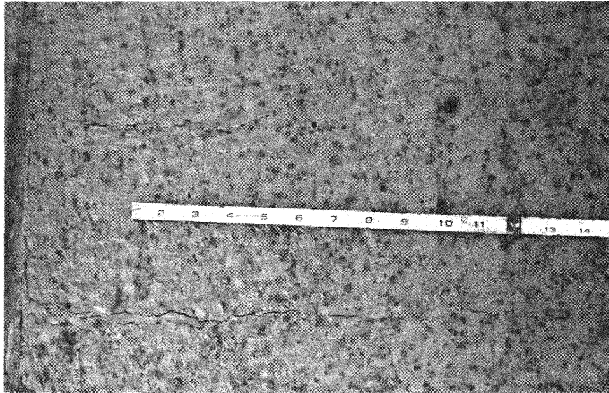
Figure 6 a. Presence of Longitudinal Shrinkage Cracks Before Surface Revibration (RVS-91).
