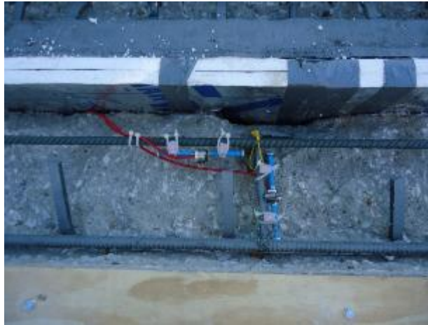
Figure 331. Strain gauges within the joint header
