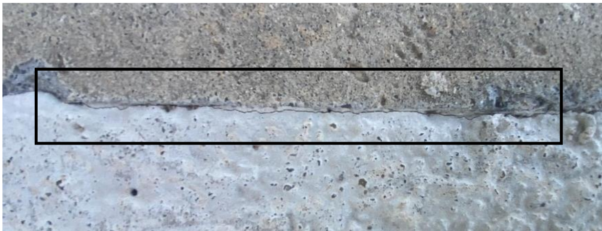
Figure 39: Shrinkage Crack on Large-Scale RS-SCC Repair Slab
