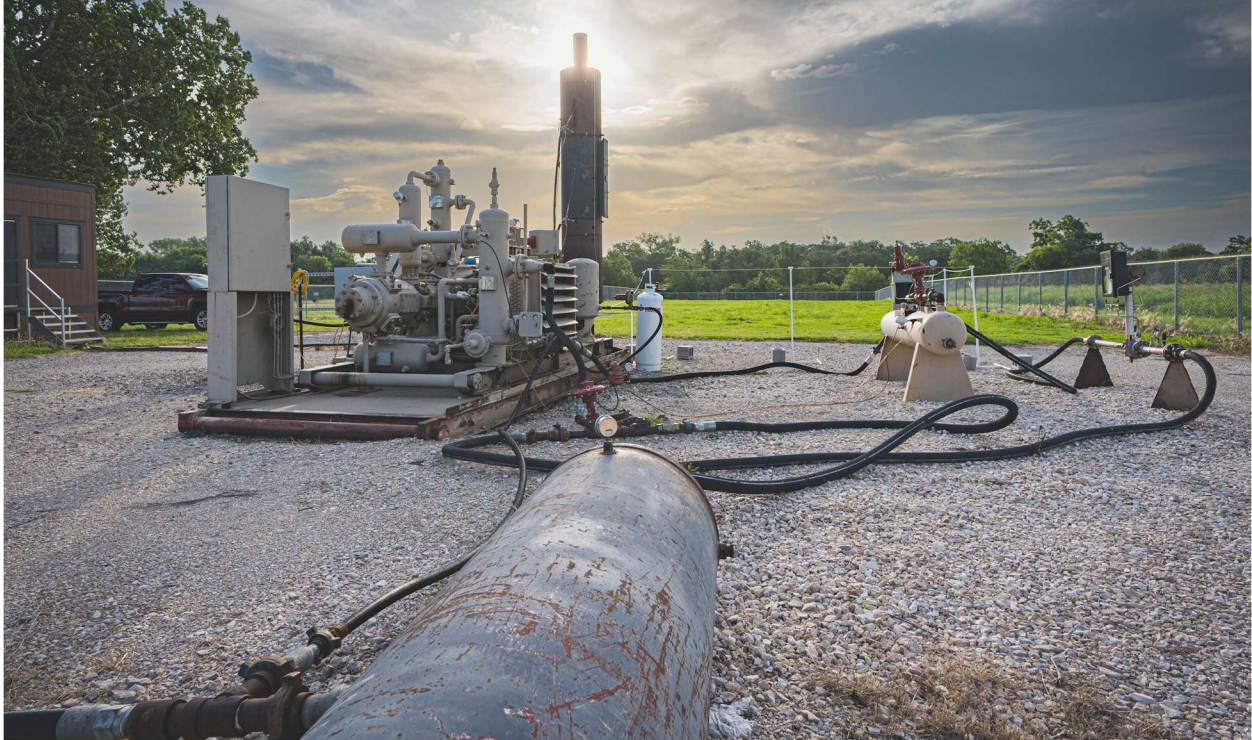
Figure 9: AJAX DPC-81 Suction and Discharge Setup
