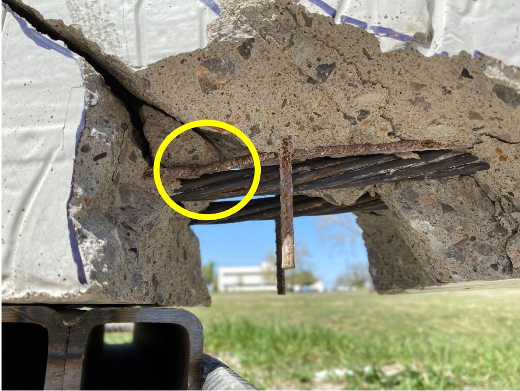
Figure 137: WWR failure mode from shear failure in beam B14-24DV – tensile yielding of gross section
