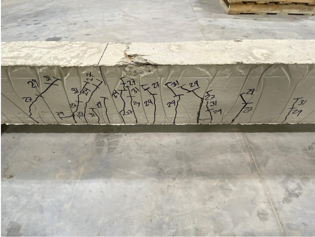
Figure 111: Compression block crushing and flexural cracking in beam B6-3DV (dead end)
