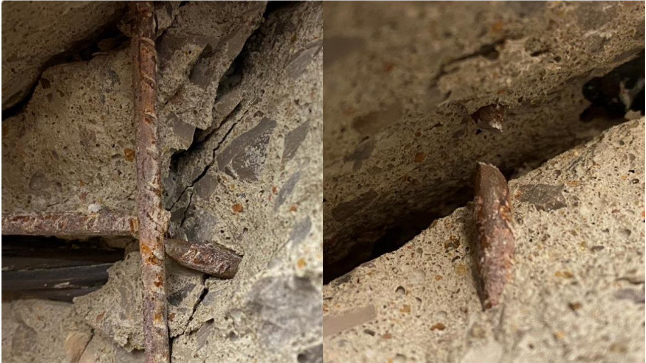
Figure 118: WWR failure modes from beam shear - welded junction failure (left) and rupture of gross section (right)
