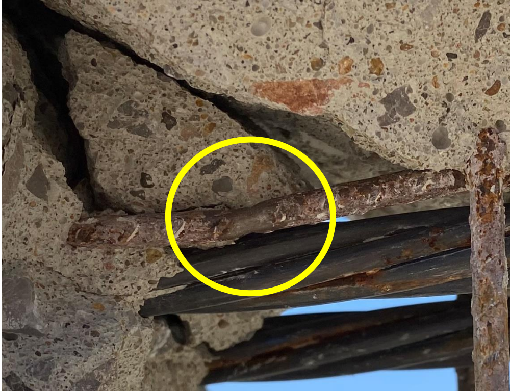
Figure 138: Magnified view of tensile yielding in WWR after beam B14-24DV shear failure
