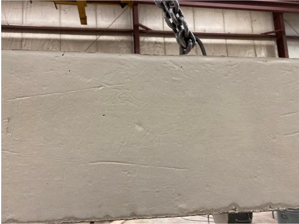
Figure 98: Close-up view of Trial beam B2 showing smooth beam surface free of bug holes
