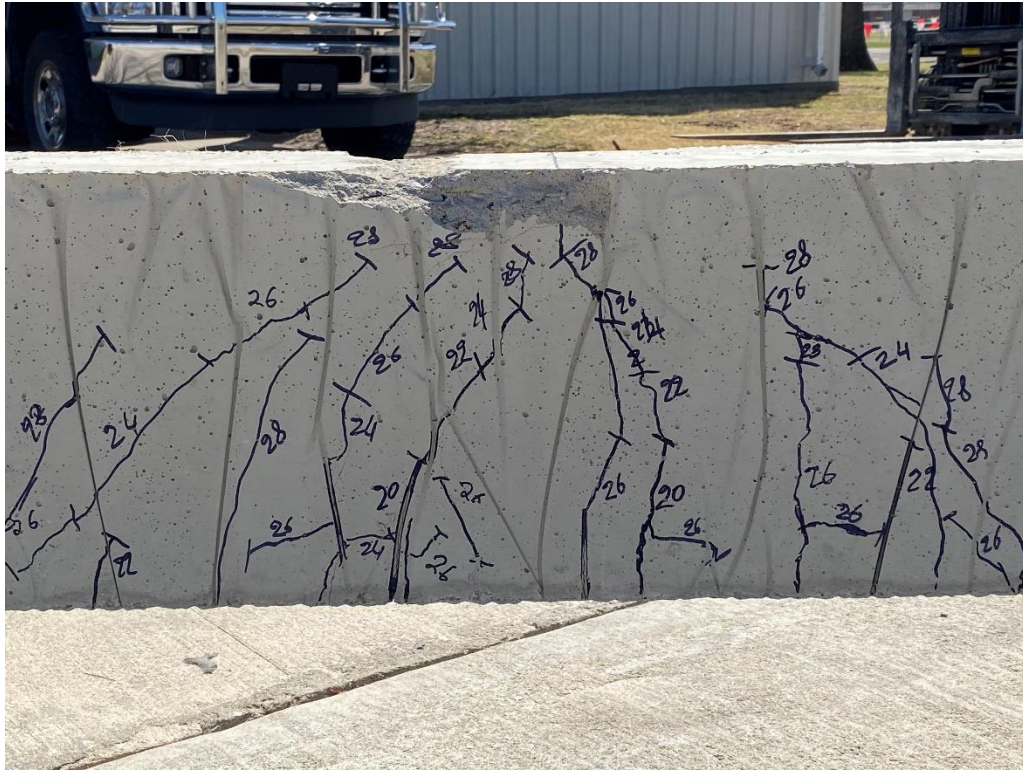
Figure 108: Compression block crushing and flexural cracking in beam B9-3DV
