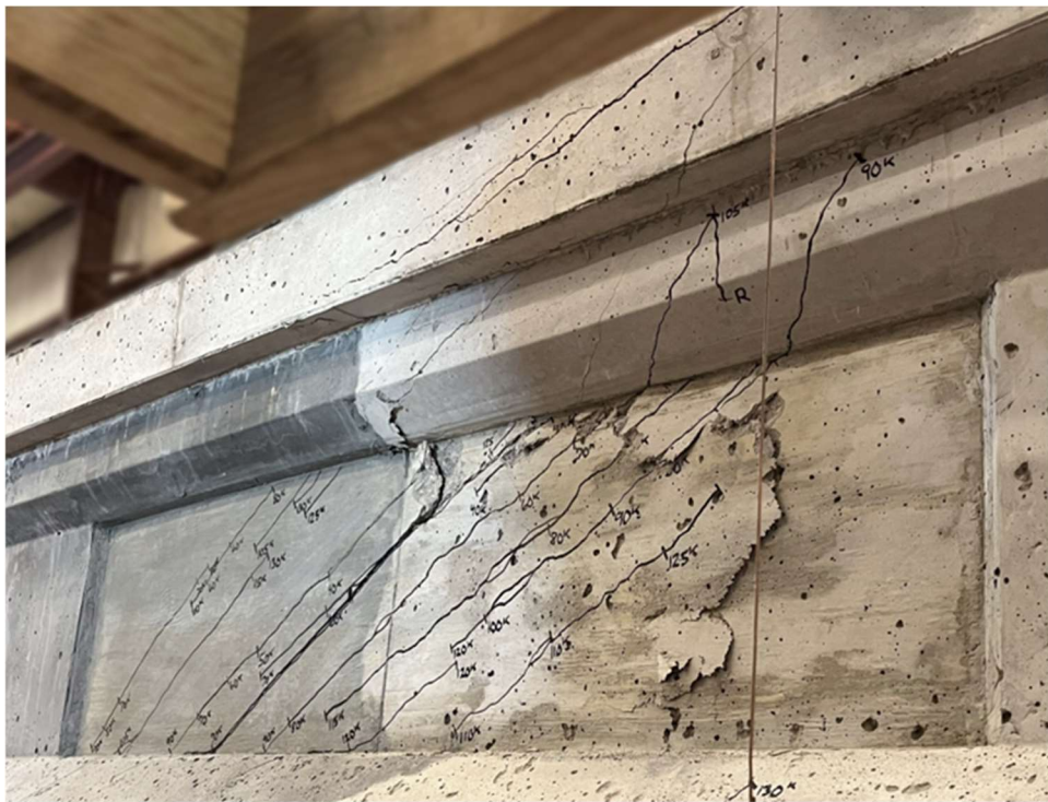
Figure 6.14: Observed, post-testing failure in BiFluid with Divider Girder No. 2
