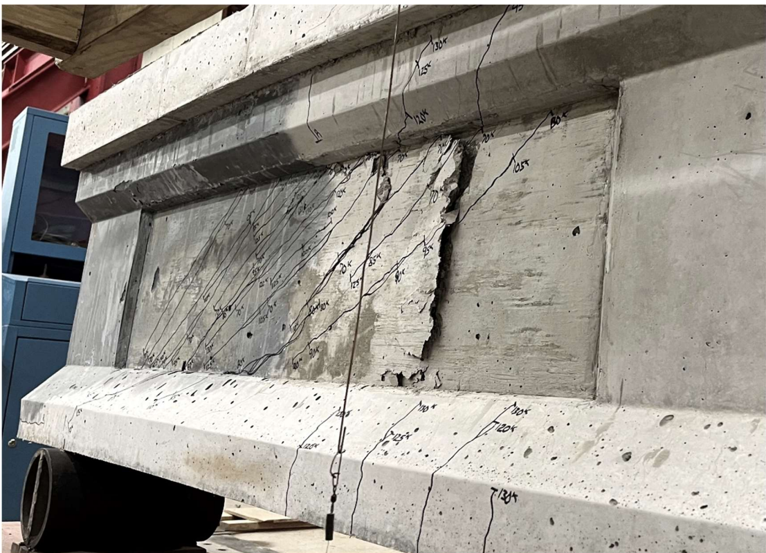
Figure 4.16: Failure of BiFluid hybrid girder no. 2
