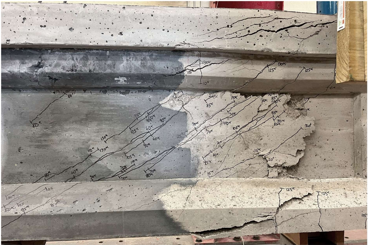
Figure 6.2: Post-failure damage observed in BiFluid Girder No. 1
