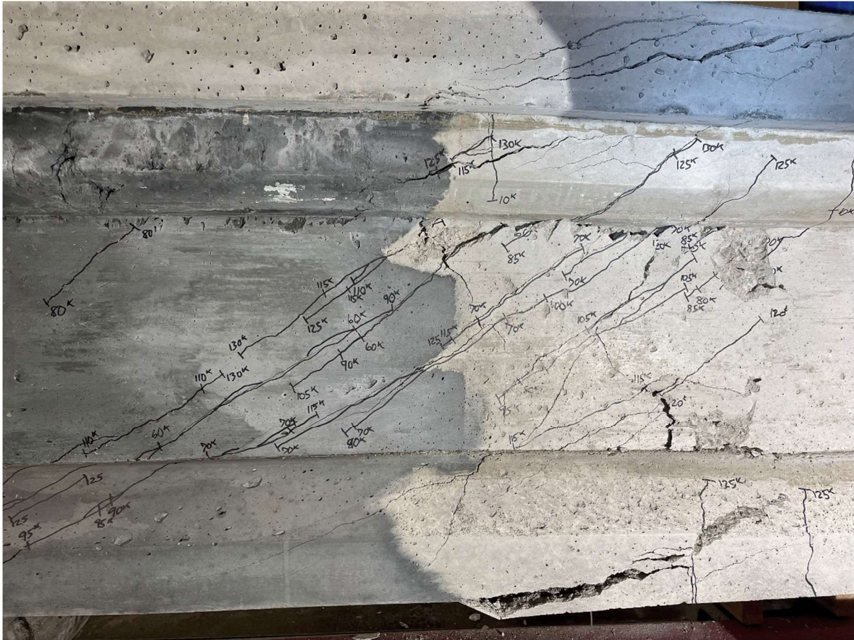
Figure 6.1: BiFluid Girder No. 1 cracking in the shear span up to failure
