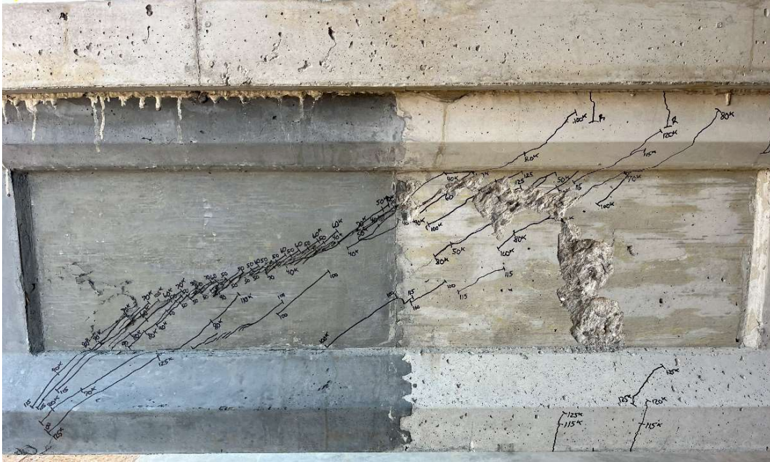
Figure 4.29: Failure of 3D textured hybrid girder no. 1
