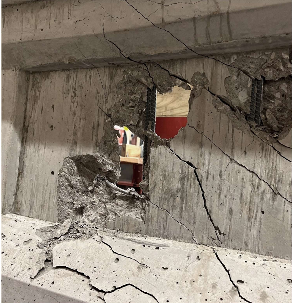
Figure 6.6: Observed, post-testing failure in BiFluid Girder No. 2 on the unmarked face (backside of girder)
