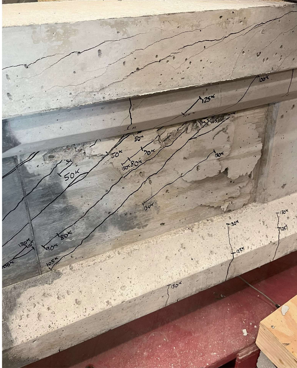
Figure 6.12: Observed, post-testing failure in BiFluid with Divider Girder No. 1
