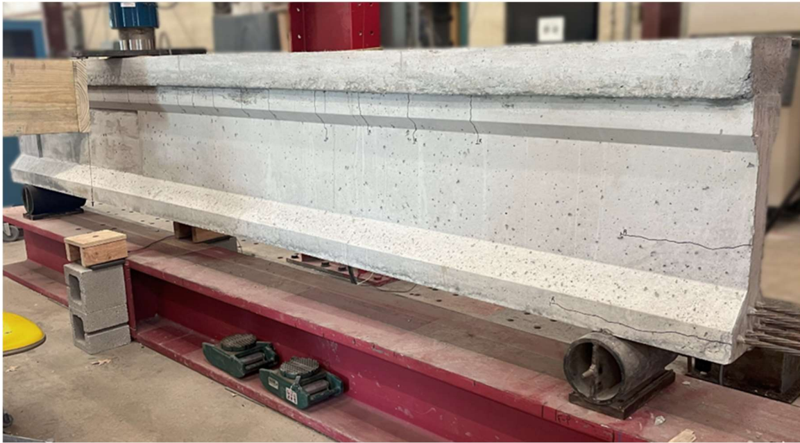
Figure 6.7: Observed cracking due to prestressing forces in BiFluid Girder No. 3
