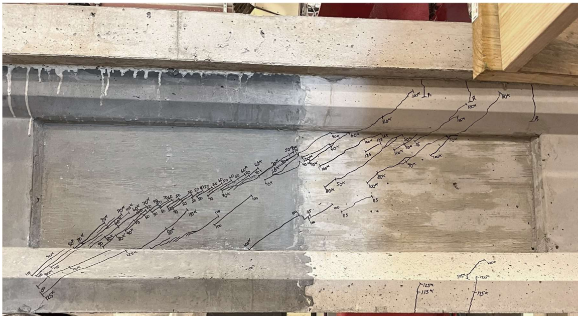
Figure 6.24: Crack propagation at 125 kips applied load for 3D Trapezoidal Girder No. 1
