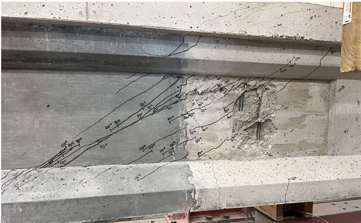
Figure 4.26: Failure of 2D textured hybrid girder no. 1
