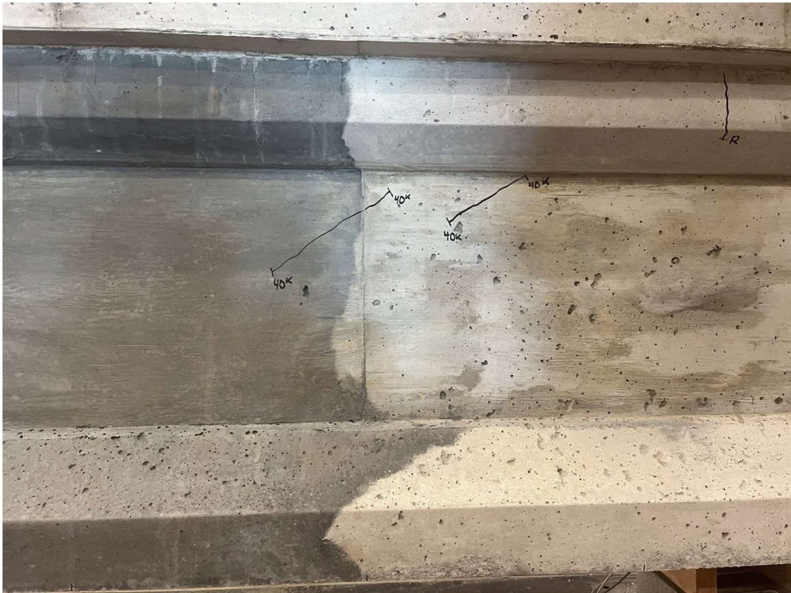
Figure 6.13: Initial cracks observed in BiFluid with Divider Girder No. 2
