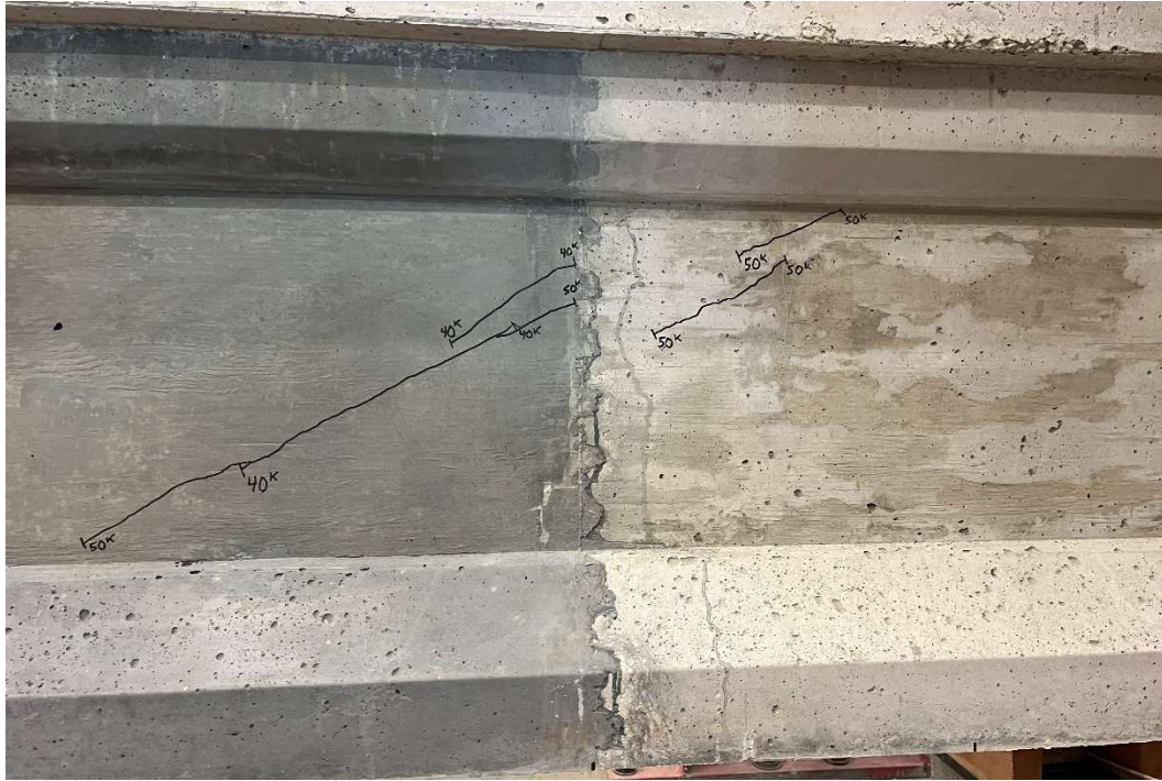
Figure 6.16: Initial cracks observed in 2D Trapezoidal Girder No. 1
