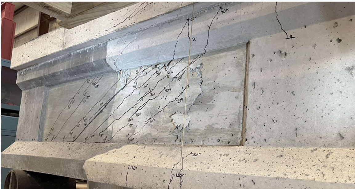
Figure 4.21: Failure of BiFluid with Divider hybrid girder no. 2
