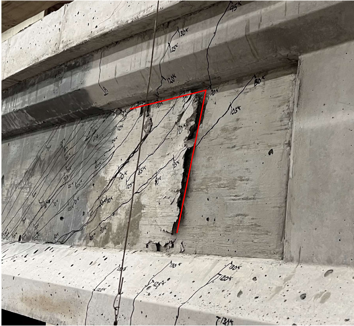
Figure 6.5: Highlighted failure path of web failure in BiFluid Girder No. 2
