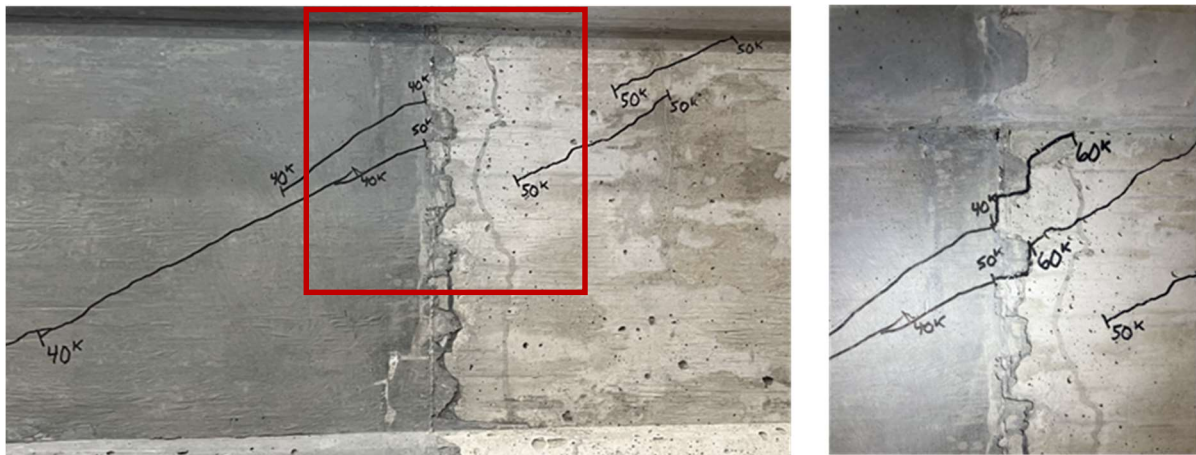
Figure 4.23: First cracks to propagate in 2D Trapezoidal hybrid girder no. 1 (left); further crack progression at the interface (right), photo taken of the region outlined in red
