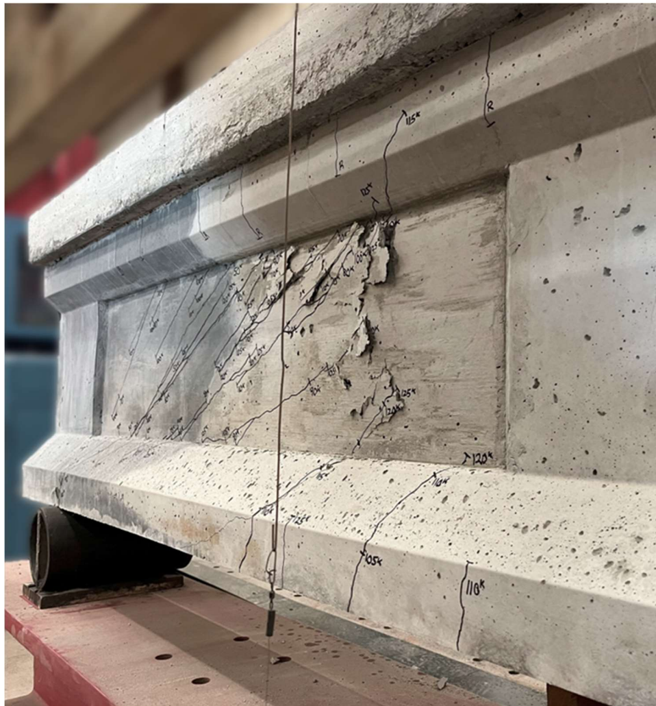
Figure 6.29: Representative extents and location of web crushing behavior in hybrid girder specimens 6
