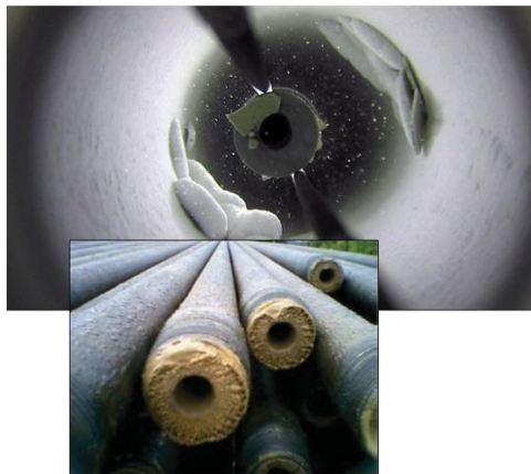
Figure 2-1. Scaling in PCK (taken from www.zerlux.com/hard-scale-removal )
