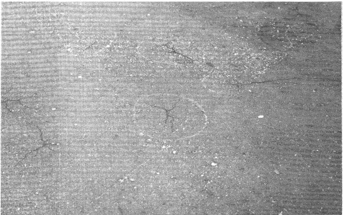
Distress in A. C. Overlay resulting from blister formation under Royston membrane.
