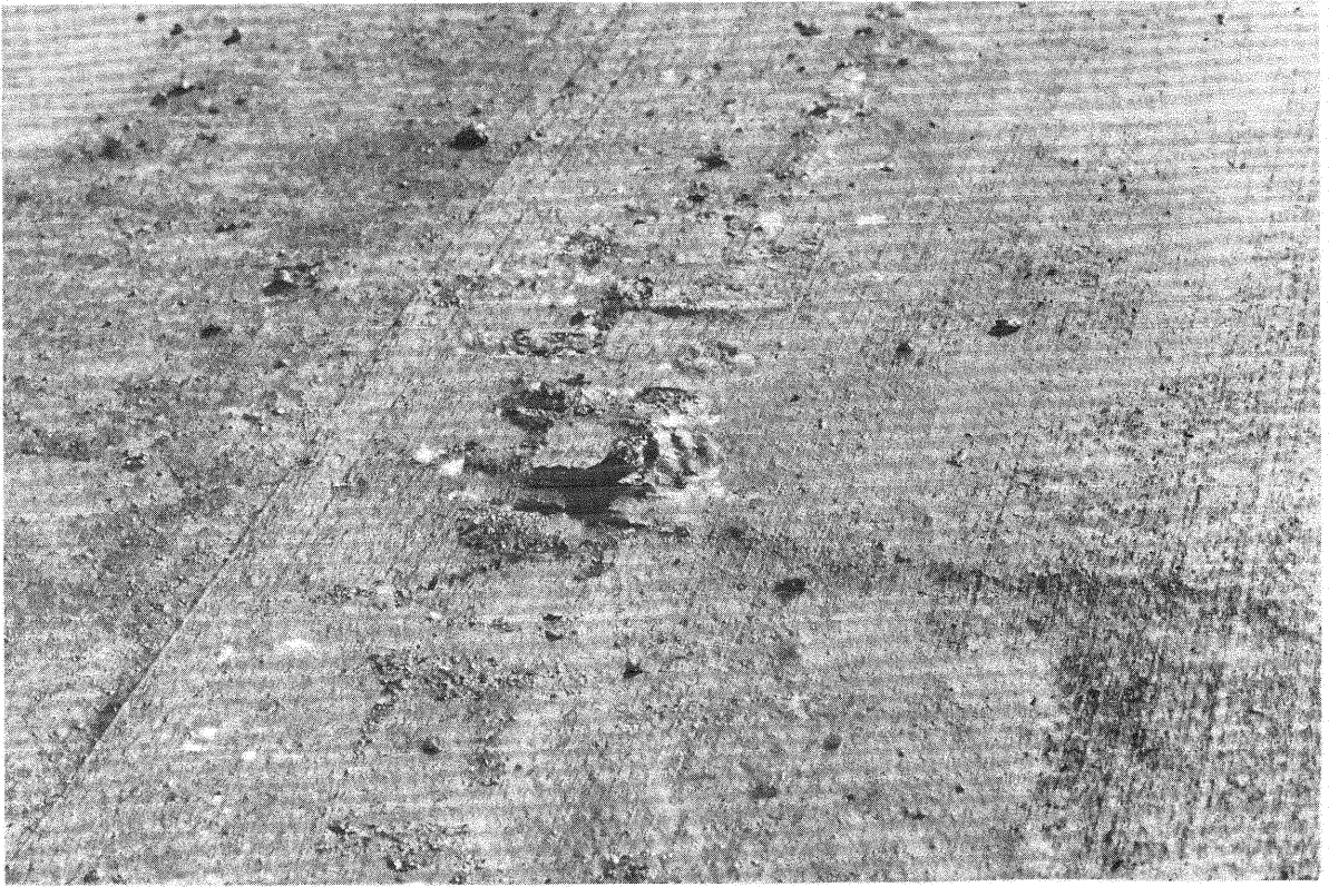
Damage to membrane caused by paver's tracks.
