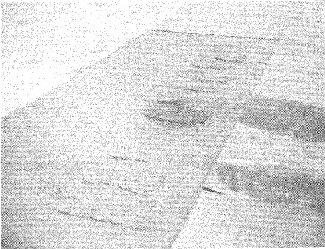
Damage caused to asphalt roofing sheet and membrane by paver's tracks.
