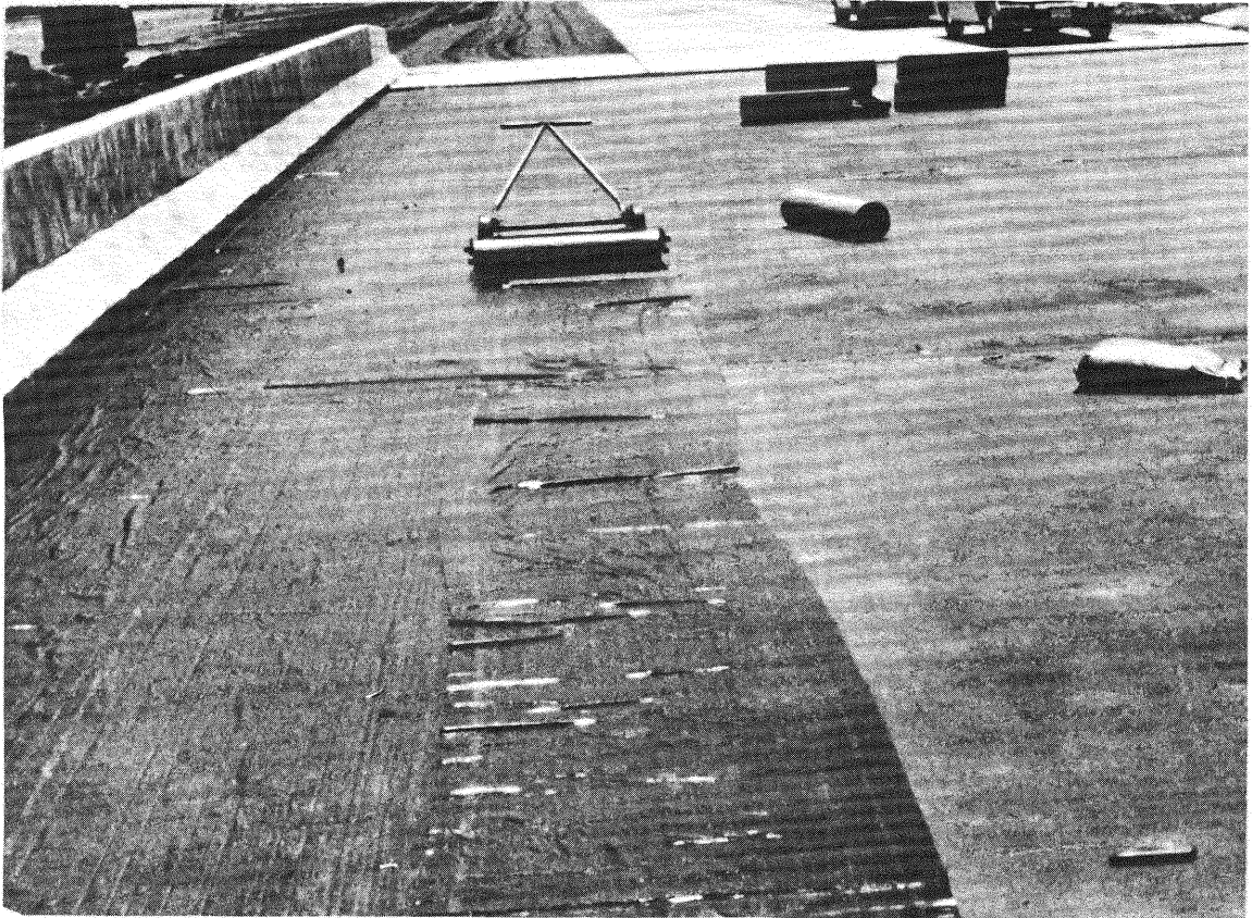
Application exhibiting good and poor workmanship.
