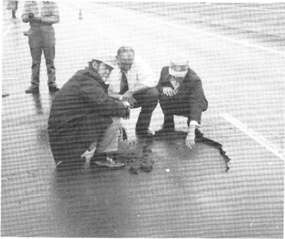
Type of failure encountered in first Bituthene application approximately six (6) months after application.
