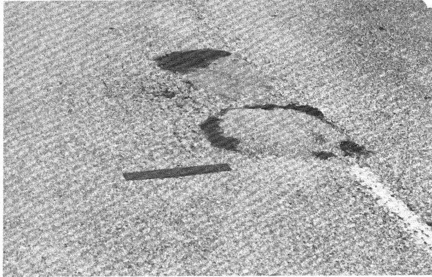
Typical failure of A.C. surfacing over Polytok membrane.
