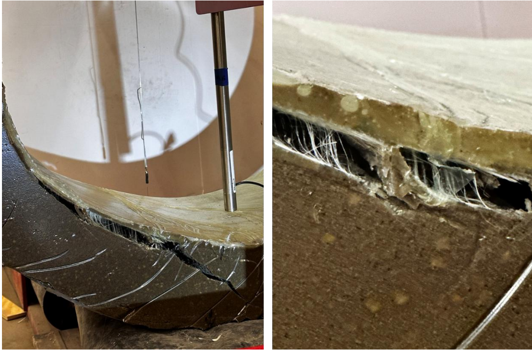
Figure 58: Bridging between GFRP pipe and polymeric grout
