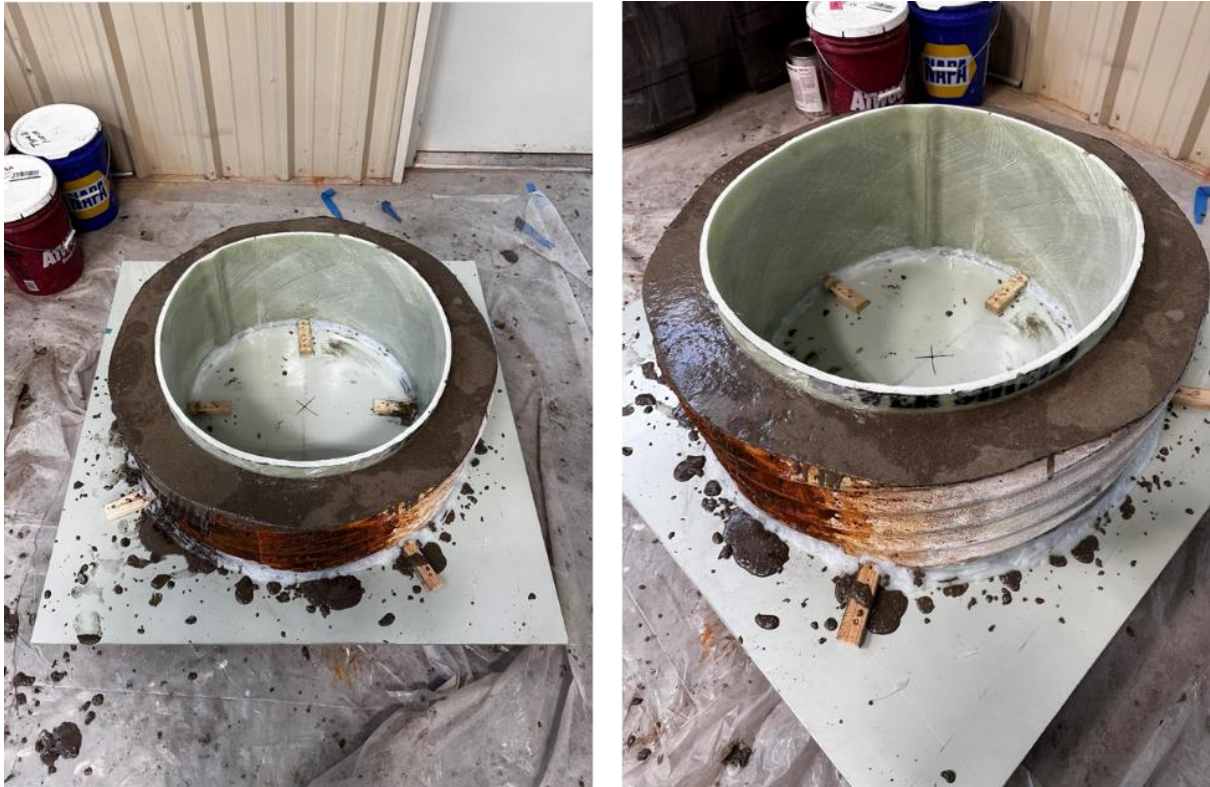
Figure 50: Corroded CMP with polymeric grout
