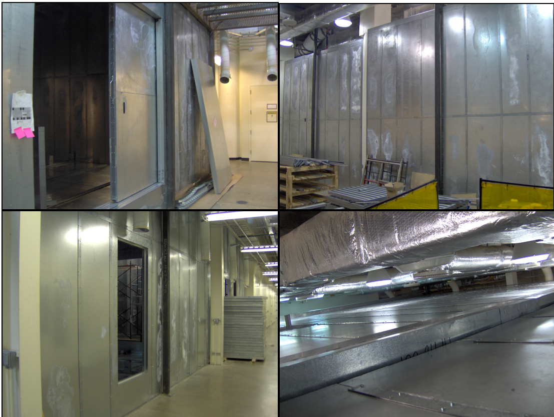
Figure 1.6: Photographs of completed chamber envelope – Clockwise from top: North wall and main access for units, East wall, West wall containing personnel access doors, and roof
