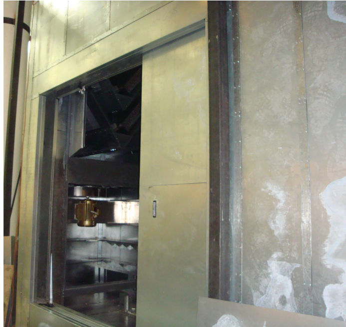
Figure 4.8: Main equipment entrance door – lintel seen at top of the doorway (north wall)
