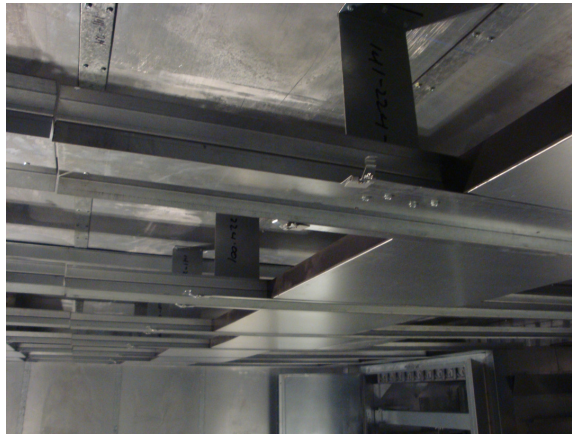
Figure 4.21: Left: Filter sleeves and ceiling plenum assembly
