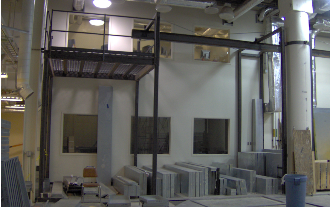
Figure 4.28: Mezzanine with accompanying trolley beam erected in basement of ATRC before construction of chamber
