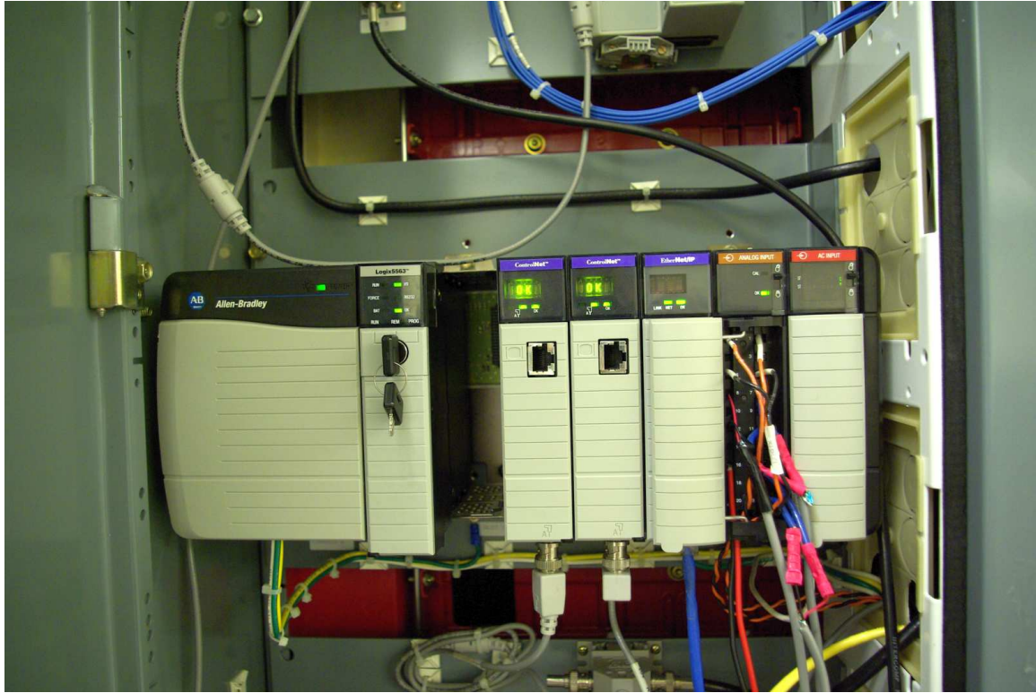
Figure 2.4: ACDrive Controller Rack
