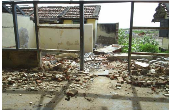
Photo 3: Nagapattinam Hospital sustained extensive damage
