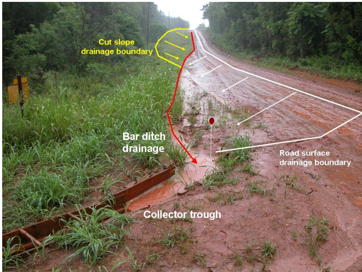
Figure 3. View of the westward draining road segment (32 NE) at the 32 nd St. site with drainage boundaries drawn in.
