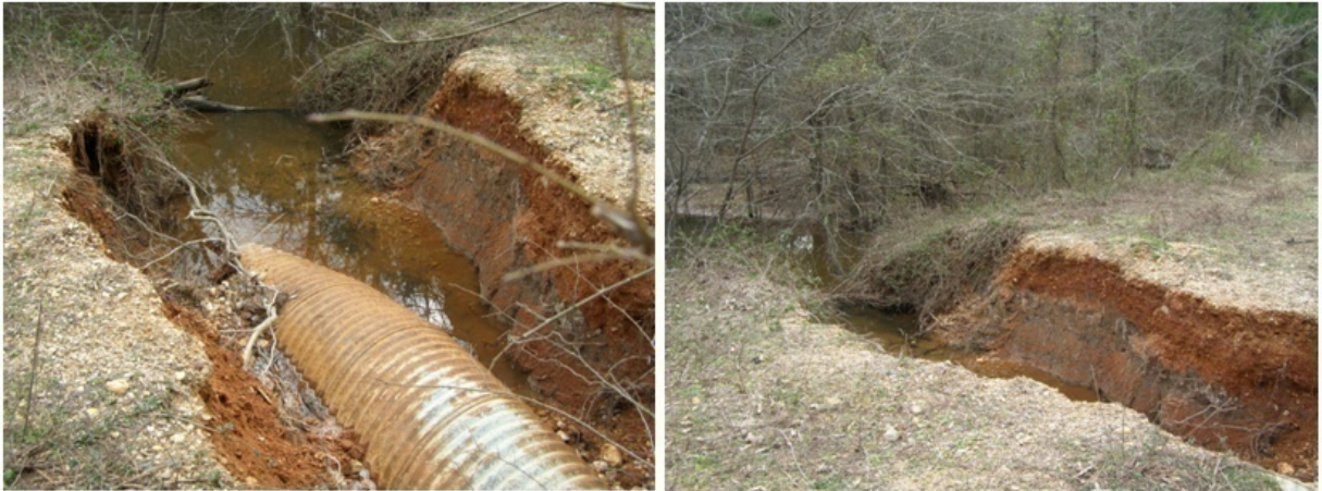
[Figure 9: Failed Culvert and Erosion]
