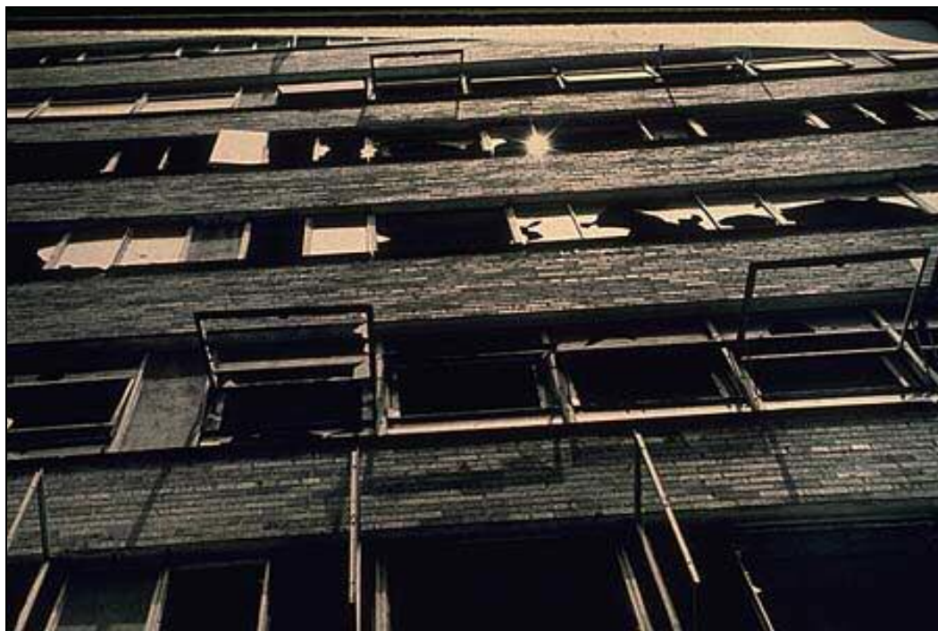
Fig. 11: Vandalized Windows at Pruitt-Igoe. Source: Oscar Newman, Creating Defensible Space .
