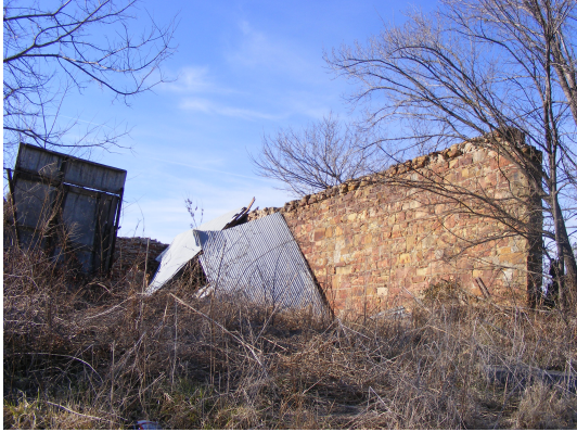
FIGURE 3.1 - Abandoned Building at Heyburn Townsite
