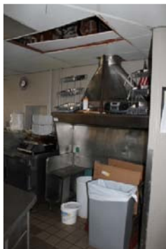
Hood Vent and wall surround, Not currently used in facility
