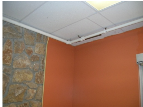
Bakery Ceiling with visible sprinklers
