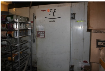
Dry Storage Room Freezer, Operational
