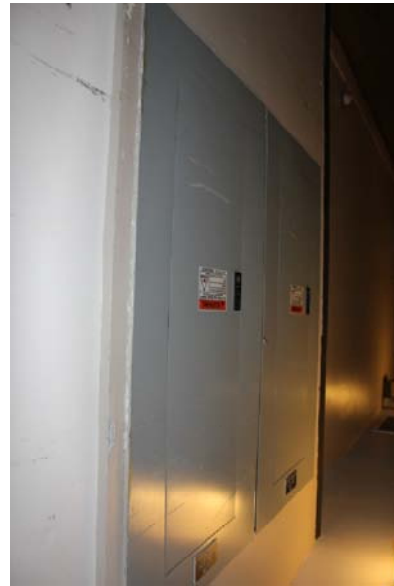
Electric Box in Corridor
