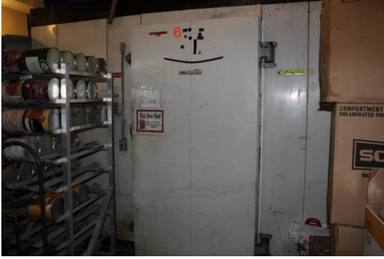
Freezer in Dry Storage area
