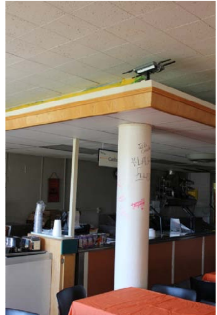
Wireless Equipment, Building has WiFi for customer usage
