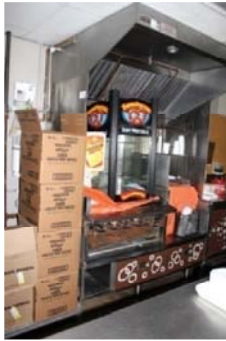
Vent Hood with Grill Top under and Fryer. Image show Pretzel warmer on top of Grill Top. All operational, Pretzel warmer is only piece currently used
