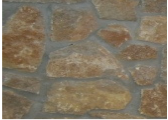
First floor masonry under windows and on east side of first floor area
