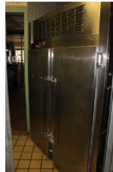
Reach in/Cart Roll in Coolers, Little Bakery Prep area
