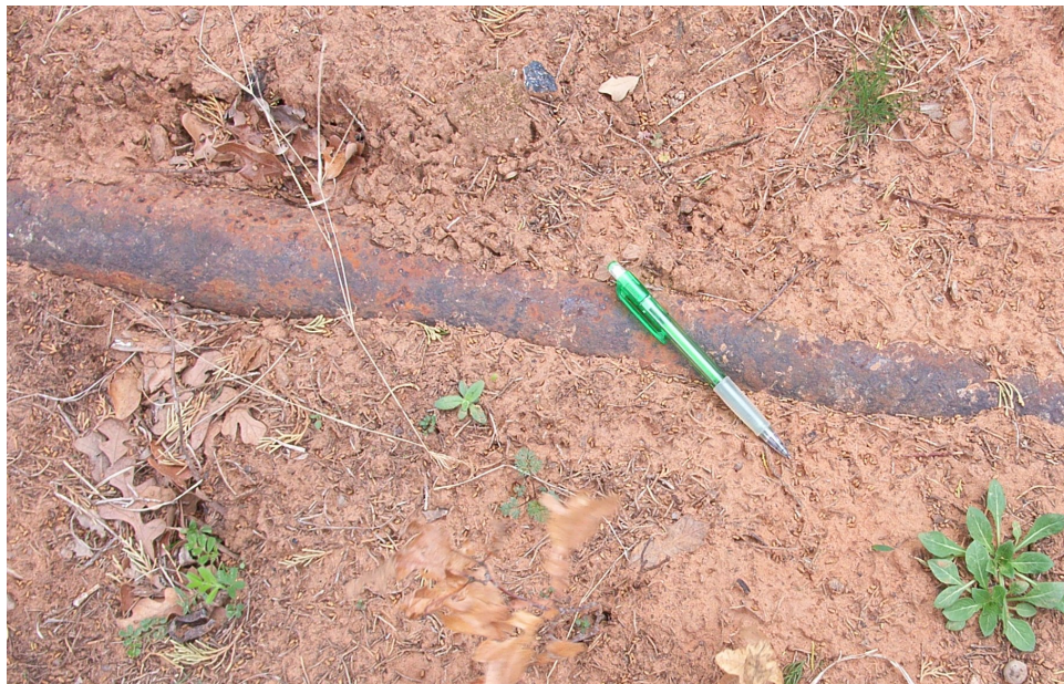
Figure 3.12: an Exposed Petroleum Pipe Found near the ERI Line TH.G
