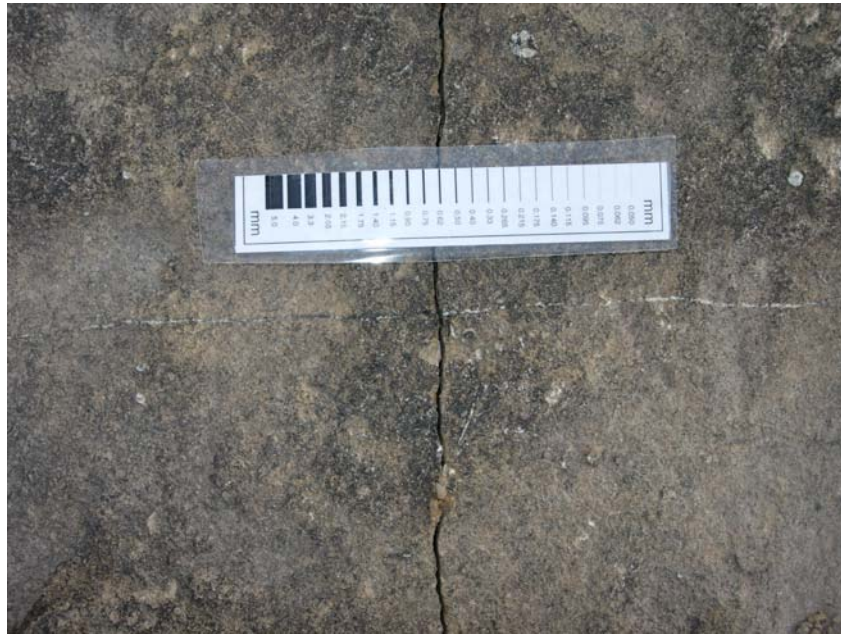
Figure 29: An image showing a fracture (N75°E) filled with calcite being cross-cut by a younger fracture (N15°W) at the Brownwood Spillway
