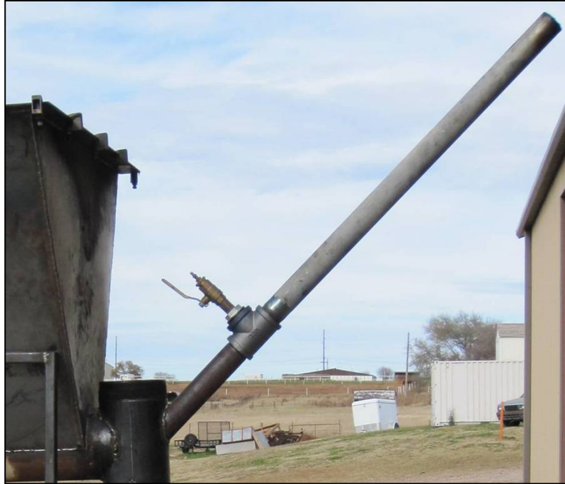
Figure 21: Producer gas outlet with sampling port.
