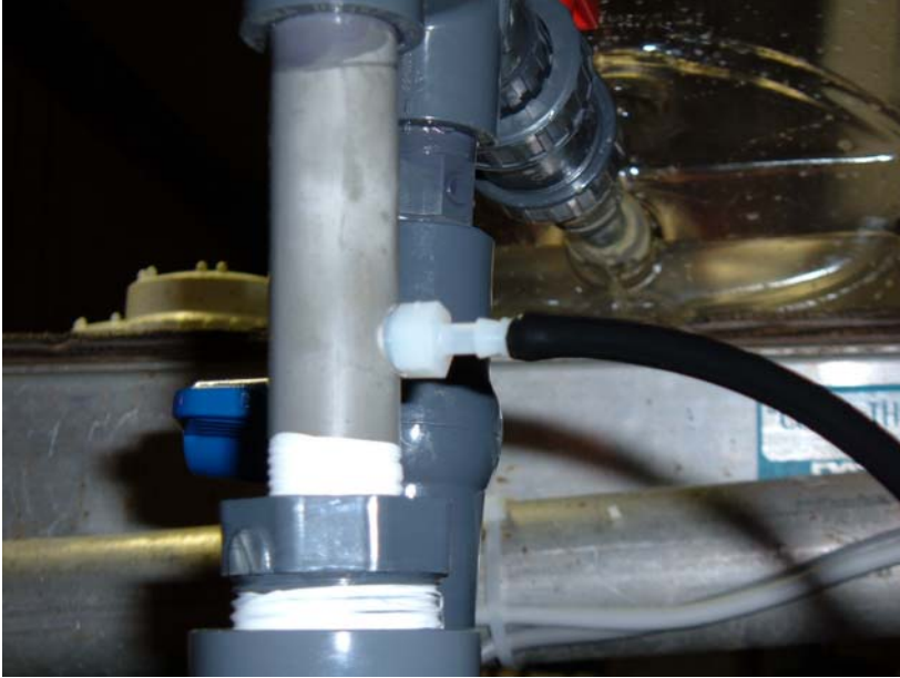
Figure 15: Injection tap into test water delivery line
