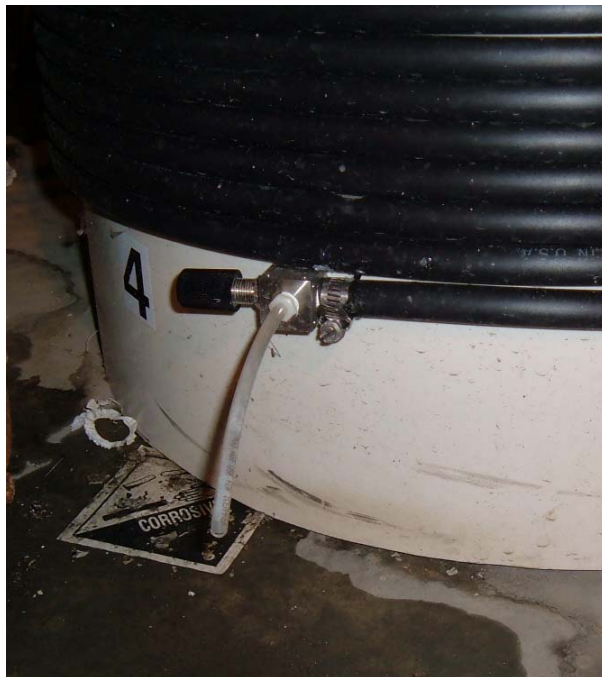
Figure 3: Needle valve at the bottom of the irrigation tubing
