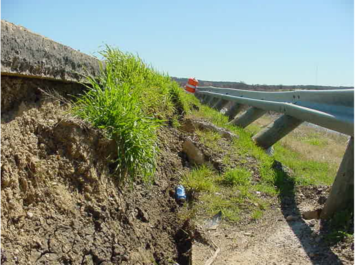
Figure 56. Slope Failure Scarp at Roadway Edge – Lake Ridge Pkwy
