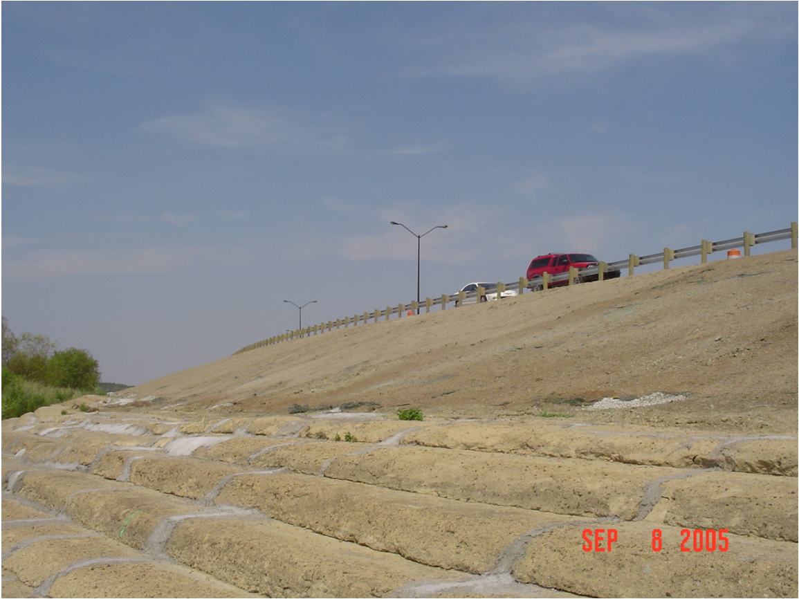
Figure 62. Up-Slope View of Completed FRS Slope Prior to Grass Establishment (Existing Soil-Cement in Foreground) – Lake Ridge Pkwy
