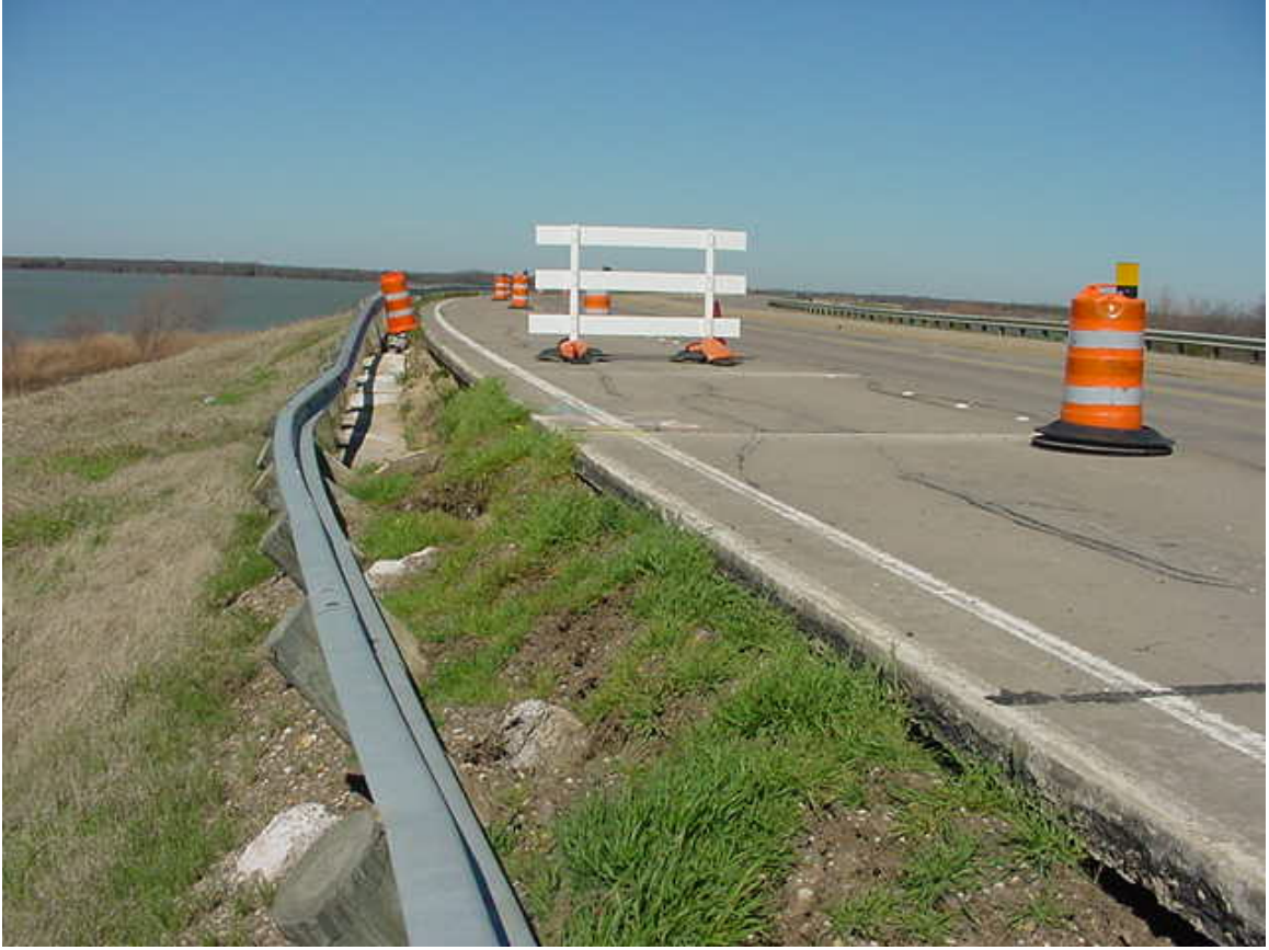
Figure 55. Slope Failure on Lake Ridge Parkway
