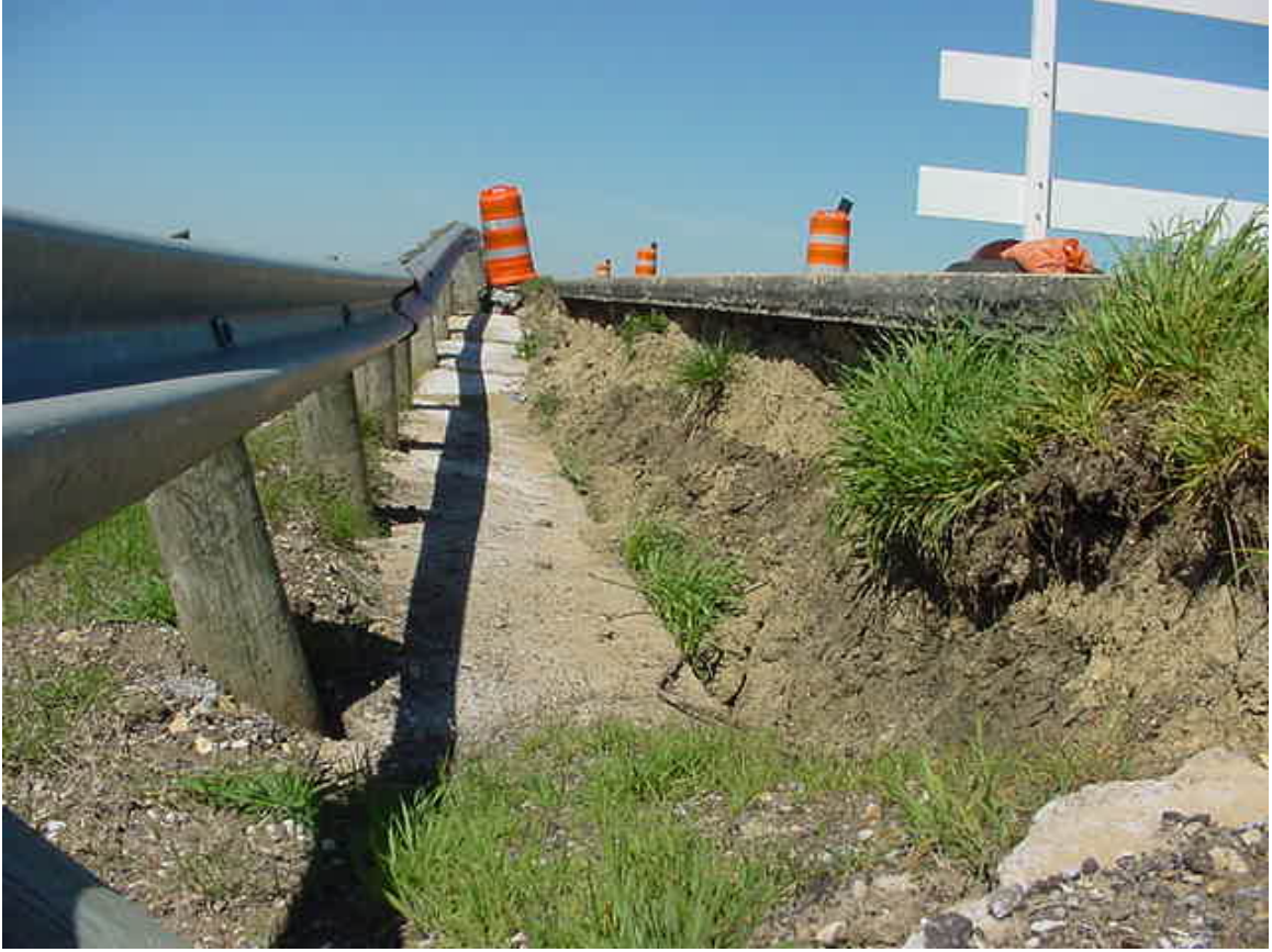
Figure 57. Slope Failure at Roadway Edge – Lake Ridge Pkwy
