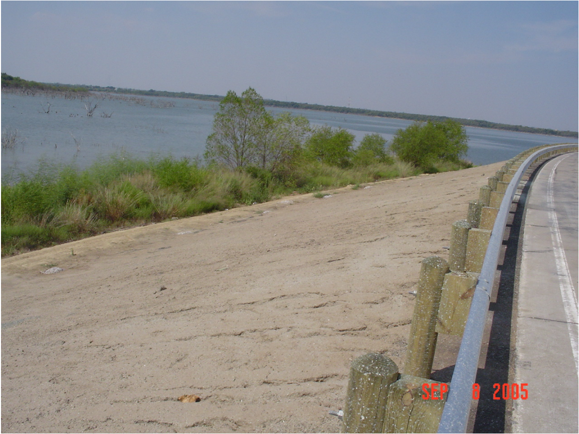
Figure 61. Down-Slope View of Completed FRS Embankment Prior to Grass Establishment - Lake Ridge Pkwy
