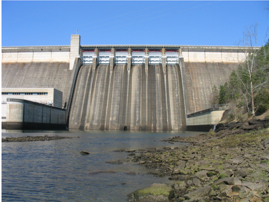
Figure 8. Greers Ferry Dam and tailwater. The dam's powerhouse is visible at the far left.
