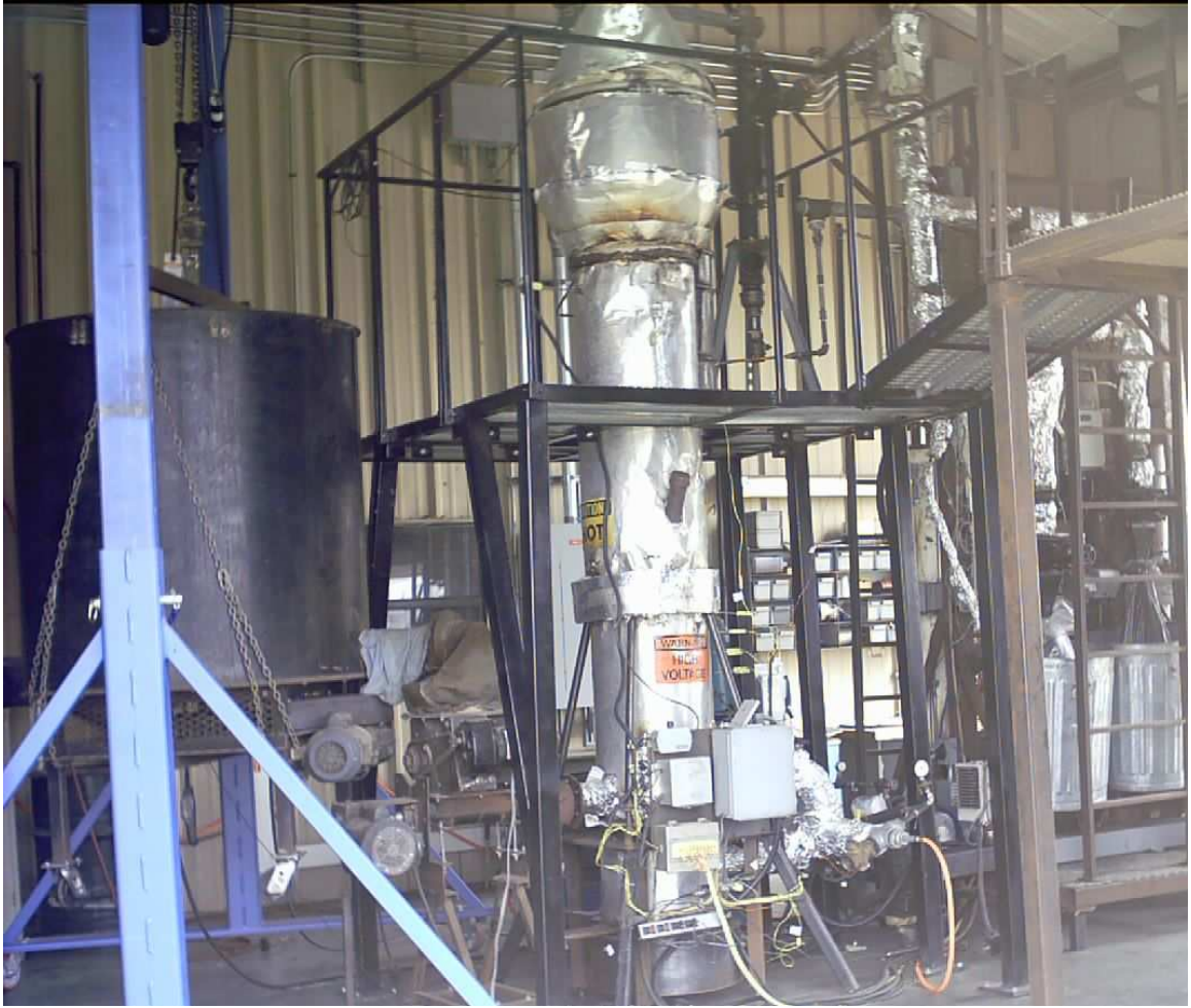
Figure 2.10 Gasifier pilot plant
