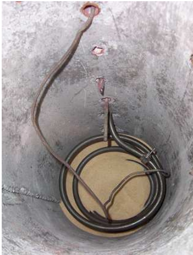
Figure 2.6 Baffle heaters in sand bed
