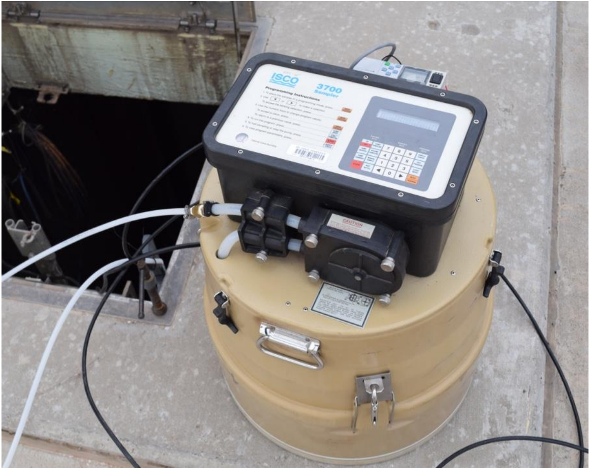
Figure 12. Automated waste water sampler placed at ground level beside wet well.
