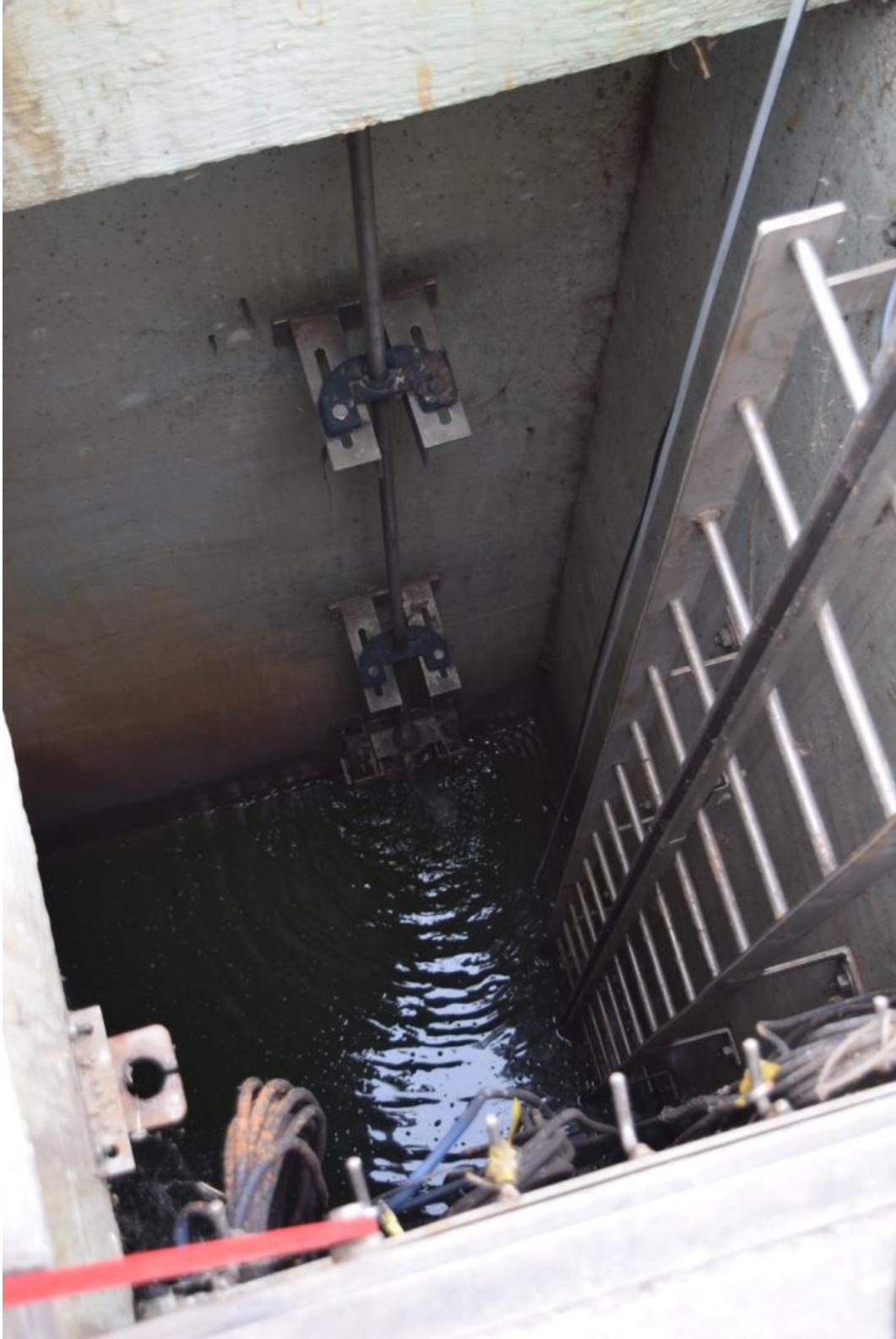
Figure 11. Interior view of wet well at low flow lift station.
