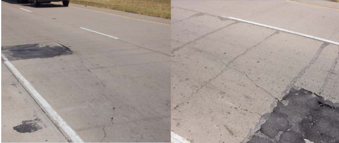
Figure A.49 Multiple transverse cracks intersected by a longitudinal crack
