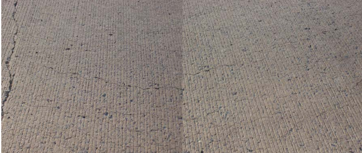
Figure A.67 Map cracking in the south bound lane
