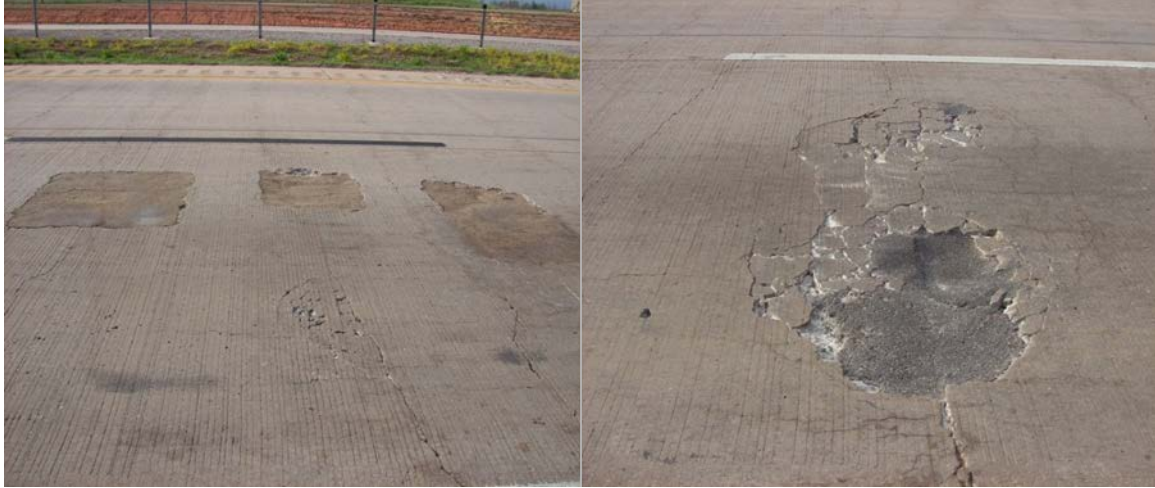
Figure A.81 Map-cracking showed at or near patches in the roadway
