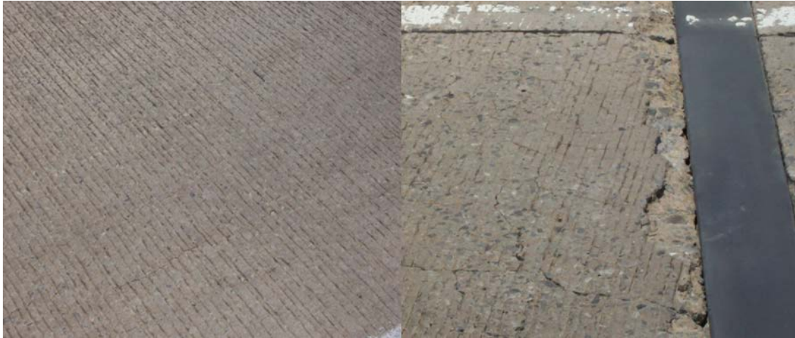
Figure A.65 Close ups showing map-cracking
