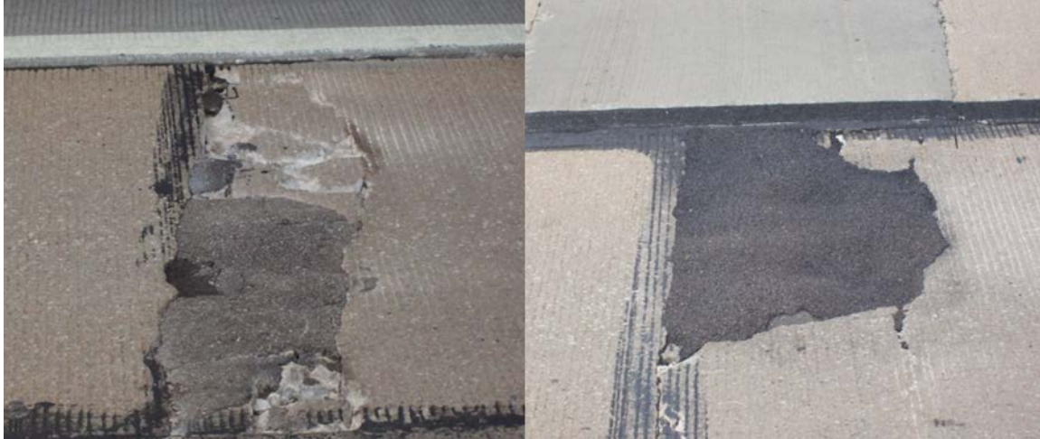
Figure A.28 Patches caused by closely spaced transverse cracks
