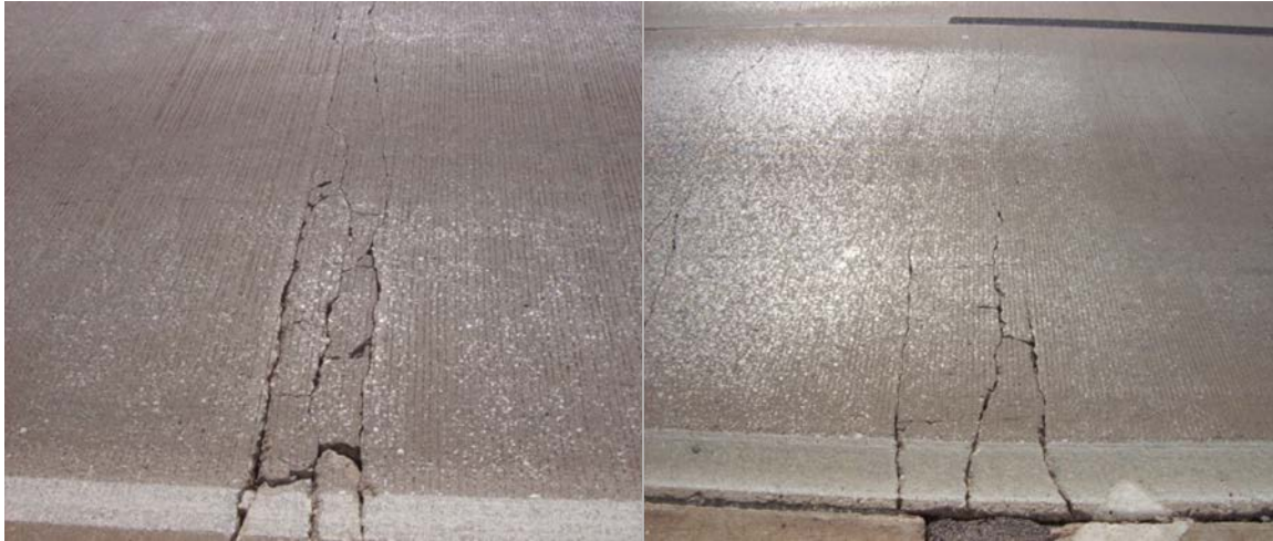
Figure A.4 Photo showing closely spaced transverse cracks developing into punchouts
