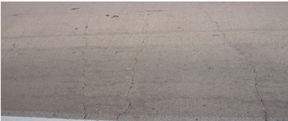
Figure A.55 Stretch of pavement showing signs of map-cracking
