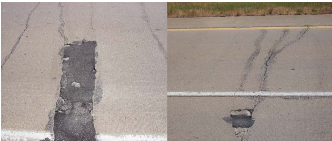
Figure A.50 Patches that appear to be the result of a failed Y-crack
