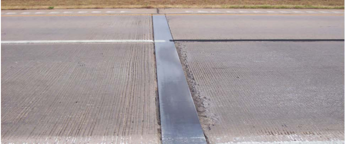
Figure A.21 Deteriorated terminal joint at project beginning
