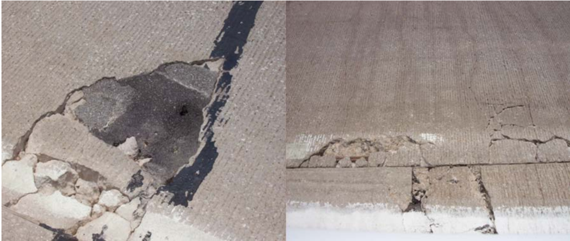
Figure A.30 (left) Y-crack breaking up, (right) distress caused by close transverse cracking
