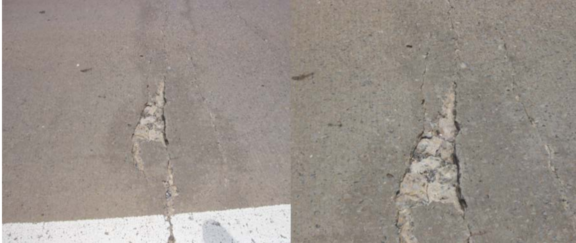
Figure A.62 Y-crack developing into a punch-out
