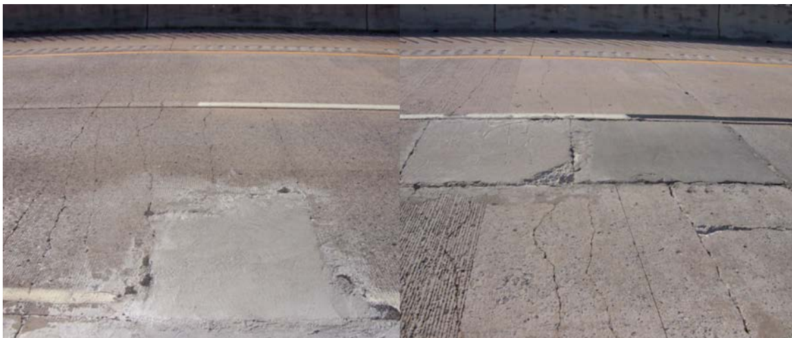
Figure A.64 Patches formed near closely spaced transverse cracks
