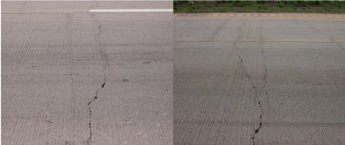
Figure A.84 Closely spaced, nearly intersecting transverse cracks
