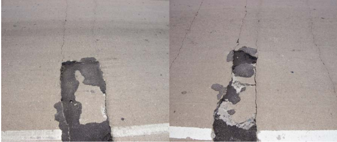
Figure A.45 Transverse cracks intersected by longitudinal cracks
