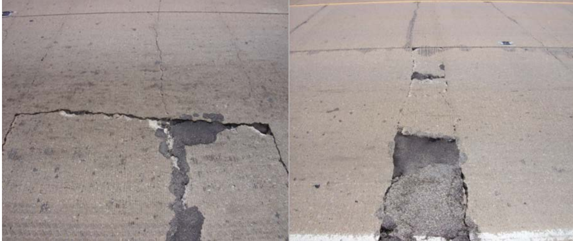
Figure A.47 Transverse cracks intersected by longitudinal cracks
