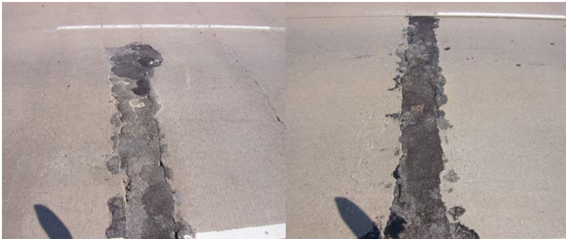
Figure A.41 Patches caused by closely spaced transverse cracks
