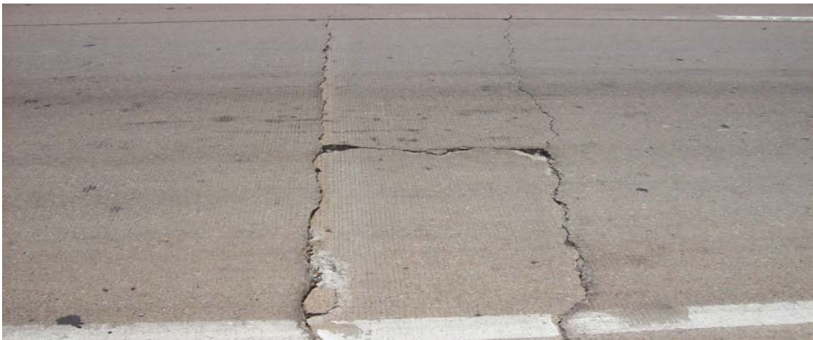
Figure A.48 Two transverse cracks intersected by a longitudinal crack
