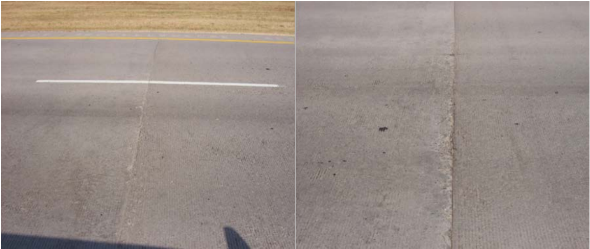
Figure A.16 Two construction joints displaying signs of spalling
