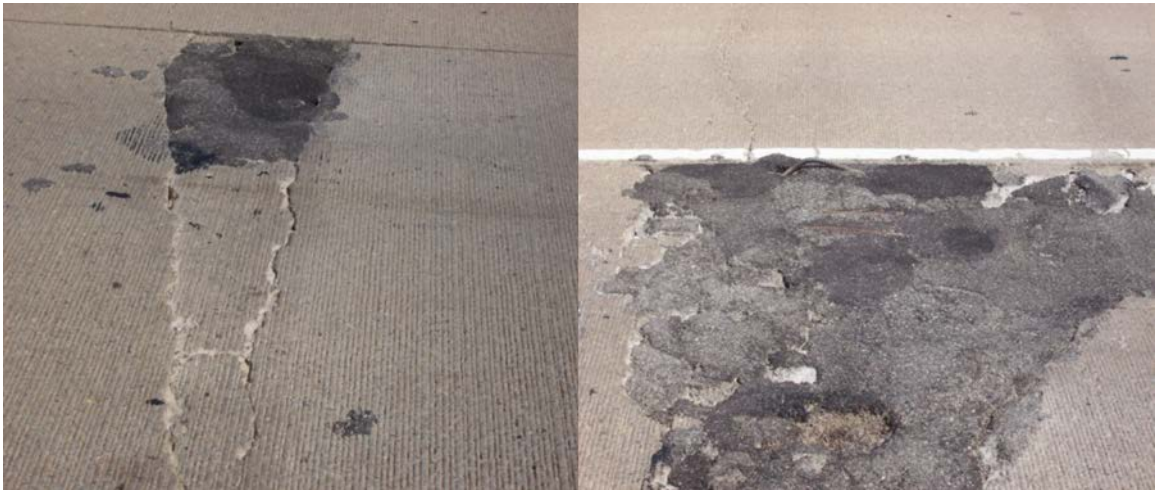
Figure A.43 (left) Patch caused by a Y-crack (right) patch with steel protruding through
