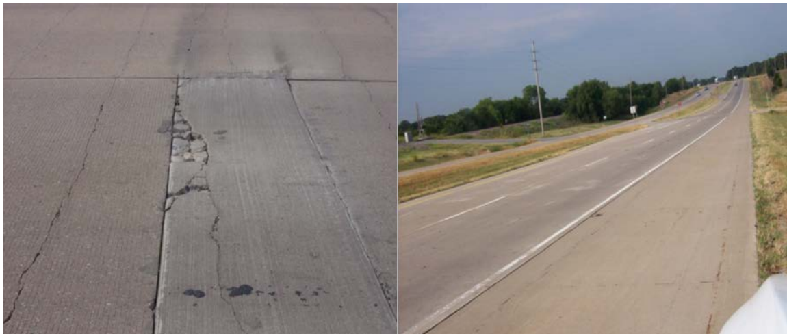
Figure A. 38 (left) patch showing signs of distress (right) area of road where crack survey was taken.
