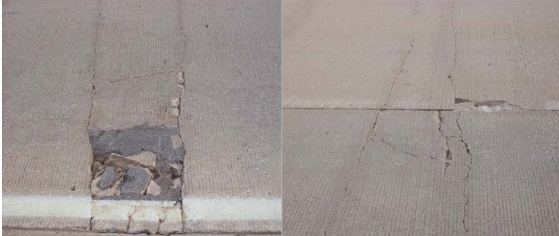
Figure A.25 Punchouts forming between closely spaced transverse cracks
