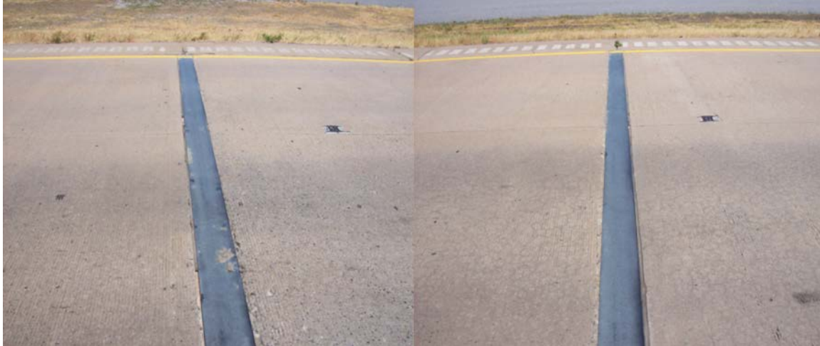
Figure A.40 Spalled terminal joints, with the (right) displaying map-cracking
