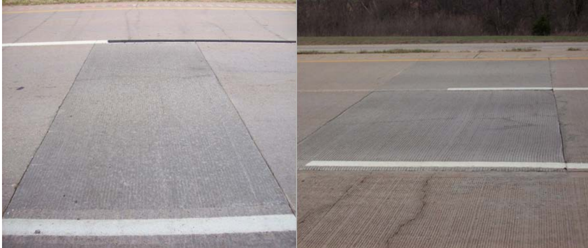
Figure A.74 Patches with longitudinal cracking
