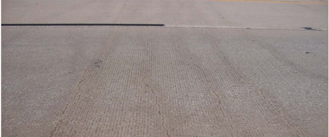
Figure A.23 Closely spaced transverse cracks
