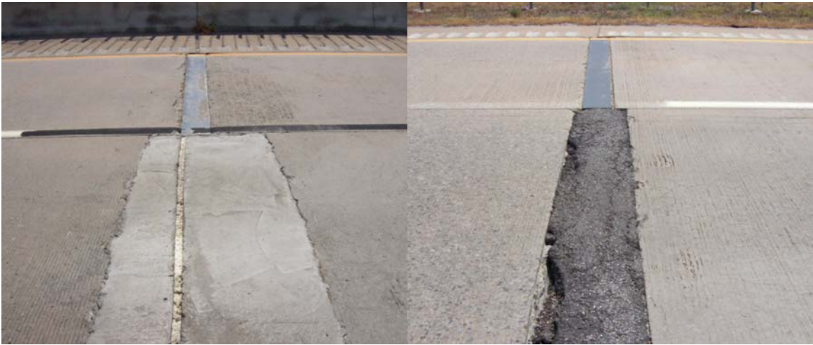
Figure A.59 Terminal joints at the beginning and end of the project
