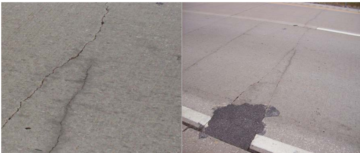
Figure A.72 A transverse crack stopping just short of a “Y” intersection with another transverse crack.
