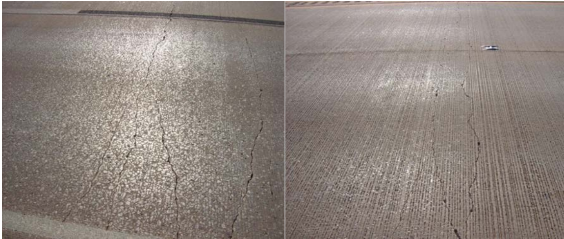
Figure A.3 Photo shows Y-cracks with multiple branches
