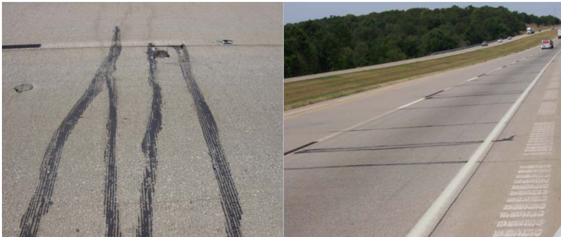
Figure A.29 Transverse cracks sealed with an asphalt joint sealant
