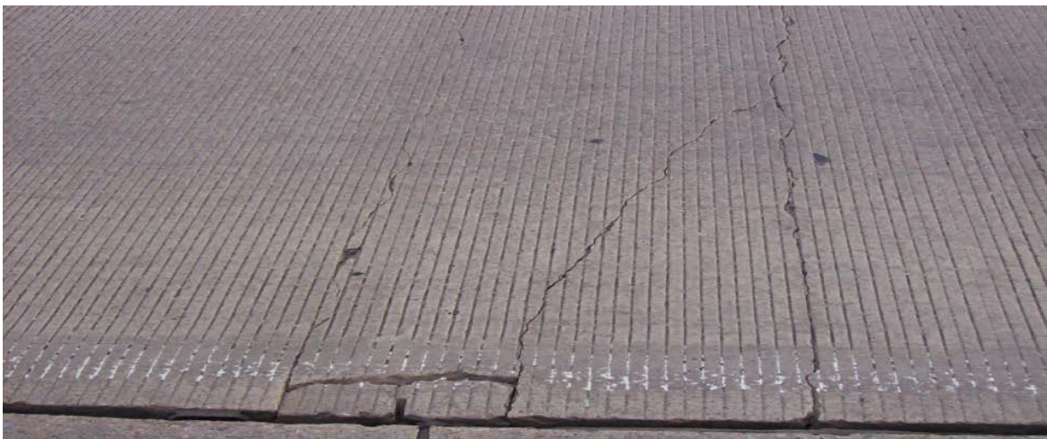
Figure A.35 Typical Y-crack for the area
