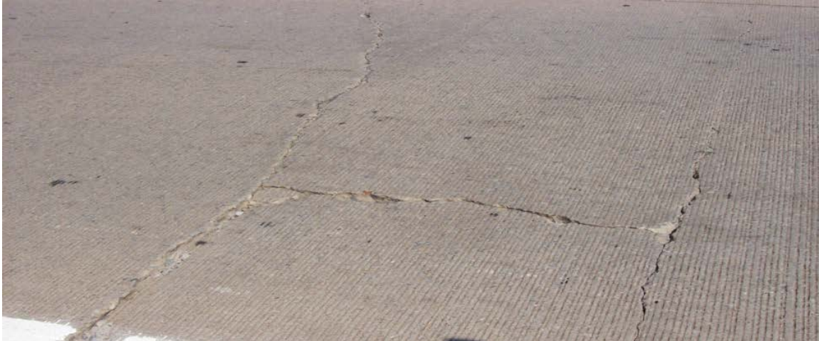
Figure A.44 Two transverse cracks intersected by a longitudinal crack
