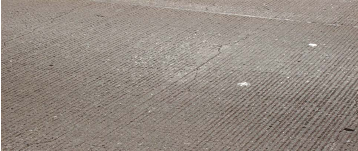
Figure A.2 Photo shows transverse cracks with inter-connecting longitudinal cracks.
