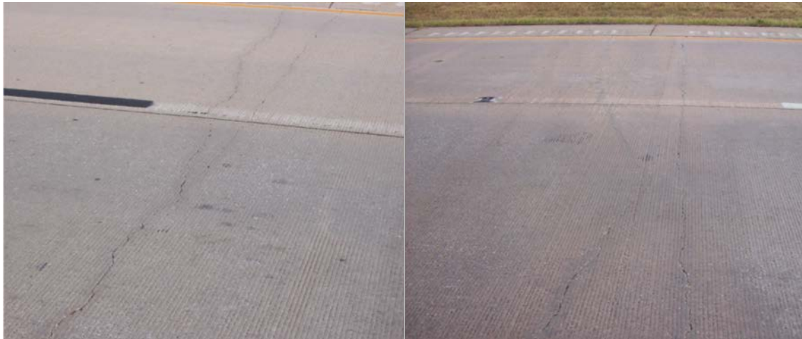
Figure A.22 Two different types of Y-cracks found in the area
