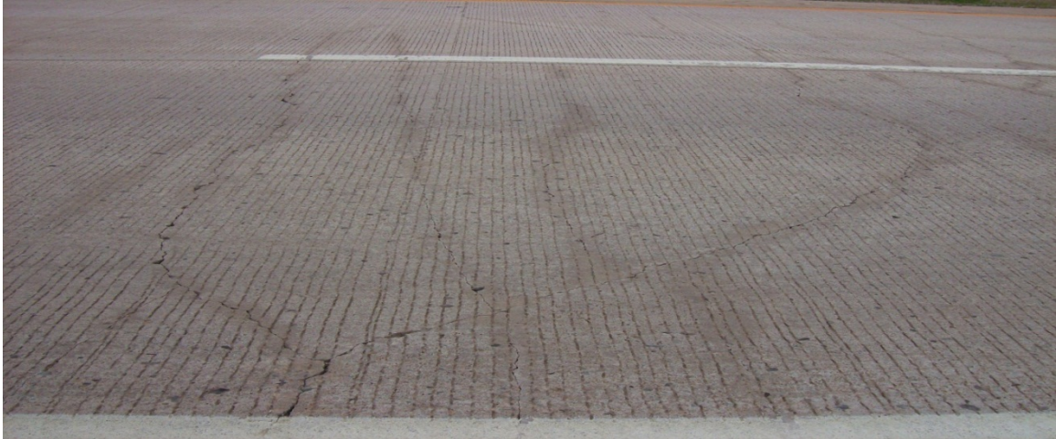
Figure A.91 A circular crack intersecting multiple transverse cracks
