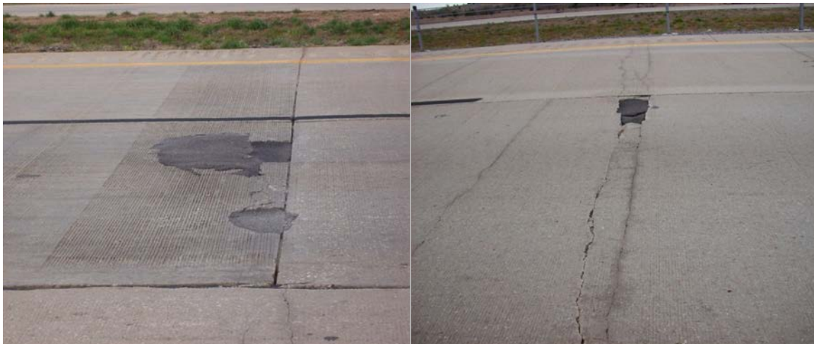
Figure A.75 Patches forming between closely spaced transverse cracks and at construction joints
