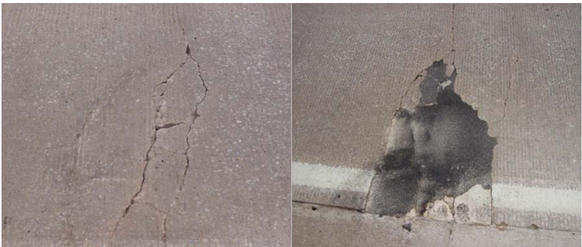
Figure A.24 Two instances where a Y-crack seemed to be developing into a punch-out
