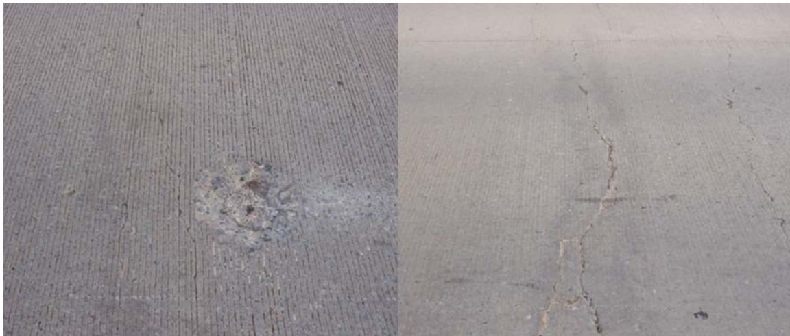
Figure A.53 (Left) Large circular distress, (right) Spalled Y-crack beginning to break up
