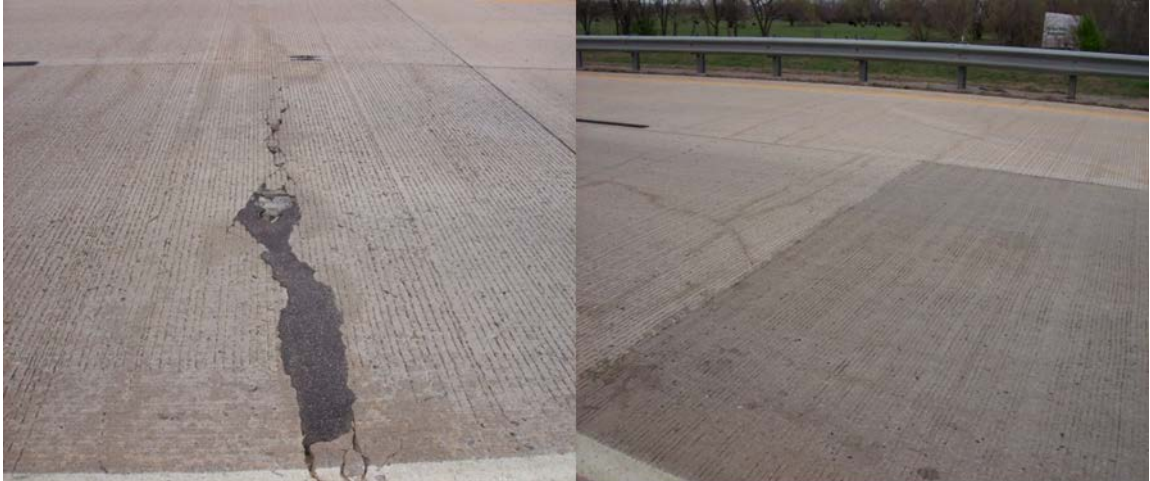
Figure A.89 Patches occurring next to construction joints
