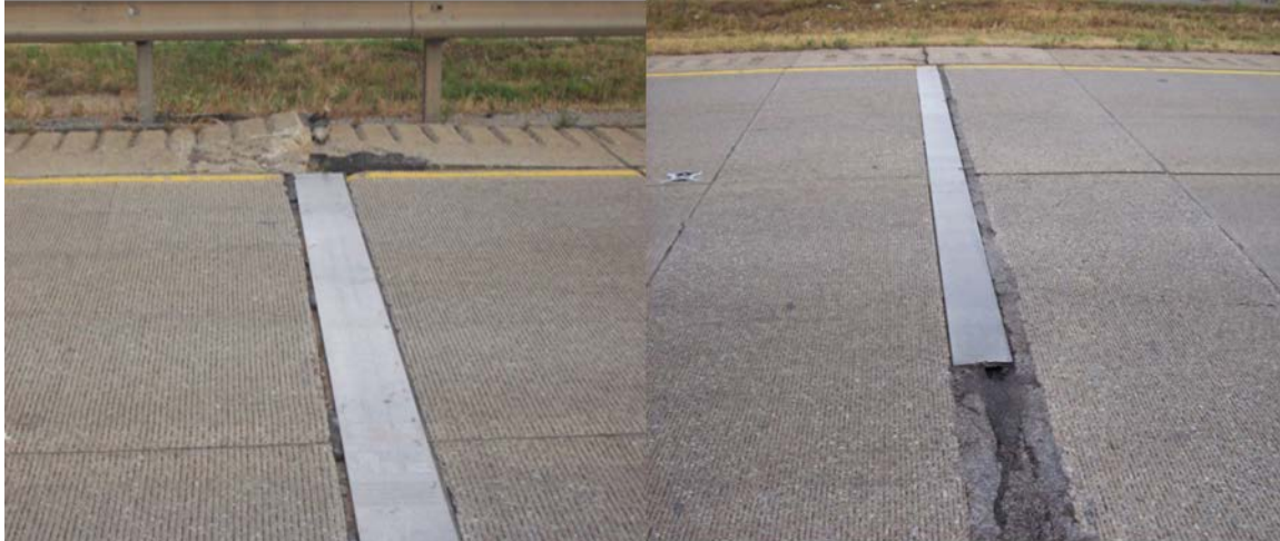
Figure A.34 Terminal Joints with different kinds of distress
