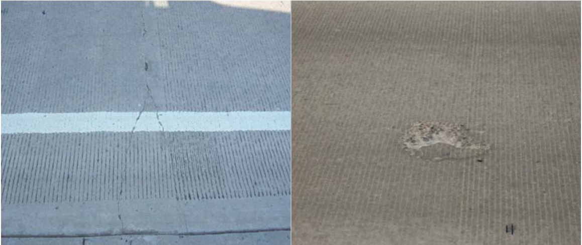
Figure A.15 (Left) Typical Y-crack for the region, (right) circular spalled area
