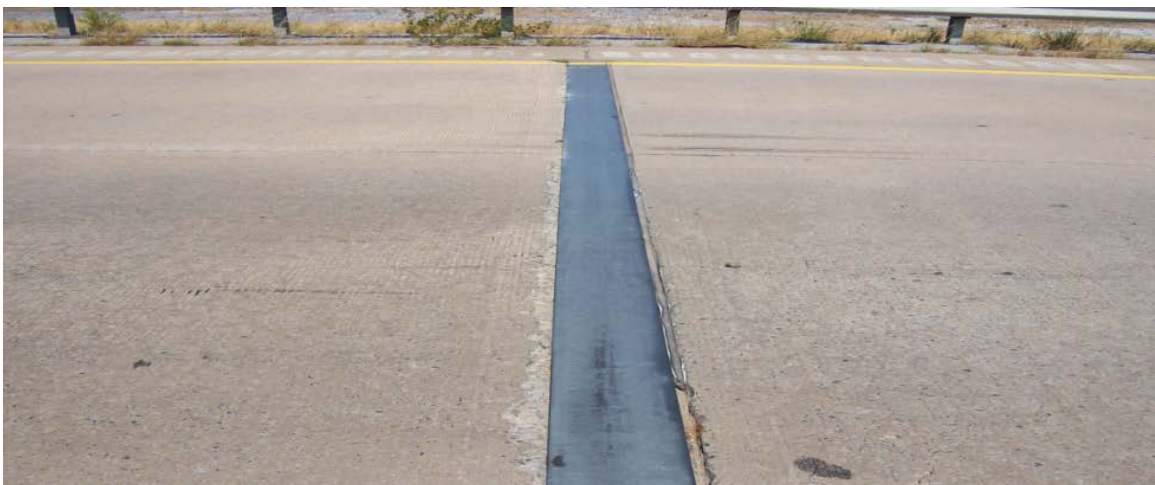
Figure A.39 Spalled terminal joint with worn roadway surface
