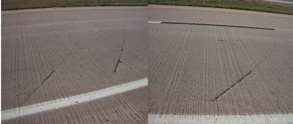
Figure A.93 Exposed steel on the surface of the pavement
