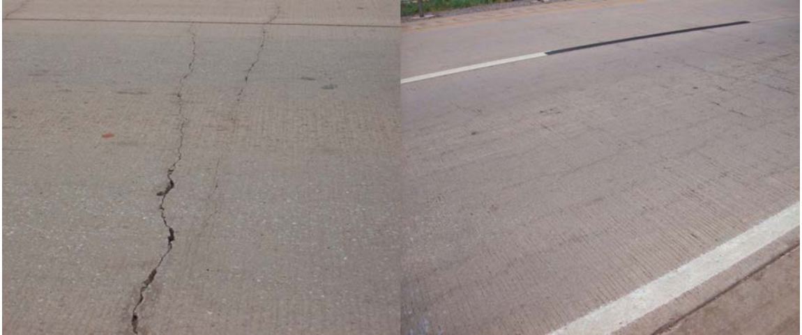
Figure A.87 (Left) two transverse cracks nearly connecting (right) longitudinal cracking
