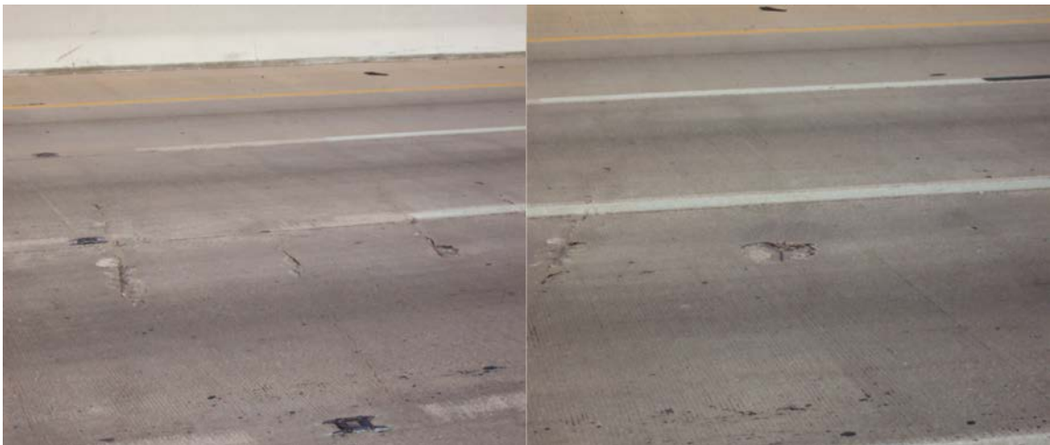
Figure A.9 More distresses in ODOT's region of concern
