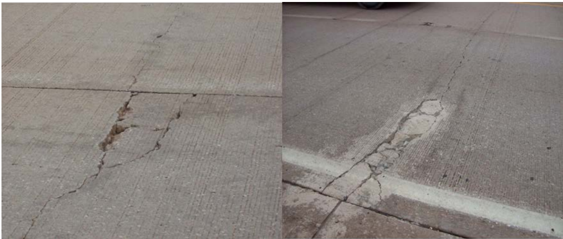
Figure A.77 Punchouts/ patches forming near Y-cracks
