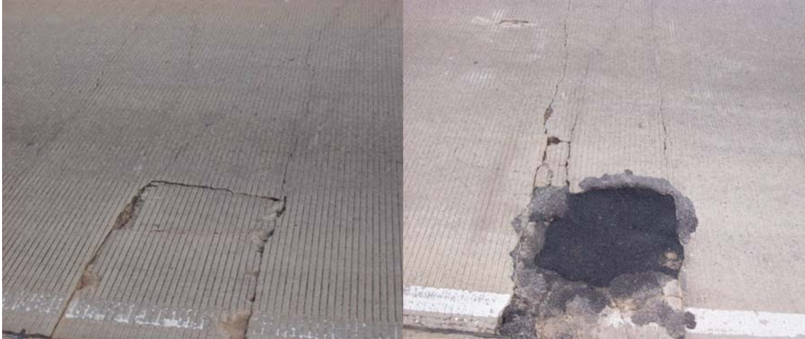
Figure A.36 Y-cracks leading to punch-out and eventually failure
