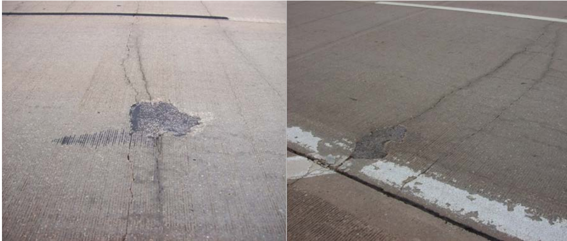
Figure A.71 Meandering cracks with small patches stopping just short of a “Y” intersection
