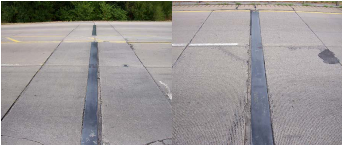
Figure A.33 Terminal joints showing signs of spalling
