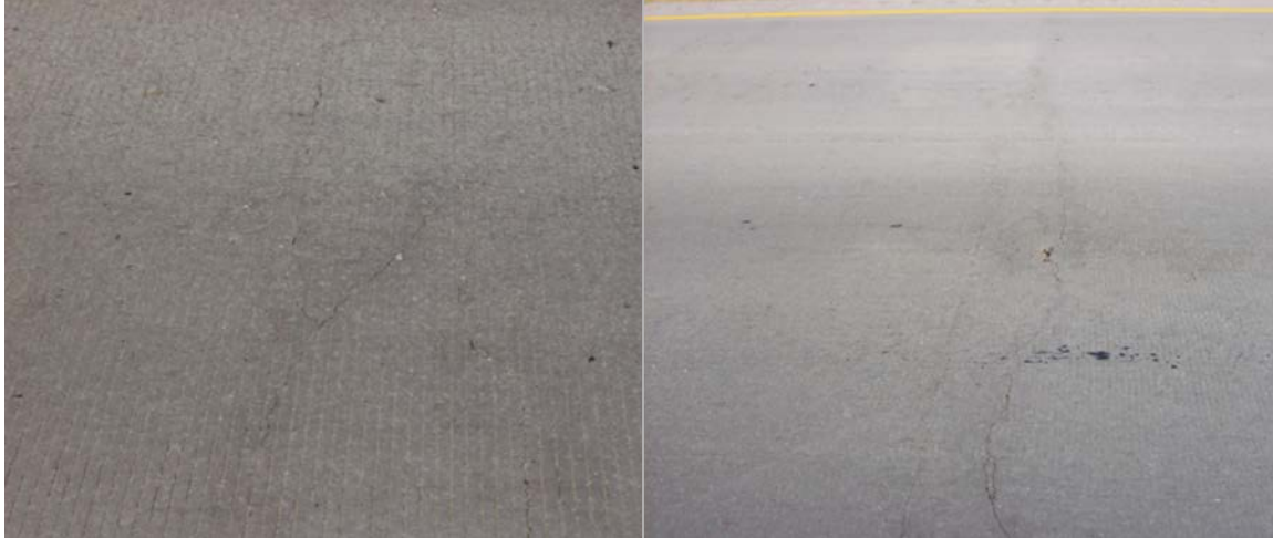
Figure A.17 (Left) Y-crack located in the region; (right) two close transverse cracks showing distress
