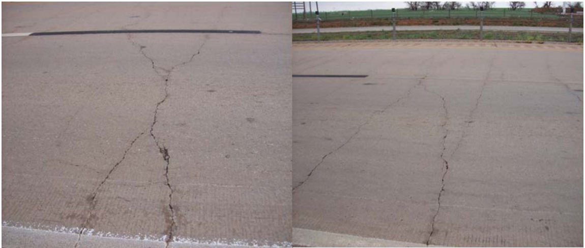
Figure A.85 Typical Y-cracks observed in the inspection
