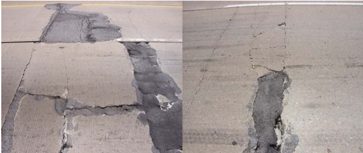
Figure A.46 Transverse cracks intersected by longitudinal cracks
