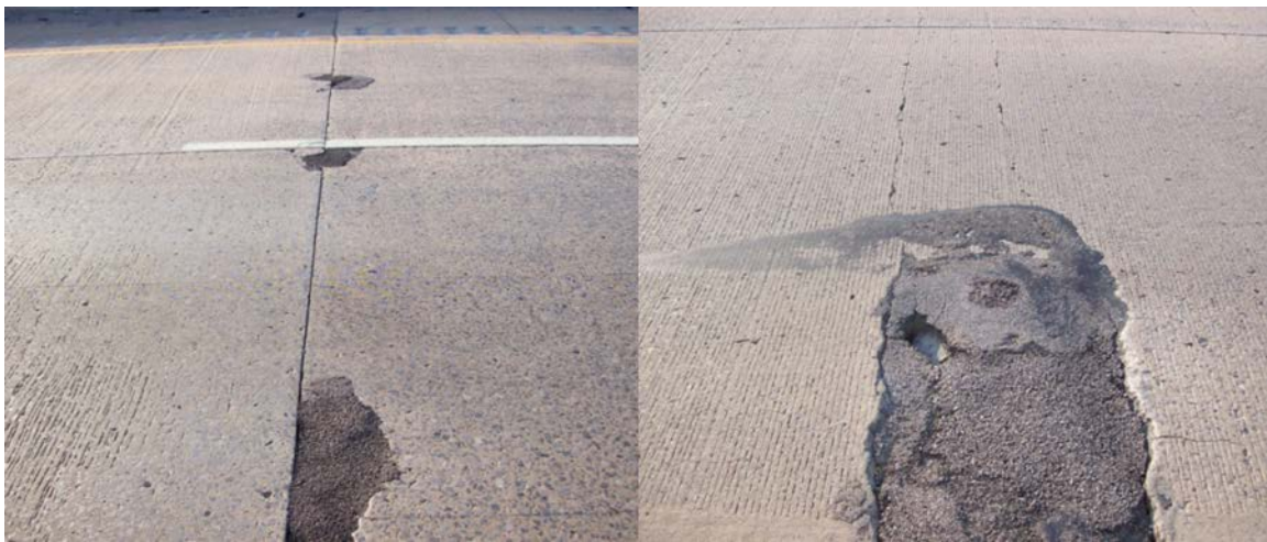
Figure A.68 Patches in the southbound lane
