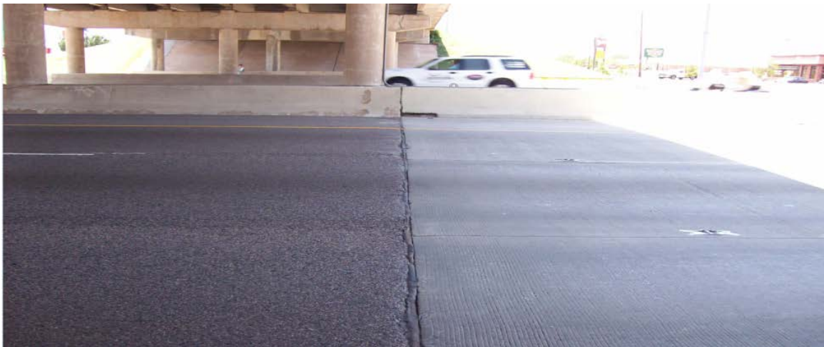
Figure A.13 Joint at the Southern end of North bound lane
