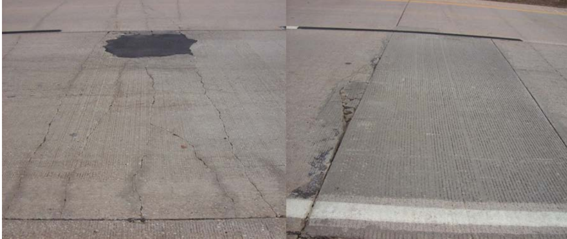
Figure A.79 (Left) Patch at construction joint, (Right) closely spaced transverse cracks with a patch
