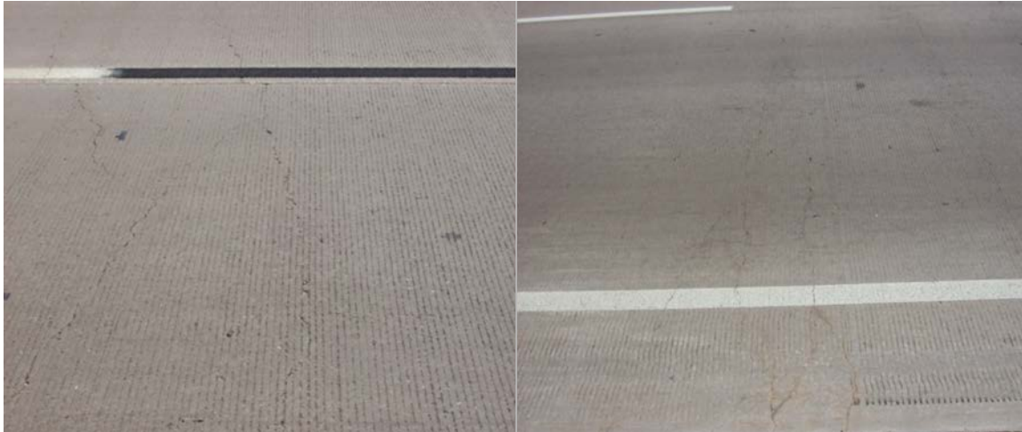
Figure A.19 Two different forms of Y-cracking
