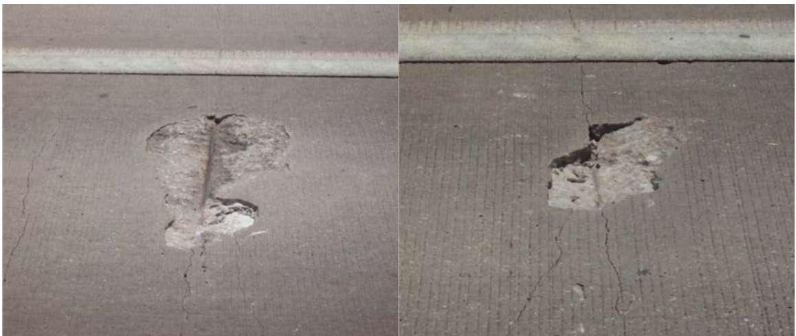
Figure A.11 Possible Y-crack over shallow transverse steel
