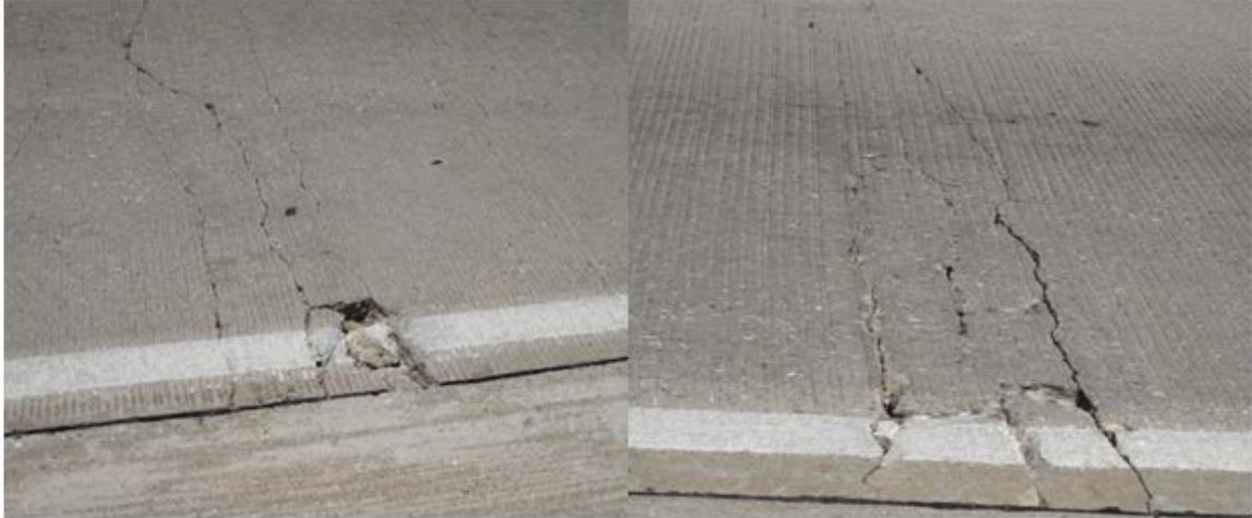
Figure A.5 Developing punch-out between two close transverse cracks
