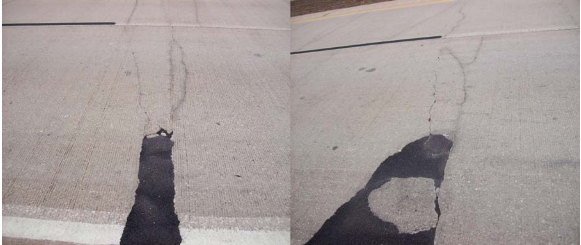
Figure A.76 Punchouts/ patches forming near Y-cracks
