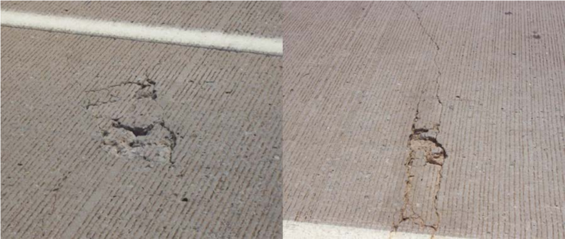
A.60 (left) Two closely spaced transverse cracks, (right) Y-crack developing into a punch-out
