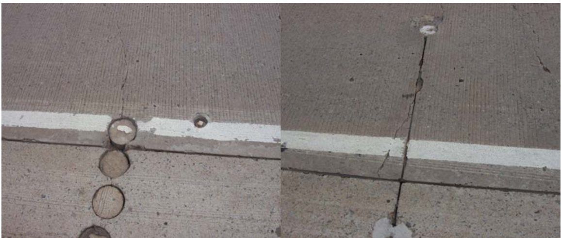
Figure A.58 (left) cores taken from shoulder, (right) core with sensor wire extending to shoulder
