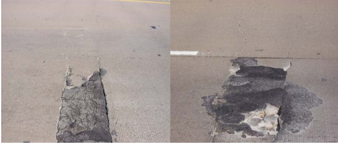
Figure A.42 More patches cause by closely spaced transverse cracks
