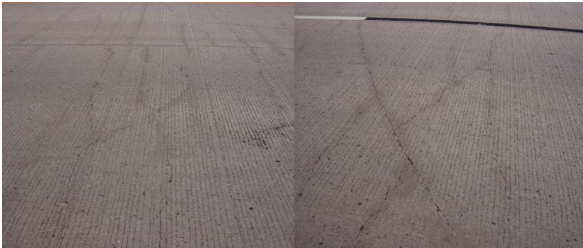
Figure A.92 Typical Y-cracks seen in the East bound direction
