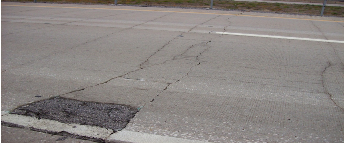
Figure A.78 Punchouts/ patch forming near Y-cracks
