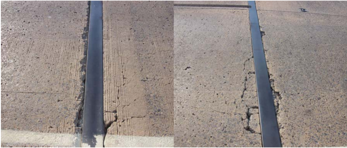
Figure A.69 Terminal joints at the beginning and end of the project
