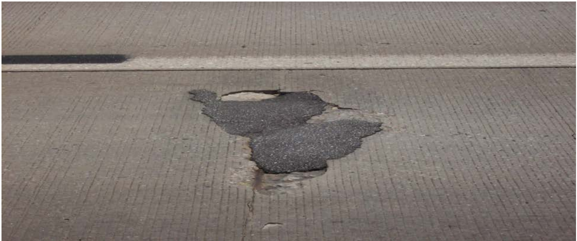
Figure A.10 AC patch over a distress with exposed transverse steel
