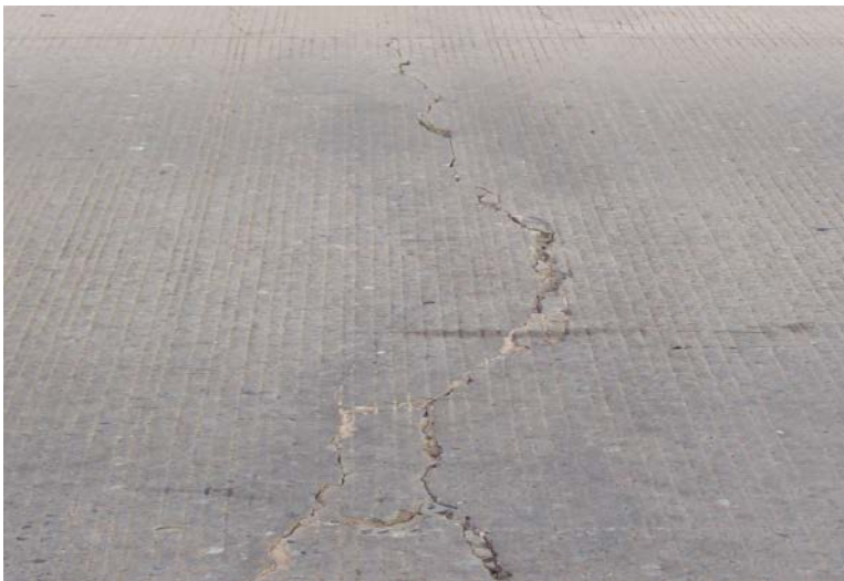
Figure 2.3 Example of spalling
