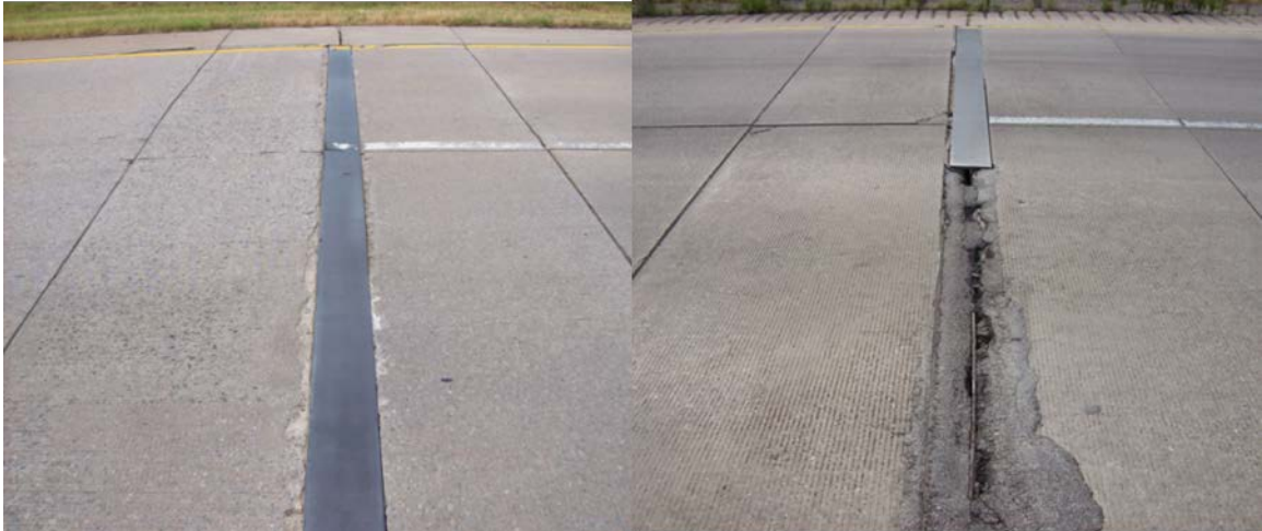
Figure A.37 Terminal joints showing distress
