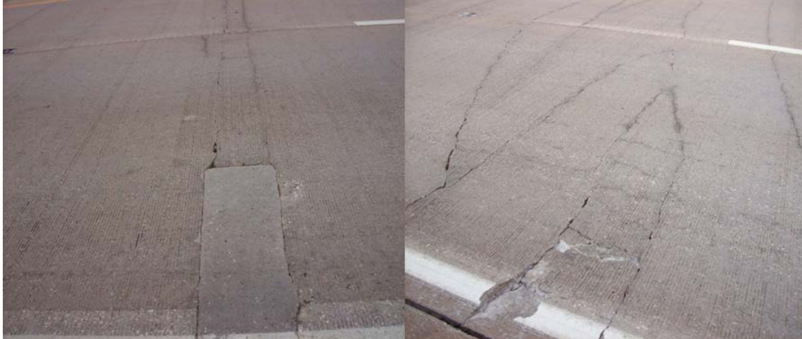
Figure A.73 Punchouts forming between closely spaced transverse cracks
