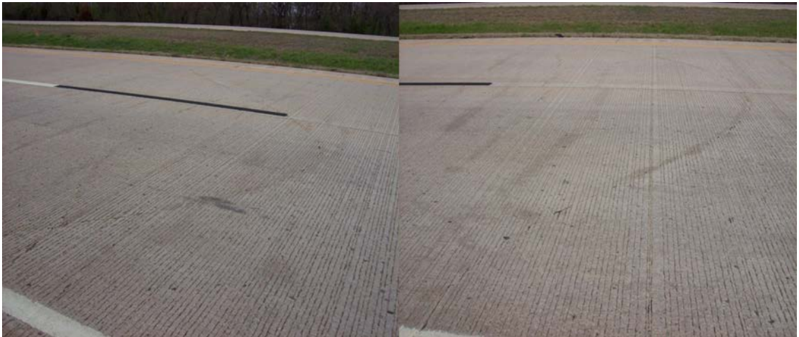
Figure A.90 Circular cracks intersecting transverse cracks
