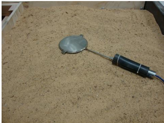
Figure 66. An earth pressure cell is placed on a 1 inch sand layer on the top of the aggregate
