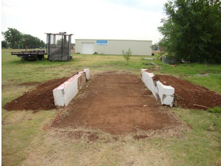
Figure 140. Concrete beams placed on both sides of the test section with soil support on the outside
