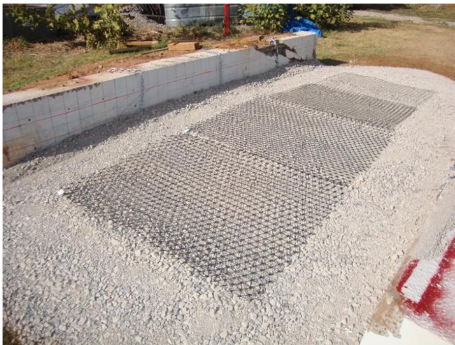
Figure 147. Four extruded geogrids are placed on the first layer of compacted aggregate
