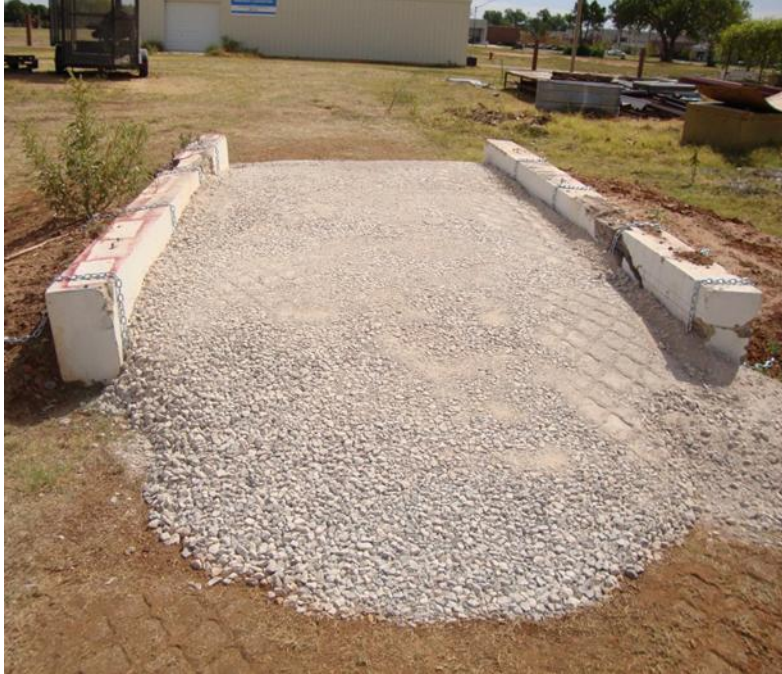
Figure 150. The top (second) layer of aggregate in the test bed after compaction
