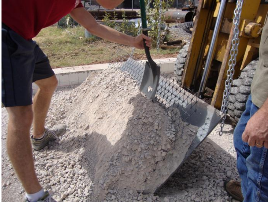
Figure 153. Tilting of steel plates and removing of aggregates to facilitate exhumation process
