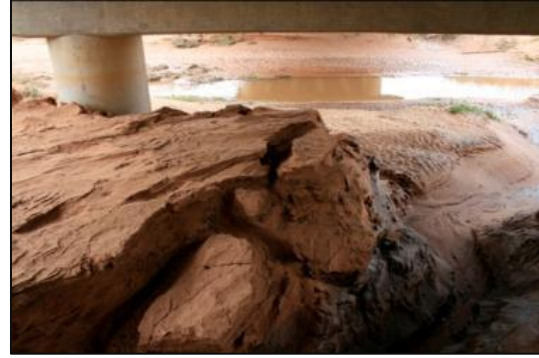
Figure 4.12 Erosion channel at S.H. 152 over Lake Creek continues
