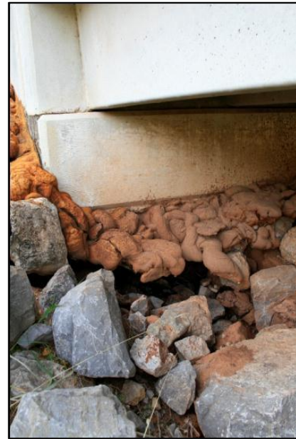
Figure 4.14 Void and maintenance under abutment at S.H. 9 over Running Creek
