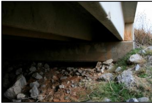
(c) Red staining on abutment at S.H. 152 over Lake Creek Overflow, photographed November 11 th , 2011
