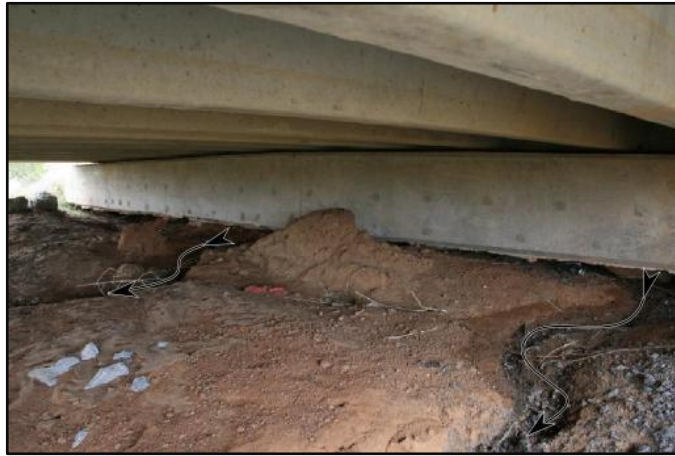
Figure 4.15 Erosion flow beneath abutment at S.H. 152 over Lake Creek Overflow
