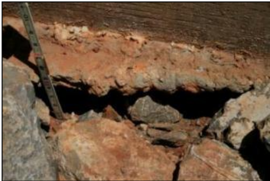
Figure 4.20 4" void beneath the abutment
