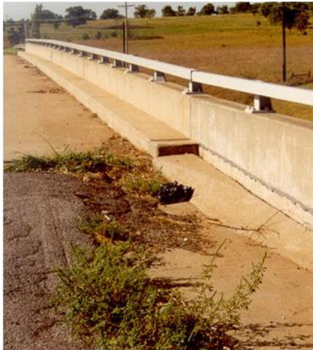
Figure 1.1 Displacement at Bridge Approach Slab-Bridge Interface due to Differential Settlement
