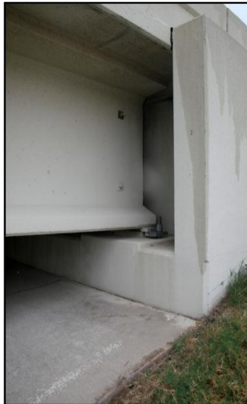
(b) Blue lines on the wing-wall indicate the original soil level and the settlement of the embankment relative to the structure at 19 th St. over I-35
