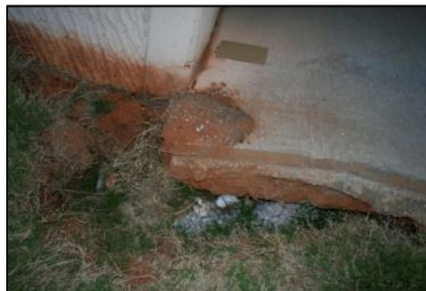
Figure 4.33 Void forming beneath slope wall and abutment
