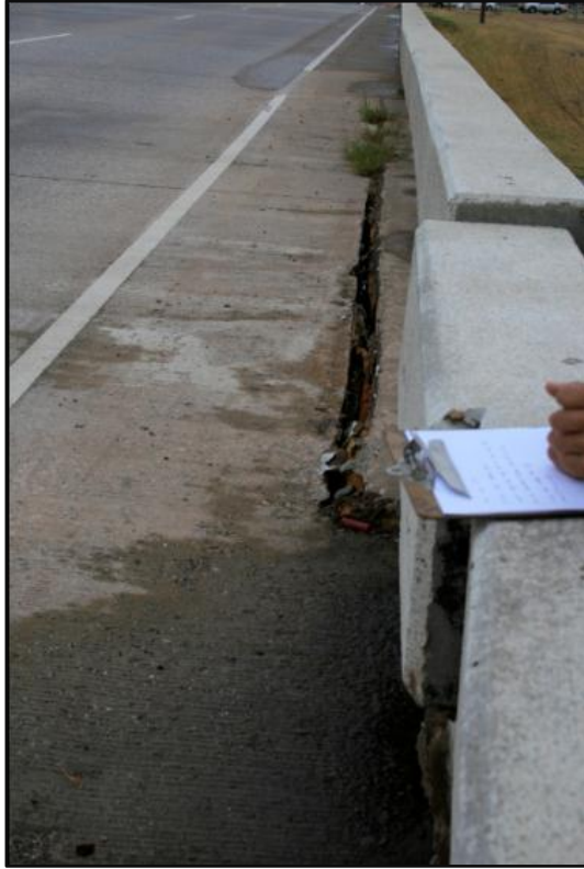
(a) Horizontal separation between wing wall and approach slab
