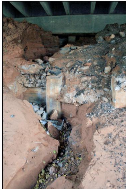
Figure 4.13 Erosion channel from beneath abutment at S.H. 152 over Willow Creek
