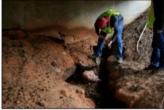
Figure 4.11 Erosion channel under abutment at S.H. 152 over Lake Creek
