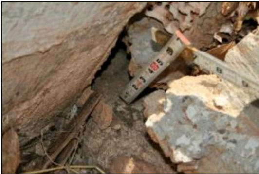
Figure 4.21 4" void beneath the approach slab
