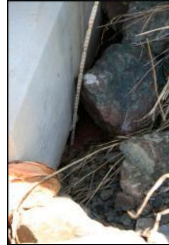
Figure 4.17 Void forming beneath abutment at S.H. 3W over Big Creek
