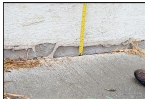
(d) 2" of embankment settlement is measured between the embankment and wing-wall at I-35 over Main St.
