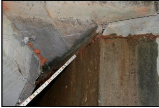
(a) Water and soil flowing through a cracked abutment on S.H. 59 B over Coon Creek, photographed May 21 st , 2011
