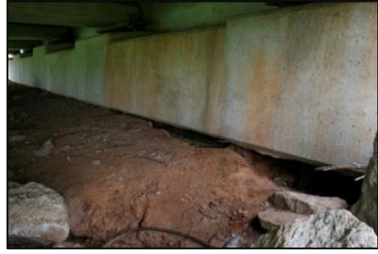
(b) Red stains on the abutment indicate the possibility of soil loss through U.S. 177 over the Salt Fork, photographed June 2 nd , 2011
