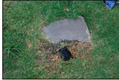
(c) The outlet at I-35 over Main St. is almost completely buried
