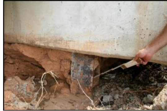
Figure 4.9 A 1' 9" void under abutment
