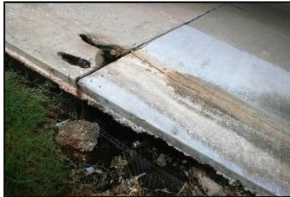
Figure 4.34 Water flowing from outlets into embankment, Tecumseh Rd. over I-35. (note large void under slope wall)
