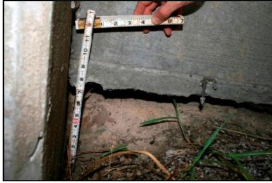
Figure 4.8 A 7" void under approach slab
