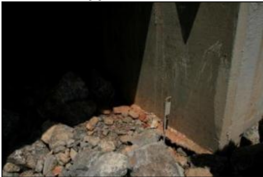
4.22 Void beneath north abutment
