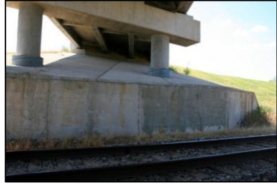
(d) Red stains originating from crack at S.H. 1 over BNSF, photographed August 26 th , 2011
