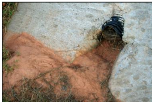
Figure 4.32 Soil flowing from underdrain outlet
