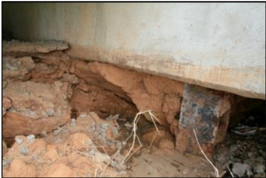
Figure 4.28 Erosion beneath abutment at U.S. 177 over Salt Fork, Embankment B-2
