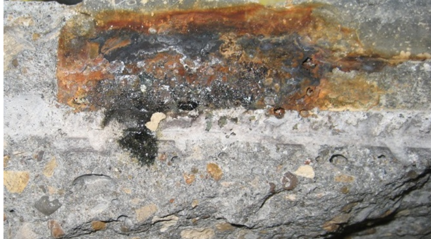
Figure 93b: Staining on inside of cracked beam specimen 1 containing 2304 stainless steel
