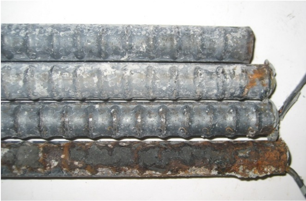
Figure 101b: Bottom bars from Southern Exposure specimen 3 containing stainless steel clad reinforcement as the anode and conventional steel as the cathode after autopsy
