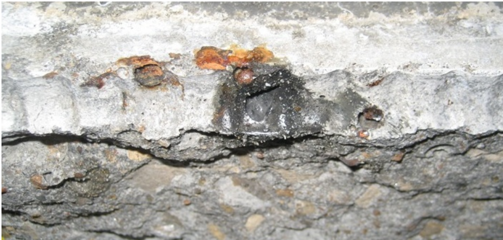
Figure 91: Staining on inside of Southern Exposure specimen 3 containing epoxy-coated reinforcement with penetrations in the epoxy.
