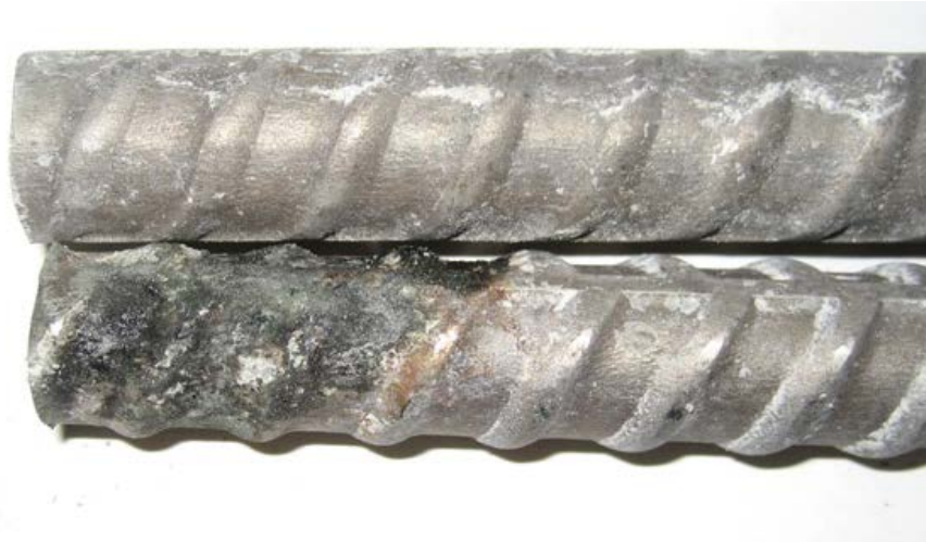
Figure 70: Corrosion product on 2304 stainless steel anode bar in 2304/Conv. Southern Exposure specimen 2 after autopsy
