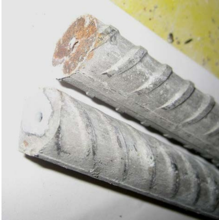
Figure 101c: Top bars from Southern Exposure specimen 2 containing stainless steel clad reinforcement as the anode and conventional steel as the cathode after autopsy, showing corrosion of at ends of top bars (close up)
