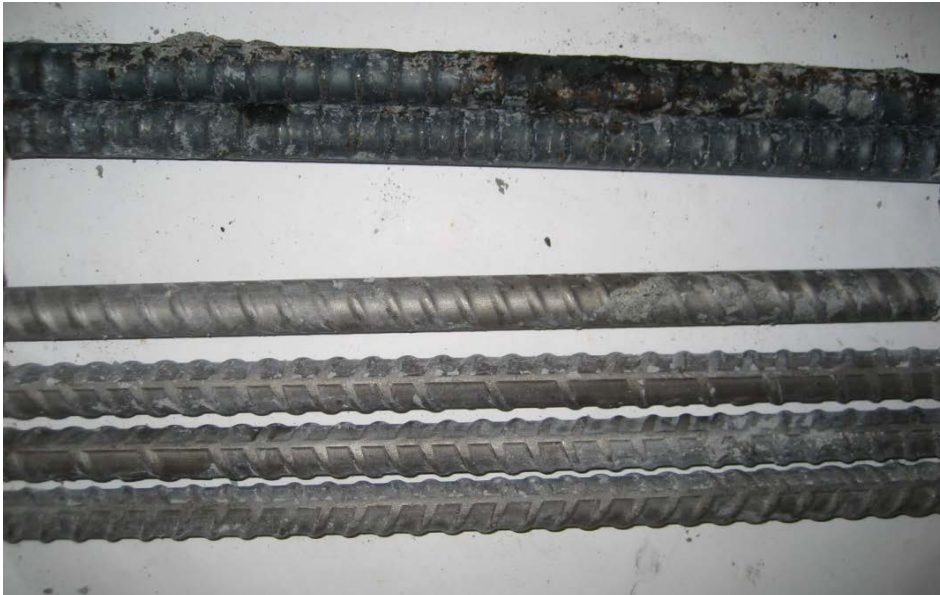
Figure 88b: Bars from Southern Exposure specimen 3 containing conventional reinforcement as the anode and 2304 stainless steel as the cathode after autopsy
