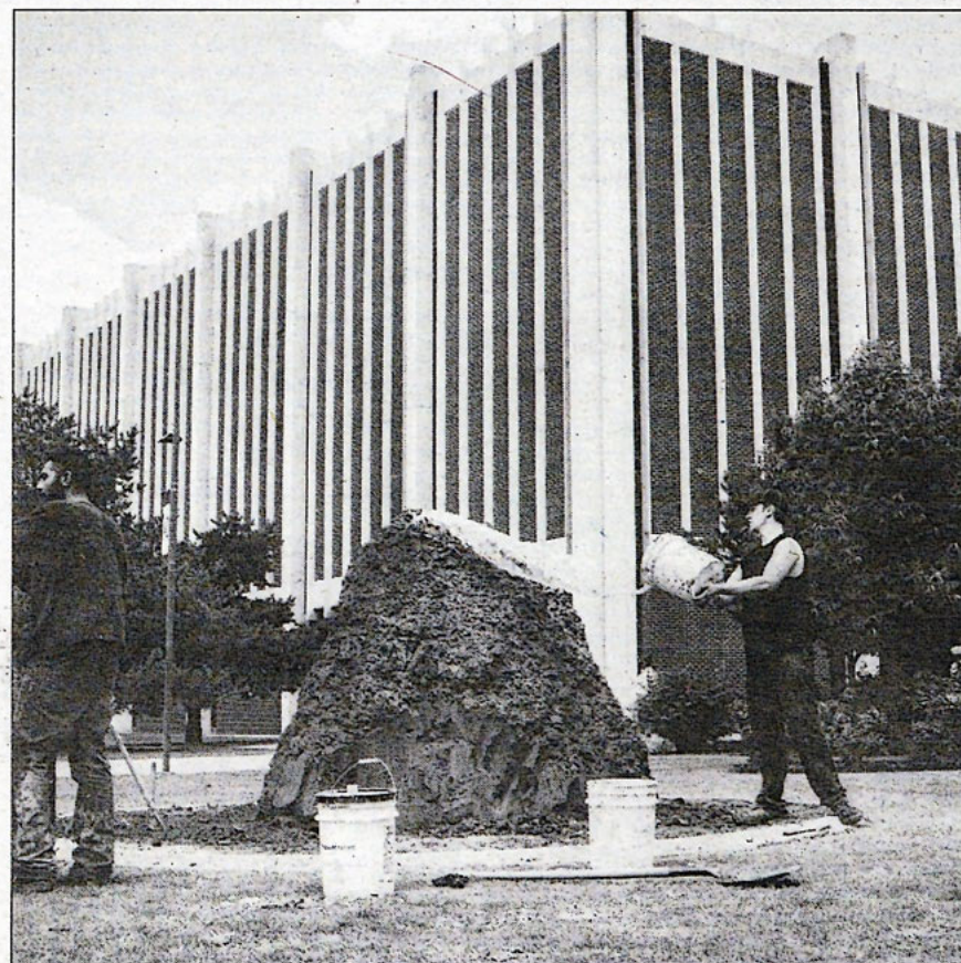
Professional contractors Slade Tosh and Marcus Jernigan construct the new BRock on Thursday, June 8. The two contractors finished the rock over the course of two days. Photo by Ryan Naeve, The Vista.
