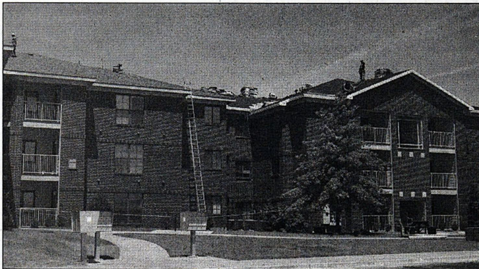
The UCO Commons' roofs under construction during the summer. Photos by Quang Pho, The Vista.
