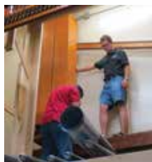
John Riester during the installation of the Kilgen at the Oklahoma History Center.
