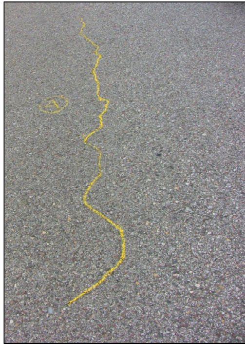
(b) Longitudinal cracks from 24 ft. to 32 ft.
